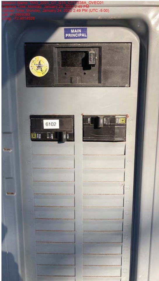
Existing Electrical Service Used For Upgrade
