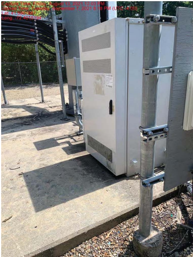
Existing T-Mobile Equipment Mounted To Concrete Pad
