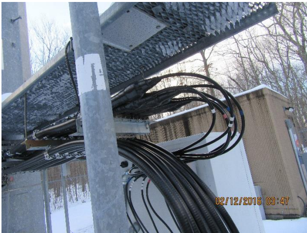
Six lengths of new coaxial cable and six lengths of existing coaxial cable on ice bridge
