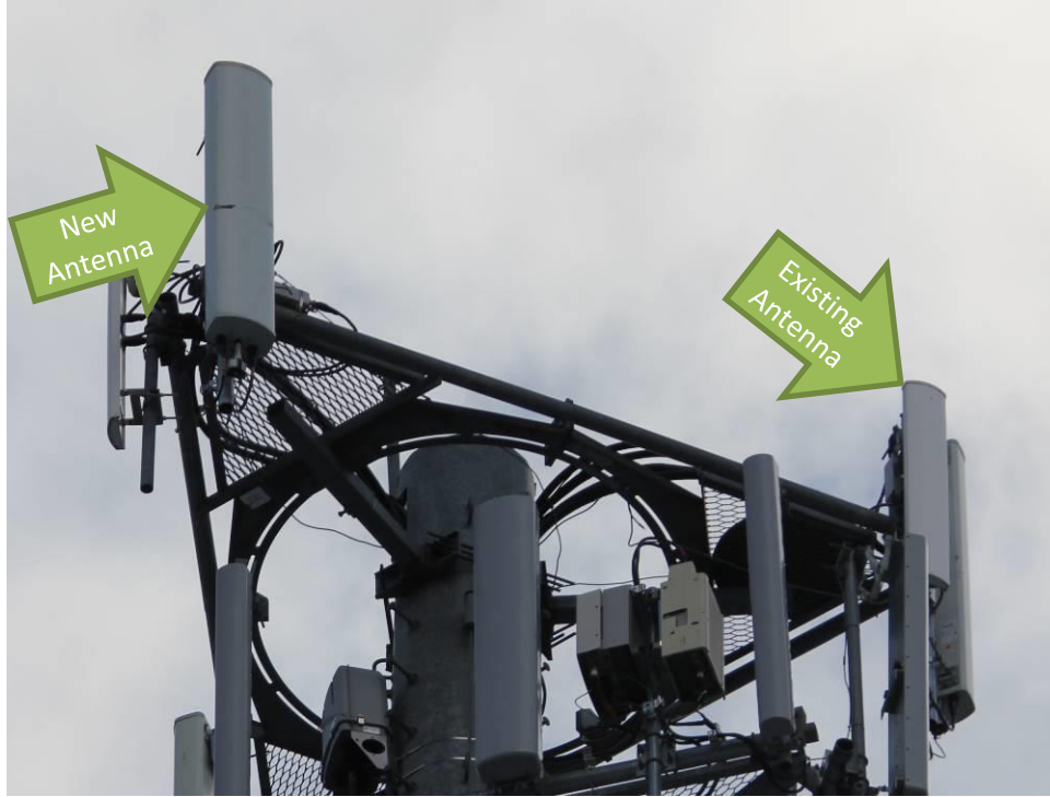
Typical sector showing new and old panel antennas
