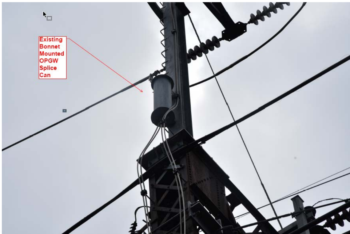
Typical Bonnet Mounted OPGW & Splice Can L753 – August 5, 2019 Inspection
