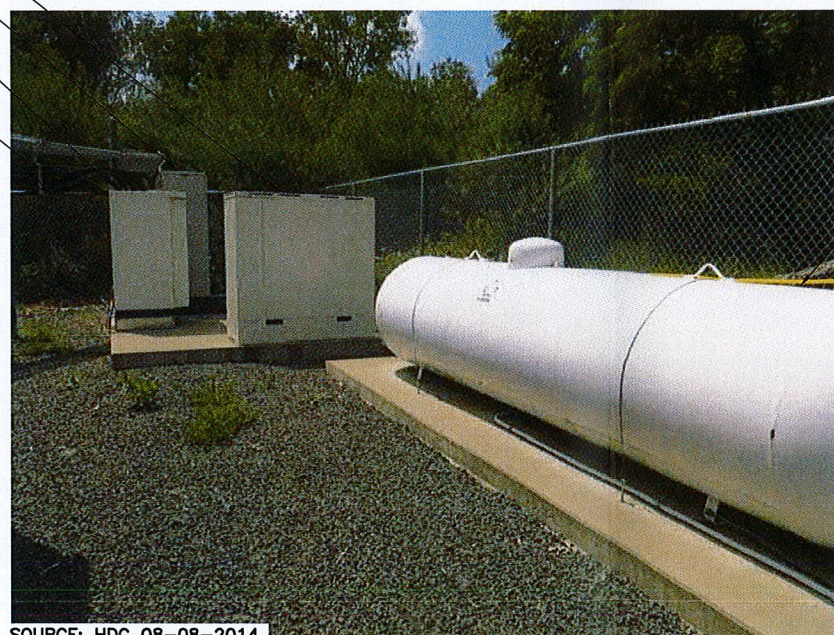
EXISTING PROPANE TANK
