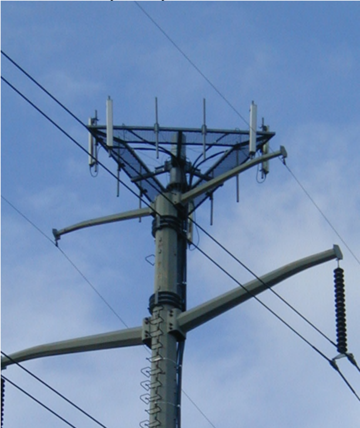
Close-up of antenna platform and mount extension
