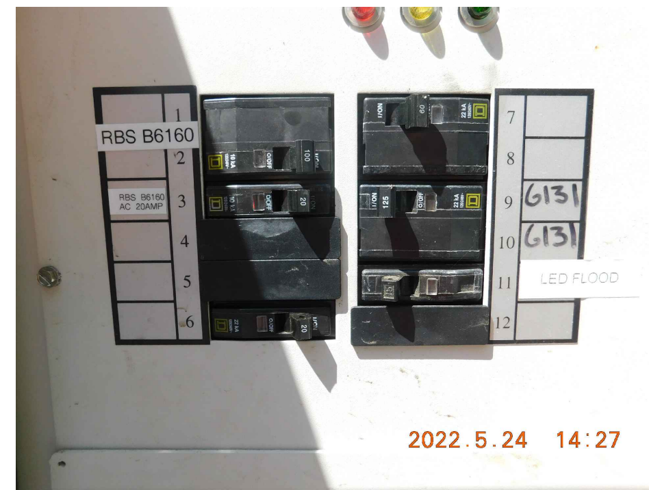
EXISTING POWER PANEL PHOTO
