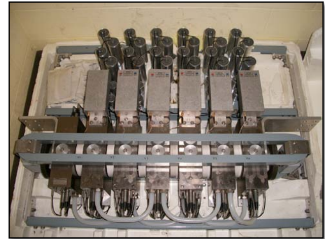
Note: Valve Module
