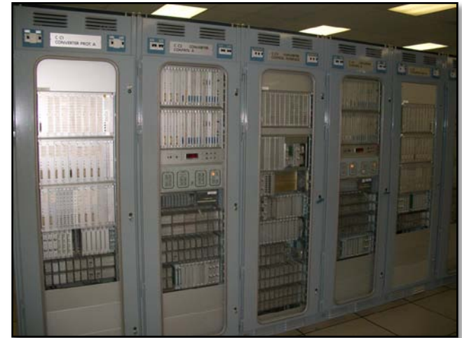
Note: HVDC Control System where internal Faults generally lead to failed equipment and permanent failures
