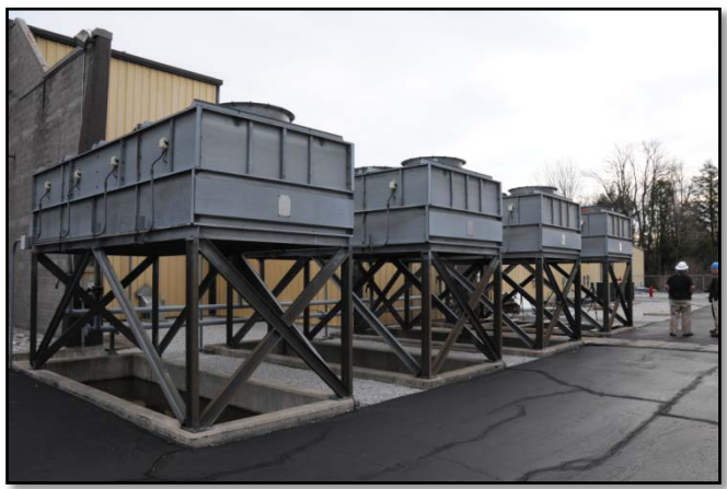
Note: Raw water heat exchangers
