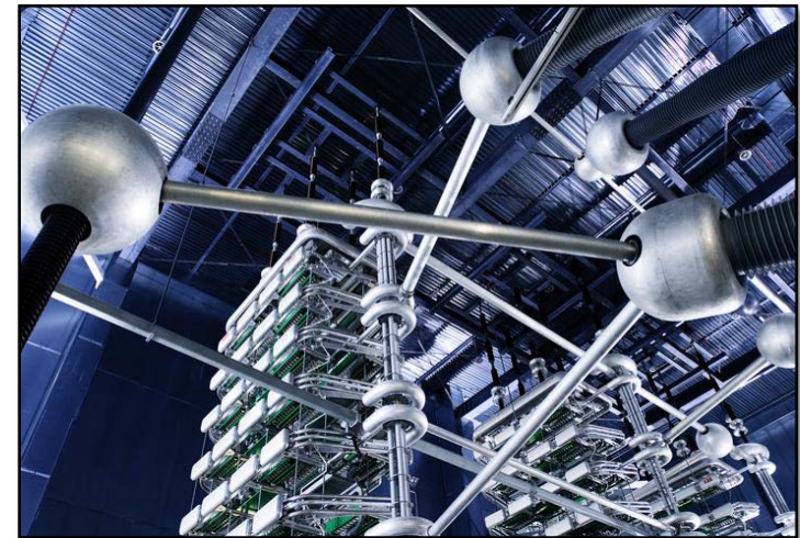
Note: Valve Hall Testing Facility
