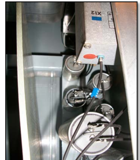
Note: Leaking capacitor in a valve module (center of the picture)
