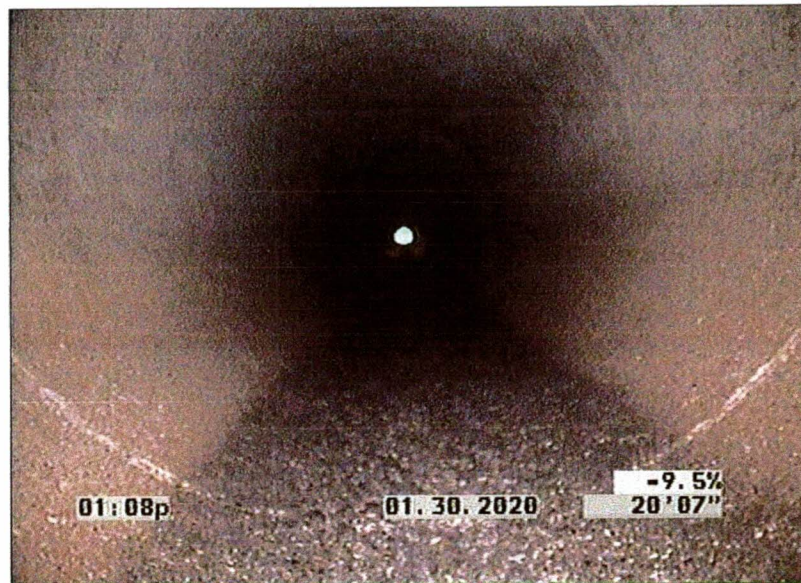
Photo: 1_1_2_30012020_121406_A.JPG, 00:02:17 service connection, at 12 o'clock / 20' Out Fr Cb 1 Dp 6' 7"
