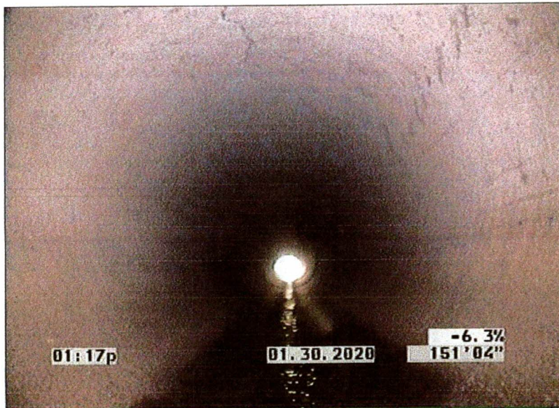
Photo: 1_1_8_30012020_122329_A.JPG, 00:06:48 service connection, at 12 o'clock / 150' Out Fr Cb 1 Dp 6' 5"
