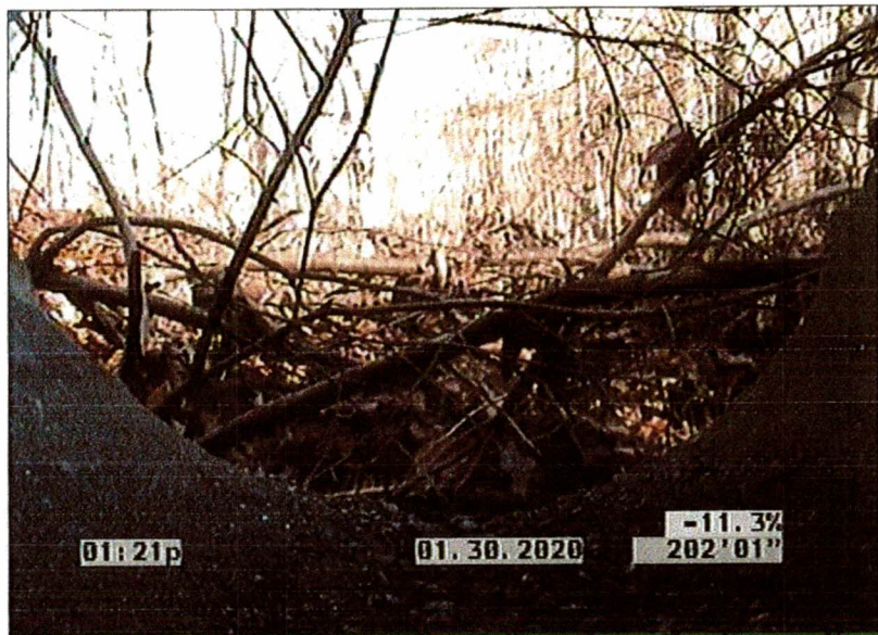
Photo: 1_1_10_30012020_122704_A.JPG, 00:08:24 inspection ends at downstream manhole / 200' Out Fr Cb 1 End Of Inspection Culvert
