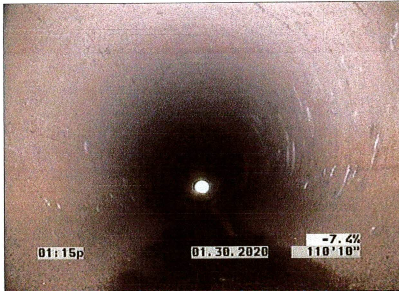
Photo: 1_1_6_30012020_122038_A.JPG, 00:05:25 service connection, at 12 o'clock / 110' Out Fr Cb 1 Dp 7' 9"
