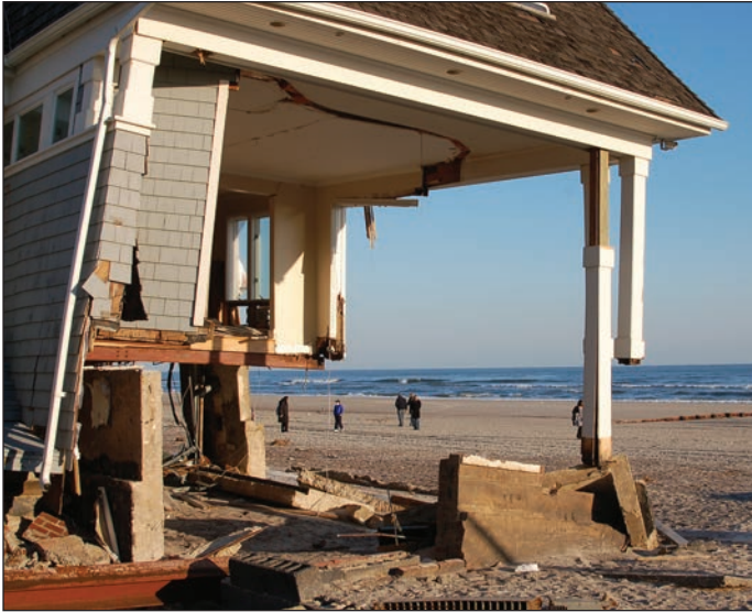
Figure 6: Wave, storm surge, and erosion damage to oceanfront house at Rockaway, NY
