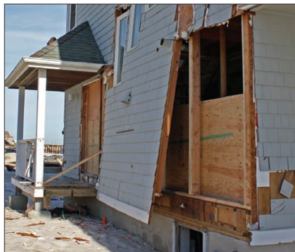
Figure 1: Back wall failure due to flood level above the lowest floor of a house in Ortle Beach, NJ
