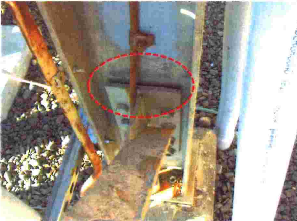
Figure 7: Box Structure Bracing Gap#2 indicates movement (Before Temp Repair)
