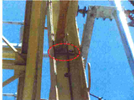
Figure 6: Box Structure Bracing Gap#1 indicates movement (After Temp Repair)
