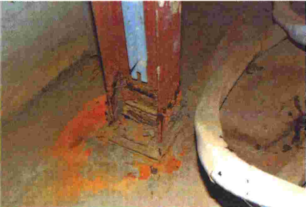
Figure 14: Distribution Control House Deteriorated Supports, Feb 2016
