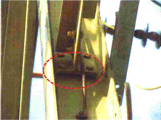
Figure 5: Box Structure Bracing Gap#1 indicates movement (Before Temp Repair)
