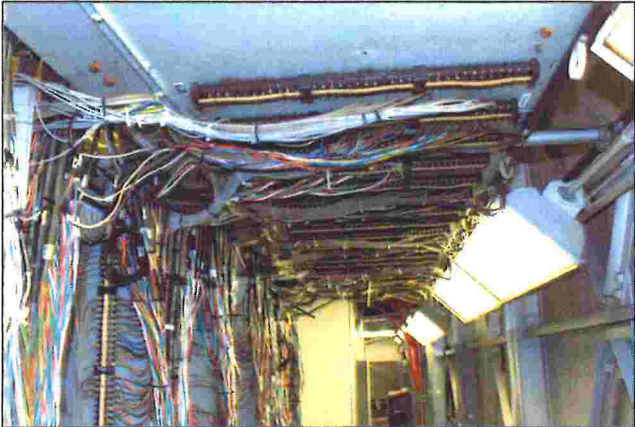
Figure 13: Congested Control Room
