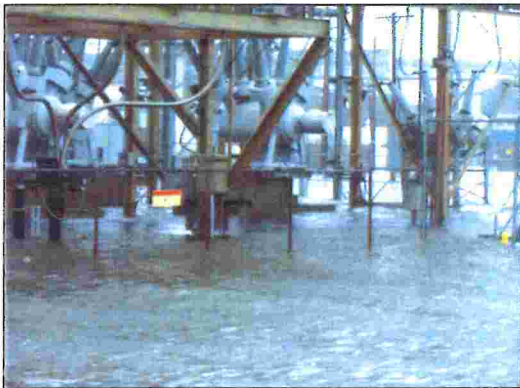
Figure 3: Tropical Storm Irene Flooding (8/28/2011)
