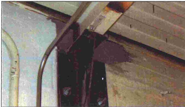
Figure 11: Wall Reinforcements With Mechanical Movement Monitoring Gauge
