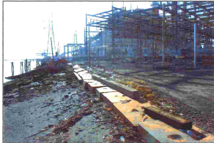
Figure 2: Substation Proximity to Eroding Riverbank
