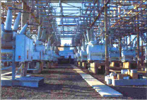
Figure 15: Emergency Mobile Transformer Cannot Fit In Energized Bay
