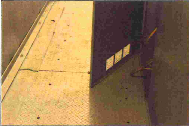
Figure 9: Settling and Cracking Causing Switchgear Door Misalignment
