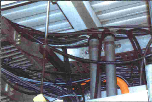
Figure 12: Protection and Control Cable Trays Overloaded
