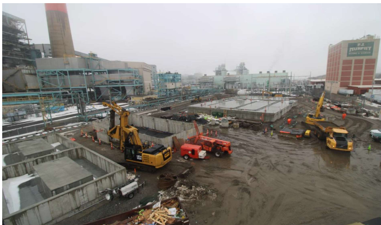
Photo 1: Broadview of project site with TXF and GIS foundation walls being installed.
