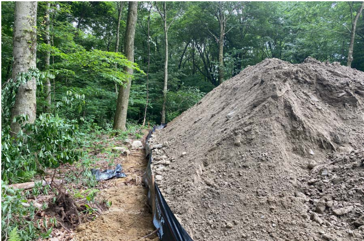
Photo 6: View of erosion controls in good condition looking south along eastern side of compound at foundation excavation spoil pile.
