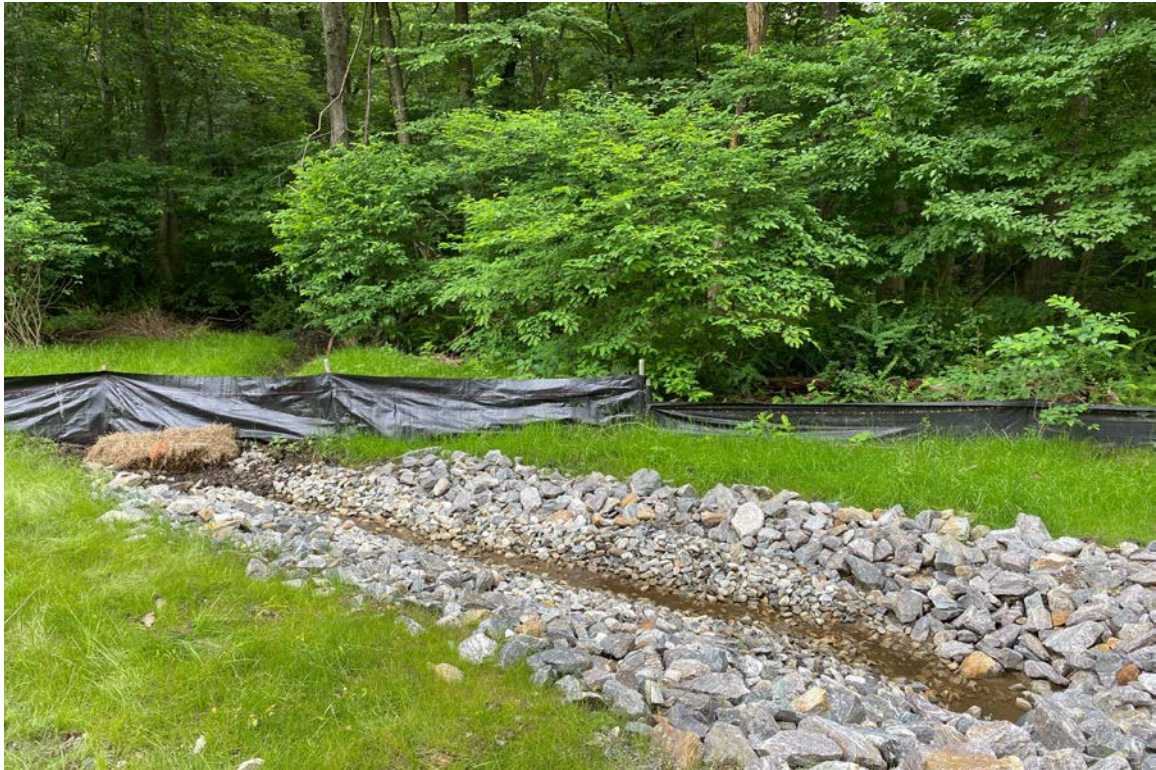
Photo 7: View of erosion controls along culvert crossing looking east; all controls found in good condition.
