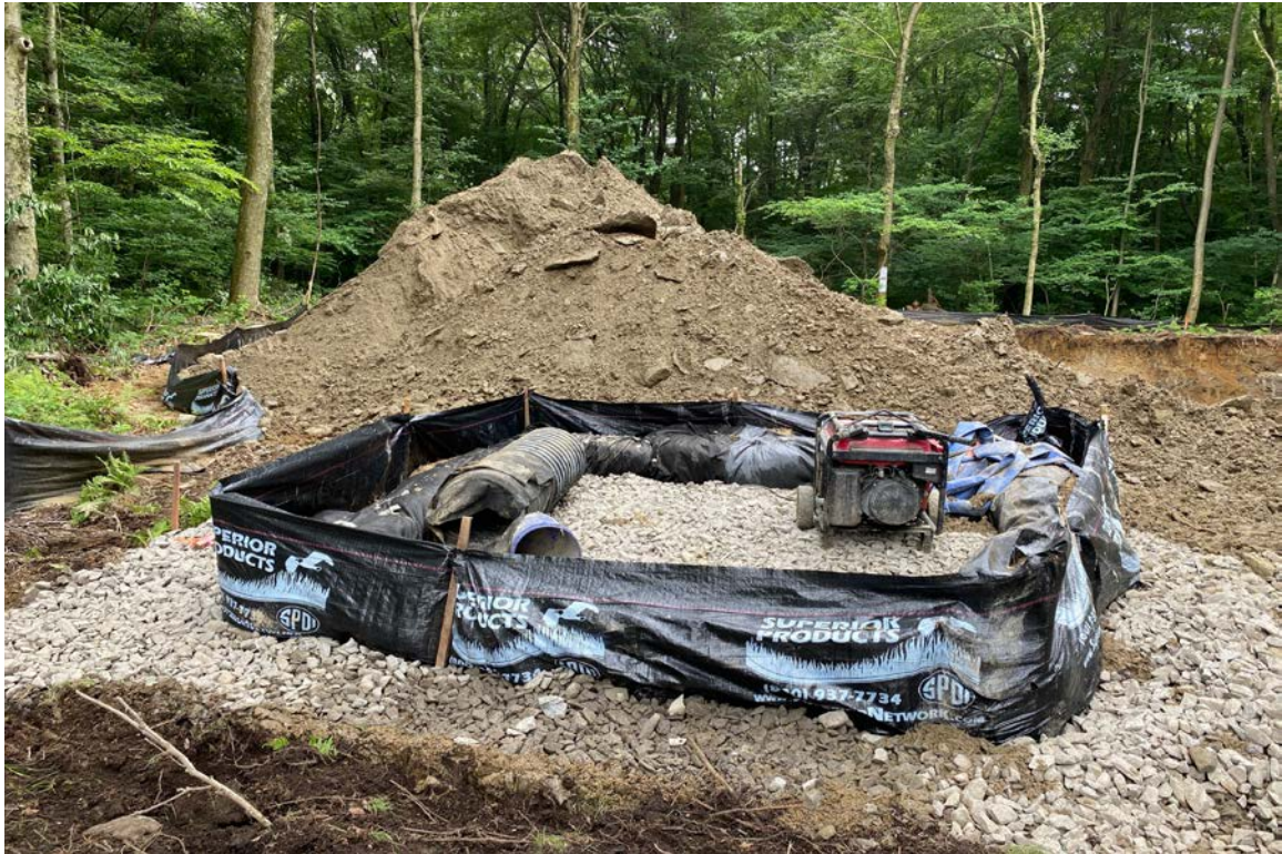
Photo 5: View of temporary dewatering basin to support foundation excavation work looking south.
