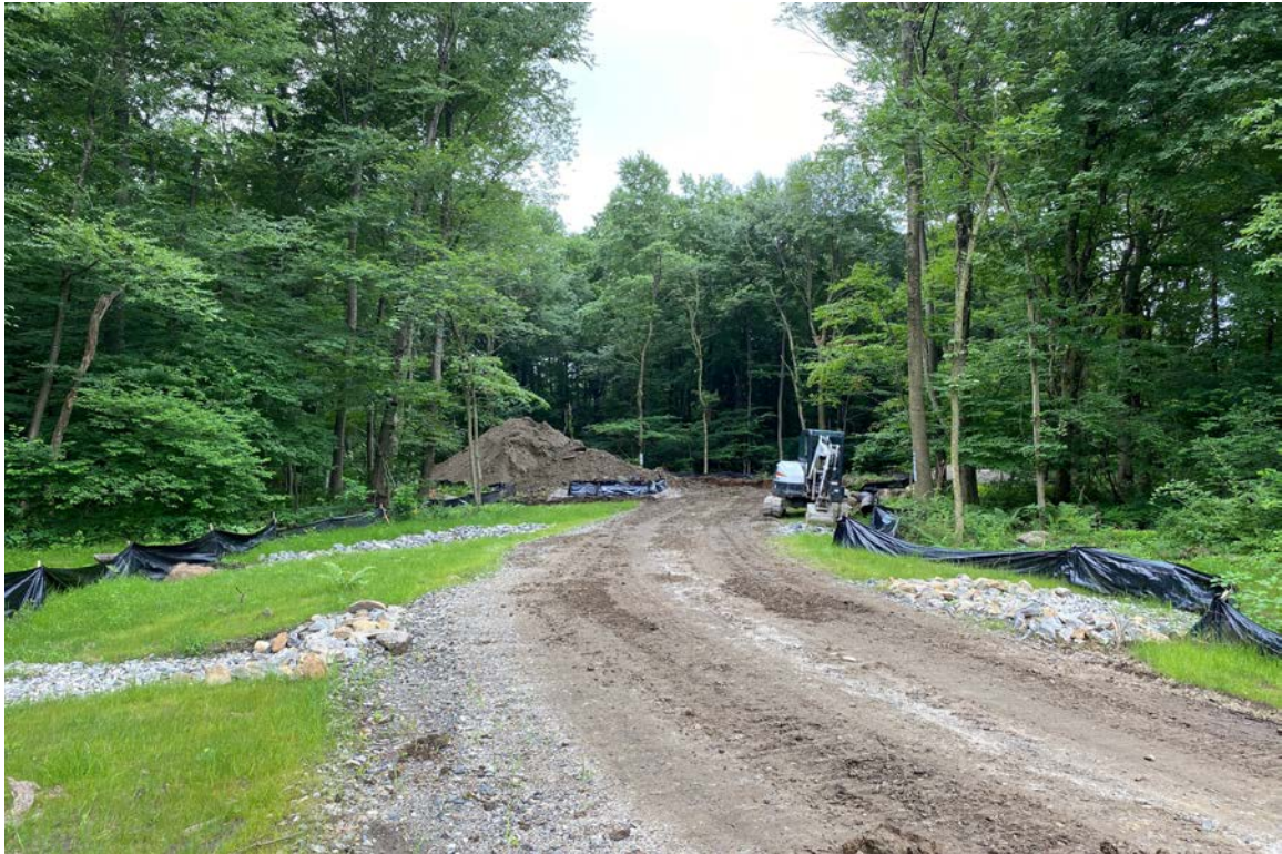
Photo 3: View of access road at French mattress and culverts crossing looking south with compound in background. Road shoulder and side slopes stabilized with well established permanent vegetation.
