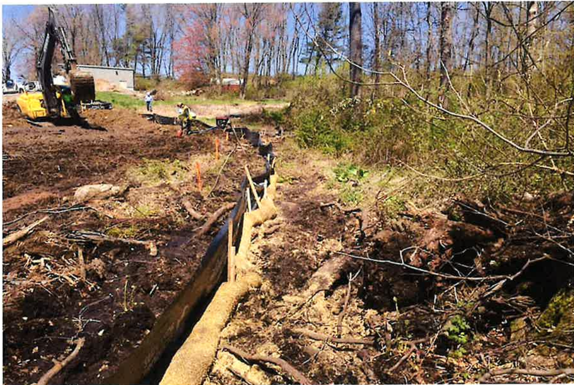
Photo 4: View of straw wattle added to the east side of silt fence for added protection, looking north.
