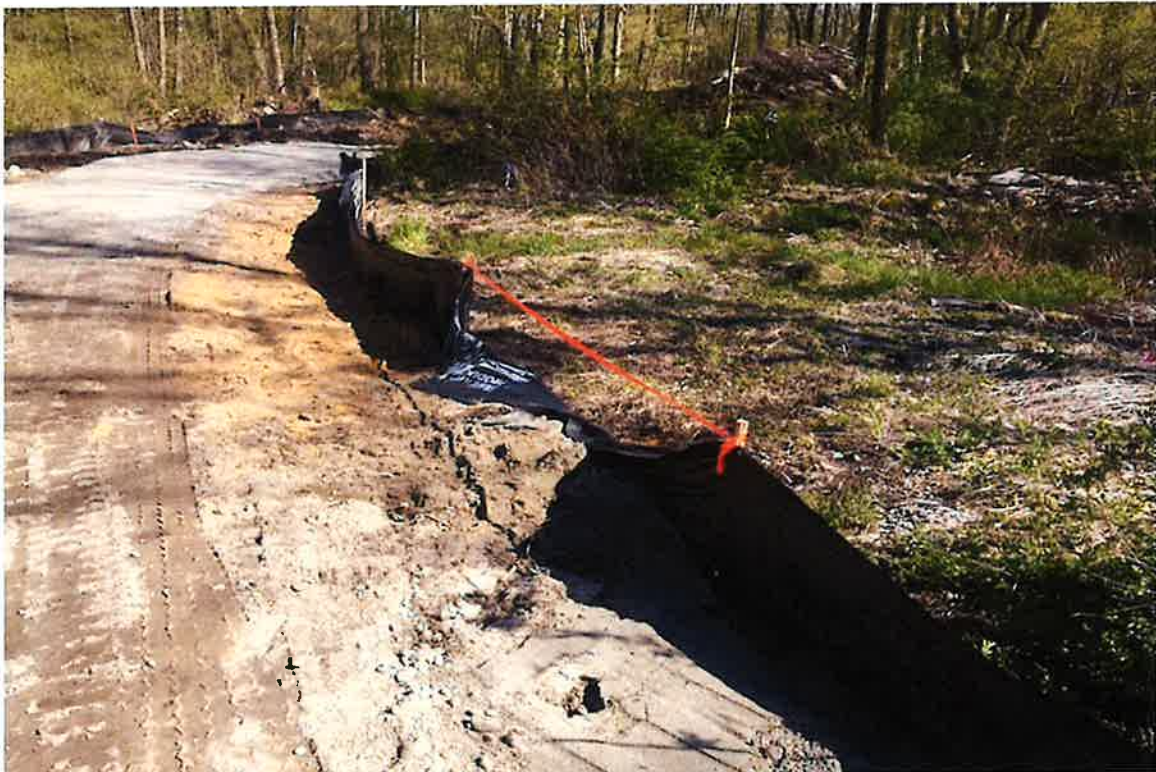
Photo 4: View of 10-foot section of silt fence needing repair along access road, looking south.
