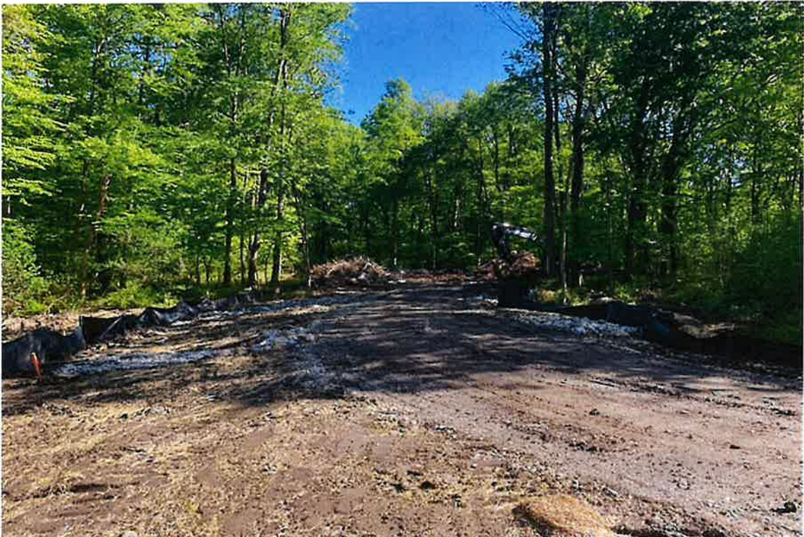
Photo 2: View of access road looking south across French mattress and two culverts section of road with compound in background.
