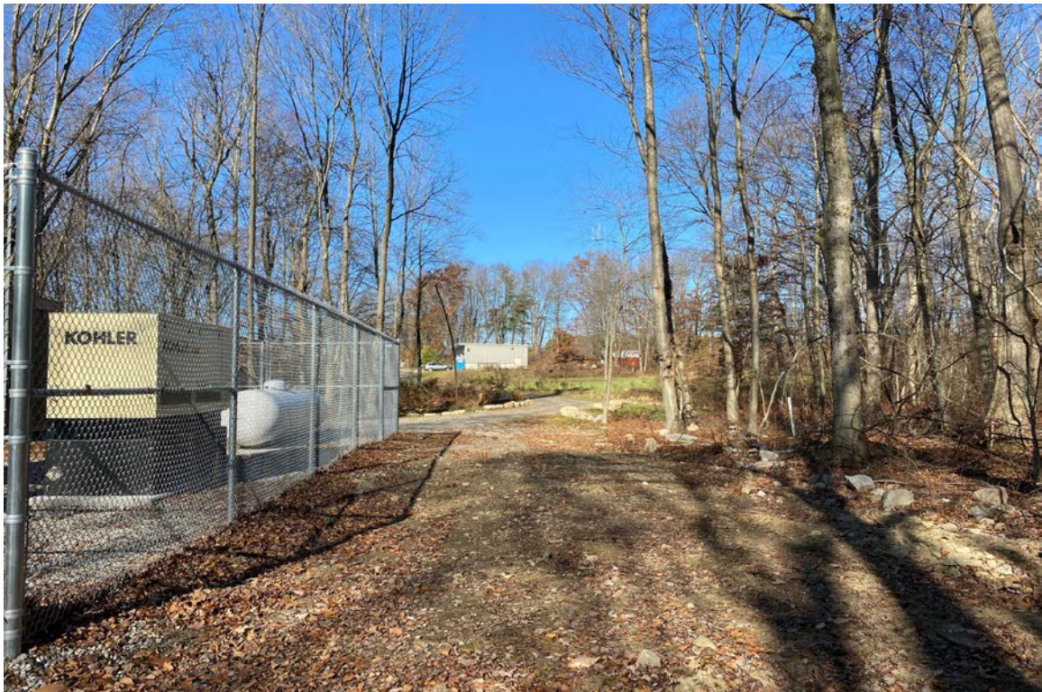
Photo 6: View of tower and compound area looking north with erosion controls removed.
