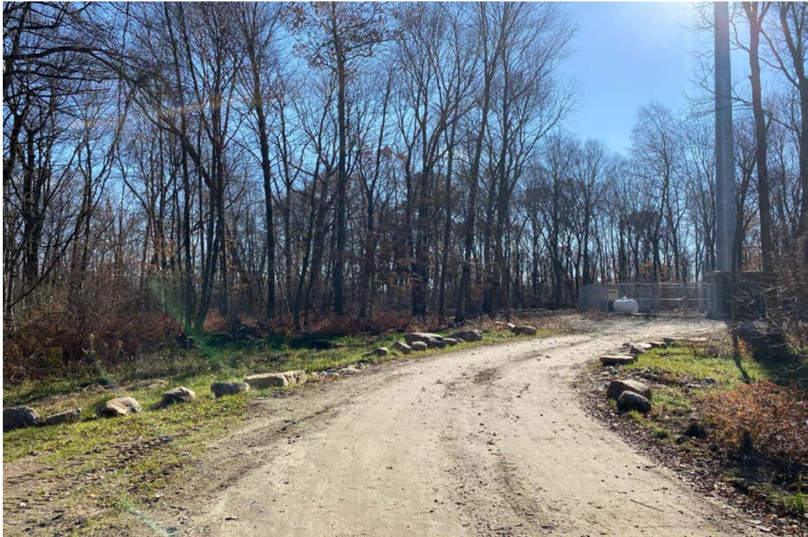
Photo 3: View of access road at French mattress and culverts crossing looking south with compound/tower in background. Road shoulder and side slopes stabilized with well established permanent vegetation and erosion controls removed.
