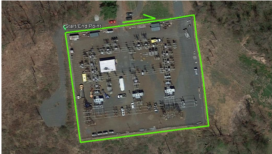
Figure C-1 – Measurement Path around Newington Substation
