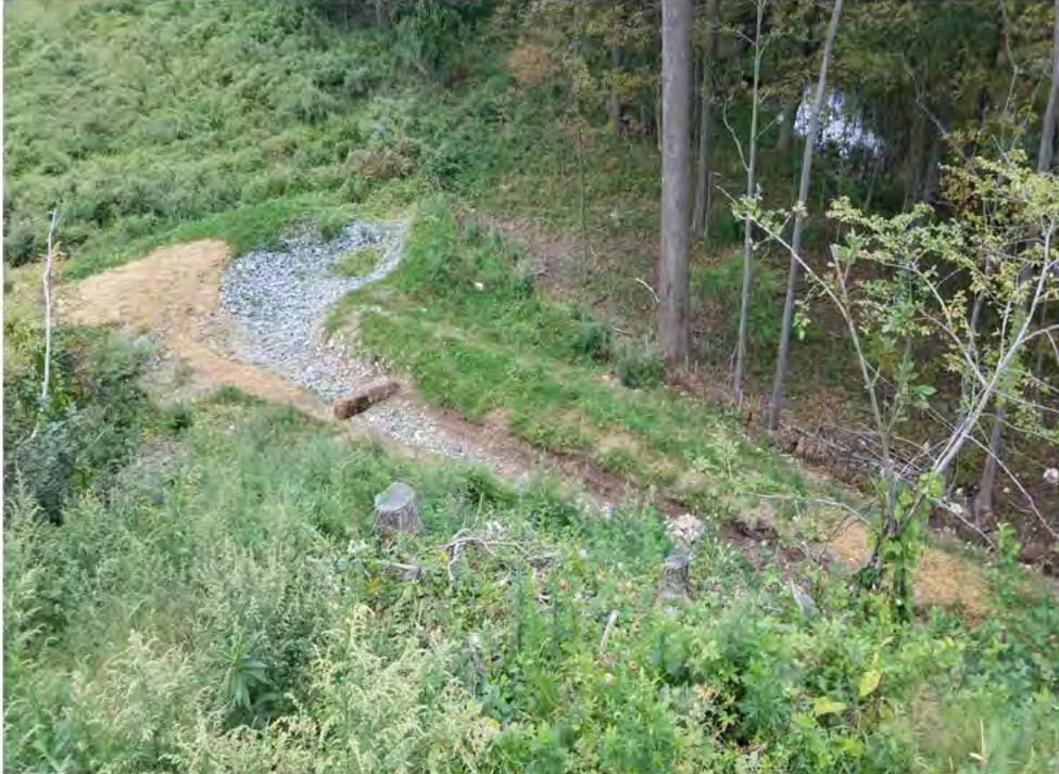
Photo 5: 09/20/2018, Danbury: Map 05, view of rip rap filled sediment basin and soil drainage swale with straw bales and/or rip rap check dams (Permanent BMPs), constructed along the bottom of the east slope, parallel with Wetland W1. Photo taken facing northeast from the structure work pad.
