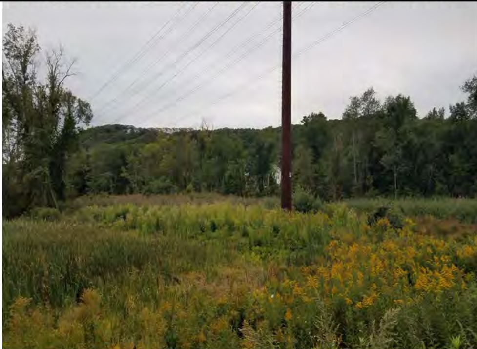
Photo 4: 09/20/2018, Bethel: Map 03, view of structure Str1007 located within wetland W1 off of Shelter Rock Road in a Rare Species Designated Area. All timber mats have been removed, all temporary anchor points were removed and initial restoration has been performed. Photo taken facing southwest.
