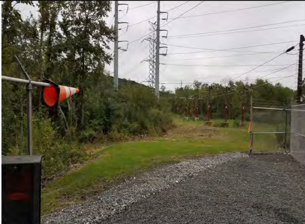
Photo 2: 09/20/2018, Bethel: Maps 01A-02, access road to Str1000 through Str1006, all timber mats removed from within Wetland W1 and initial restoration has been performed. Photo taken facing northwest from the southwest corner of the Plumtree Substation towards Str1003 in the distance.
