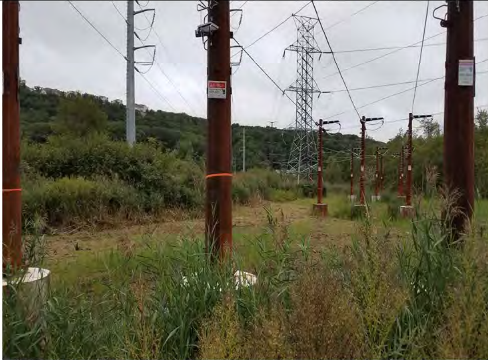
Photo 3: 09/20/2018, Bethel: Maps 01A-02, view of structures Str1000 through Str1003 within wetland W1. All timber mats removed and initial restoration performed. Photo taken facing northwest from Str1000 to Str1003 in the distance.
