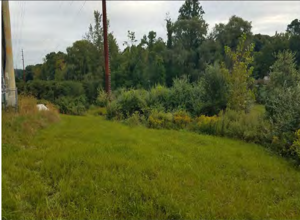
Photo 11: 09/20/2018, Bethel: Map 08, view of Structure Str1016 and access road, removal of timber mats, final grading, and initial restoration has been performed. Photo taken facing northeast from Chimney Drive towards Str1016 in the distance.
