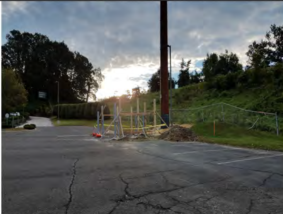
Photo 14: 09/27/2018, Bethel: Map 10, view of Str1019 restoration of ROW and the construction of fenced in area for the property owner's refuse/recycling container staging area.
