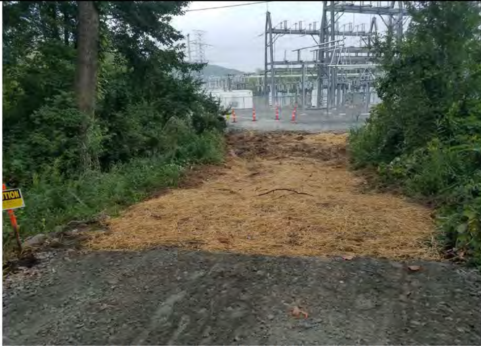
Photo 1: 09/20/2018, Bethel: Maps 01A-01, access road to Str1000 through Str1006 at the culvert crossing of Wetland W1 outside of the southeast fence line of the Plumtree Substation. Timber mats removed and initial restoration performed. Photo taken facing northwest from the southeast side of the culvert area towards the Plumtree Substation in the distance.
