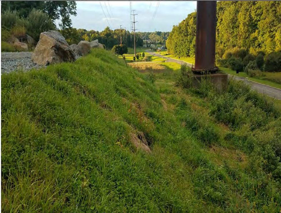
Photo 16: 09/27/2018, Bethel/Brookfield: Map 12, Str1023, north-south view of west slope of work pad where previous erosion occurred. Area has been stabilized with seed and straw mulch. At the time of this inspection grass was growing and no erosion was observed.
