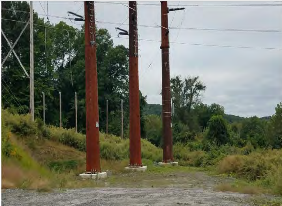
Photo 12: 09/20/2018, Bethel: Map 07, view of Str1027, Final grading and initial restoration has been performed. Stone work pad is staying in place, natural revegetation is occurring. No soil erosion observed, upland slope and pad appears to be stable at this time. Photo taken facing west towards Str1027.
