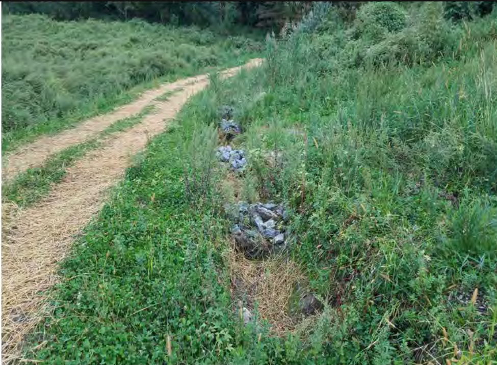
Photo 6: 09/20/2018, Danbury: Map 05, view of grass filled drainage swale with rip rap check dams (Permanent BMPs), constructed along the bottom edge of the north slope and connecting to the sediment basin shown in Photo 5 above, parallel with the pad and along the limits of disturbance as shown on Map Sheet 05. Photo taken facing east.
