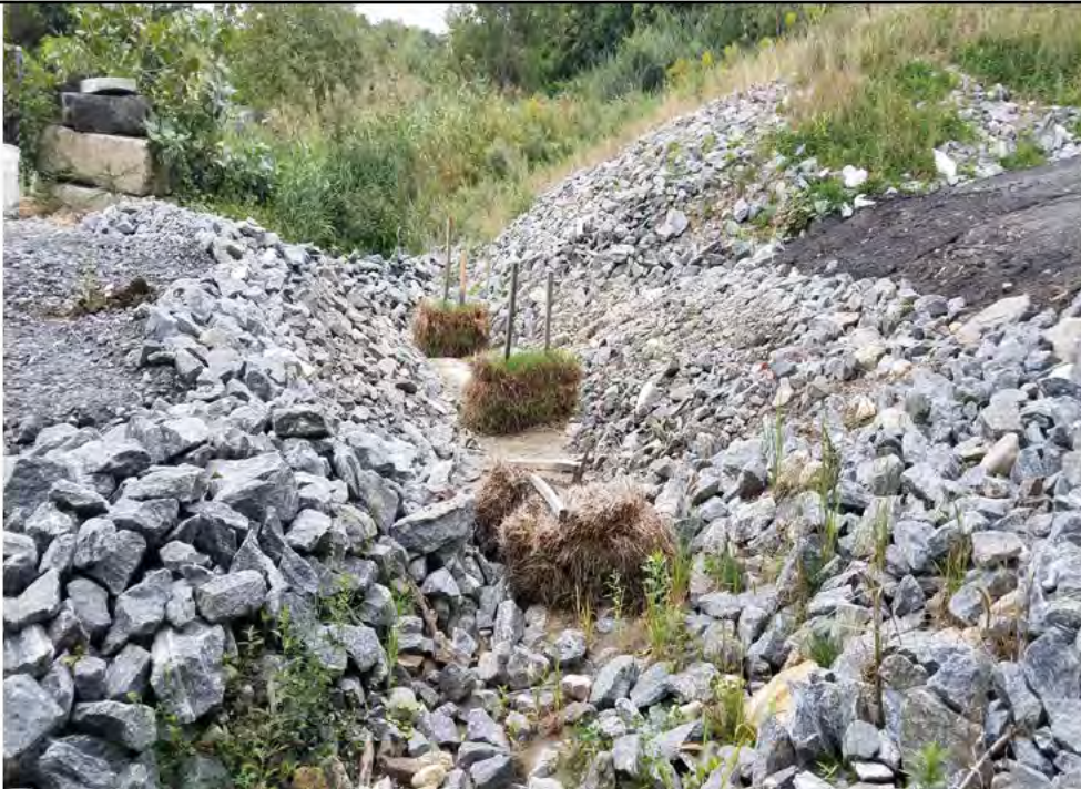
Photo 8: 09/20/2018, Danbury: Map 06, view of rip rap filled swale, sediment basin, and straw check dams constructed at the intersection of the Unnamed watercourse and the access road to Str1013, south end of Old Sherman Turnpike. A temporary rip rap filled hard bottom crossing has been removed and the final rip rap drainage swale and sediment basin is now in place (Permanent BMPs). Photo taken facing north parallel with Old Sherman Turnpike.
