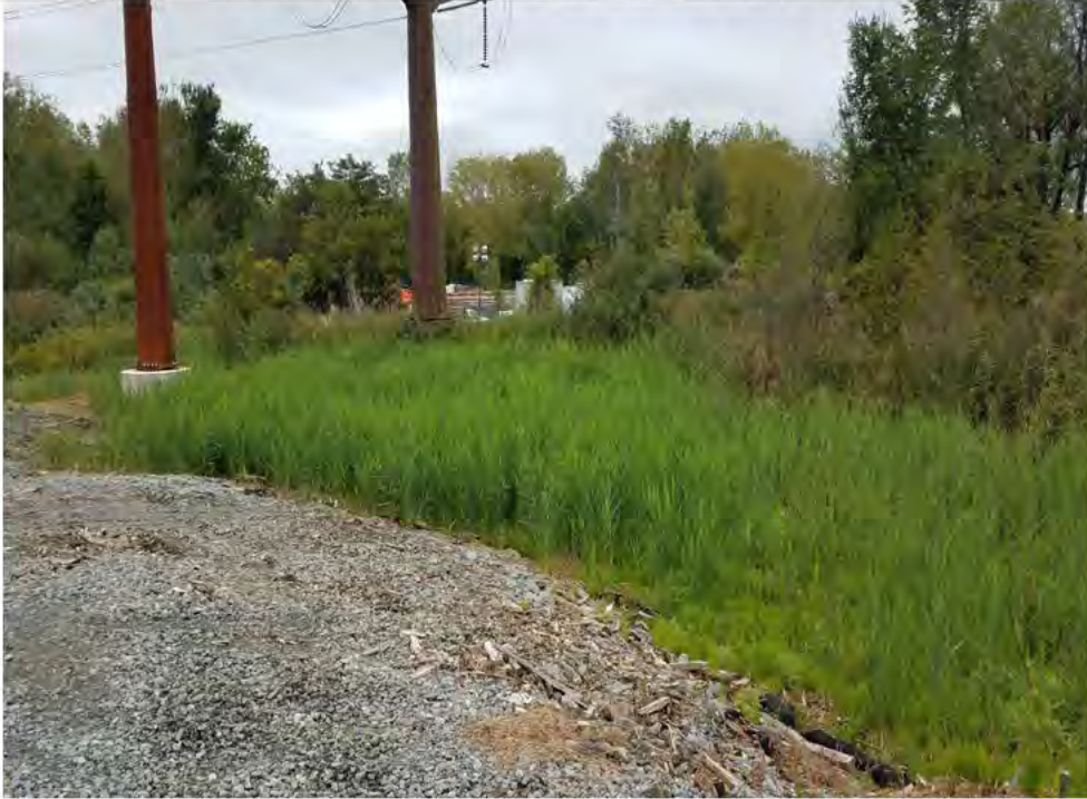
Photo 7: 09/20/2018, Danbury: Map 06, view of Str1012 and access point to Str1012 and Str1011 (to the south, not shown in this view). Gravel pull pad to remain in place, timber mat access road and work pads removed. Initial restoration performed and natural revegetation visible. Photo taken facing west from the pull pad towards Str1012.
