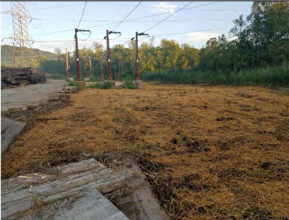
Photo 2: 08/30/2018, Danbury: Map 1, the timber mat work pad areas from Str1000 through to Str1003 have been removed and counterpoise completed. Initial stabilization/restoration has been performed. Photo taken facing west, west of Str1000.
