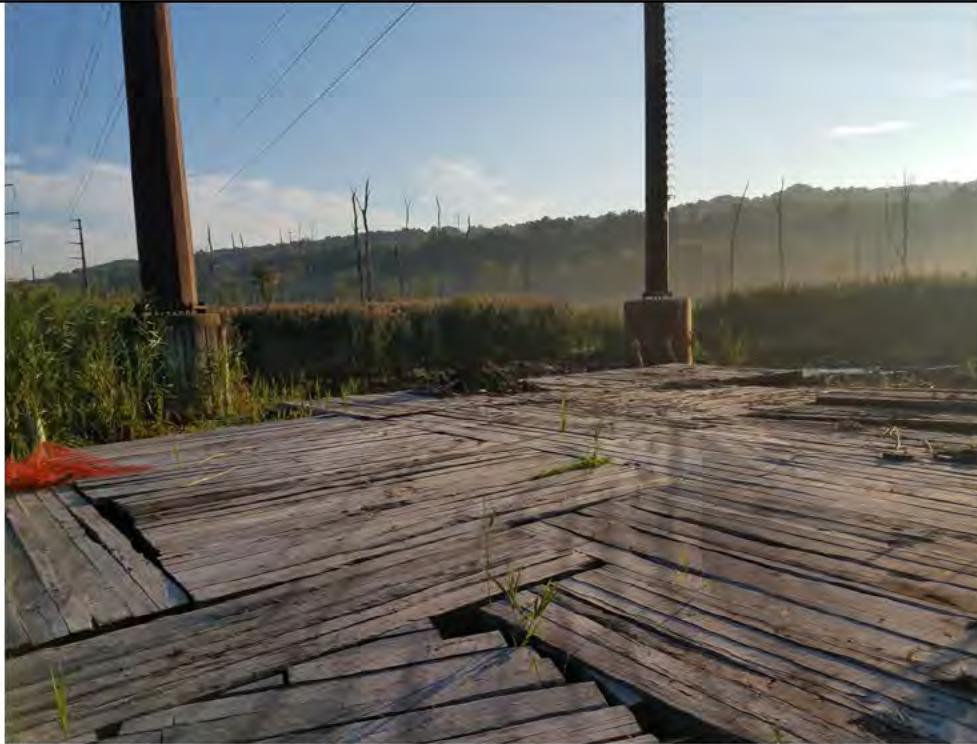
Photo 3: 08/30/2018, Danbury: Map 5, Str1010, partial timber mat pad and access road removal, and initial restoration being performed. Timber mats have been removed north and east of the structures. Photo taken facing northeast.
