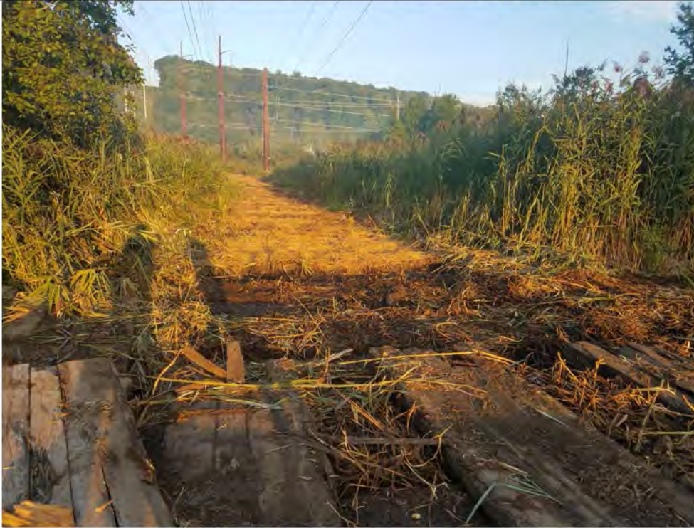
Photo 1: 08/30/2018, Danbury: Map 2, the timber mat access road and structure work pads west of Str1003 through to Str1006 have been removed. Initial stabilization/restoration has been performed. Photo taken facing west, west of Str1003.
