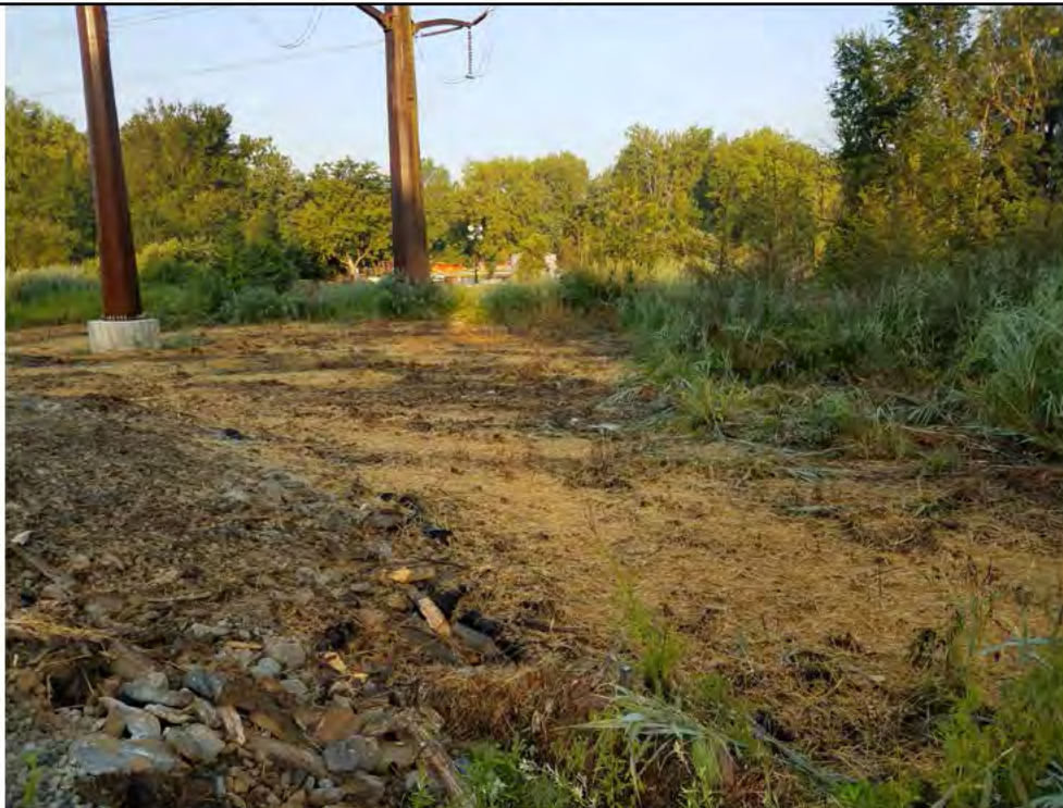
Photo 4: 08/09/2018, Danbury: Map 6, Str1011 and Str1012 (shown in photo), timber mat pads and access road removed, and initial restoration performed. Photo taken facing west.
