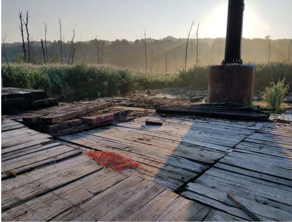
Photo 1: 08/09/2018, Danbury: Map 5, Str1010, timber mat pad and access road removal, and initial restoration being performed. Photo taken facing northeast.
