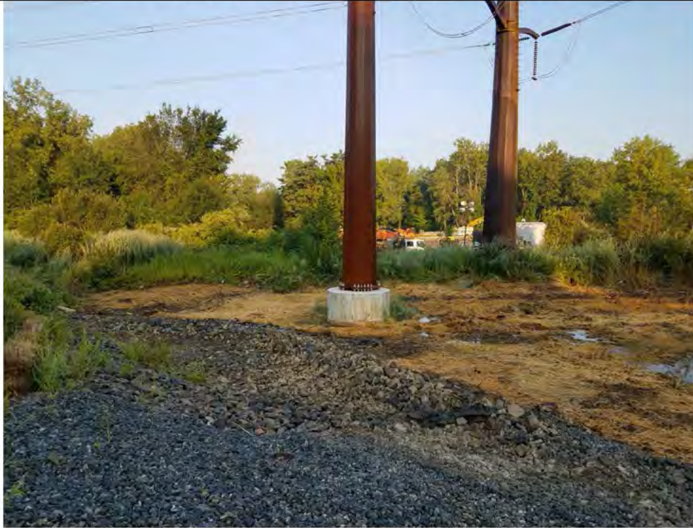
Photo 3: 08/09/2018, Danbury: Map 6, Str1011 and Str1012 (Str1012 shown in photo), timber mat pads and access road removed, and initial restoration performed. Photo taken facing northwest.
