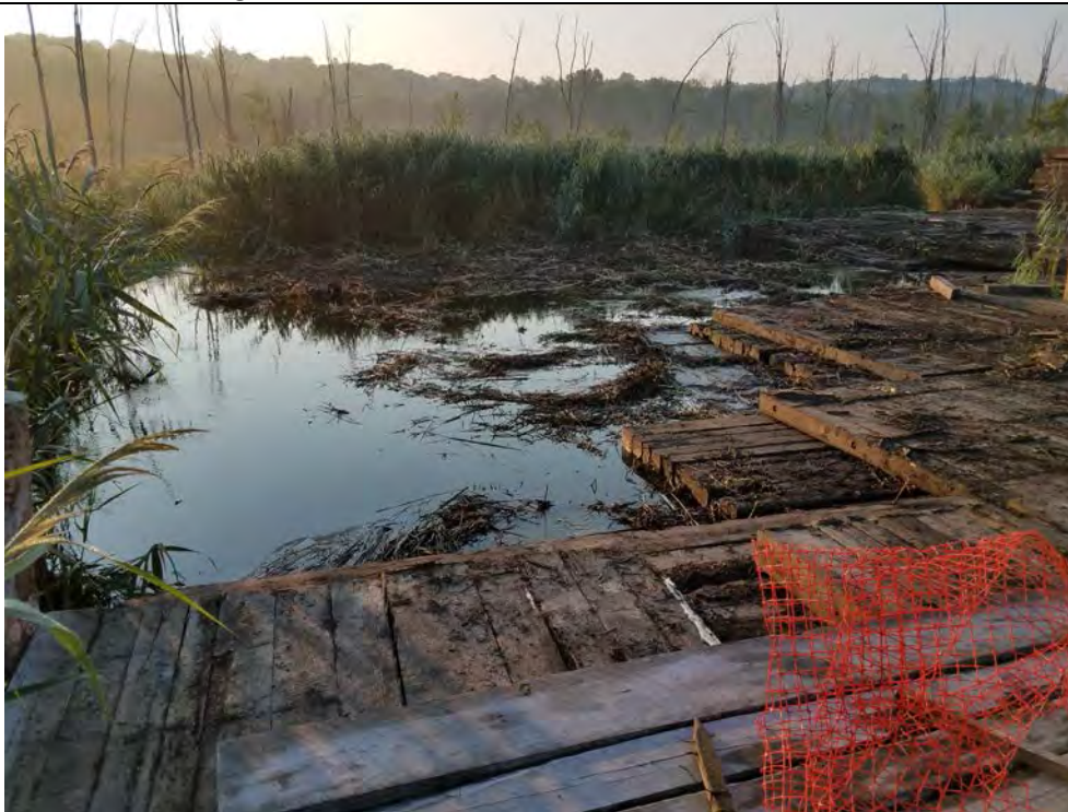
Photo 2: 08/09/2018, Danbury: Map 5, Str1010, timber mat pad and access road removal, and initial restoration being performed. Photo taken facing east.
