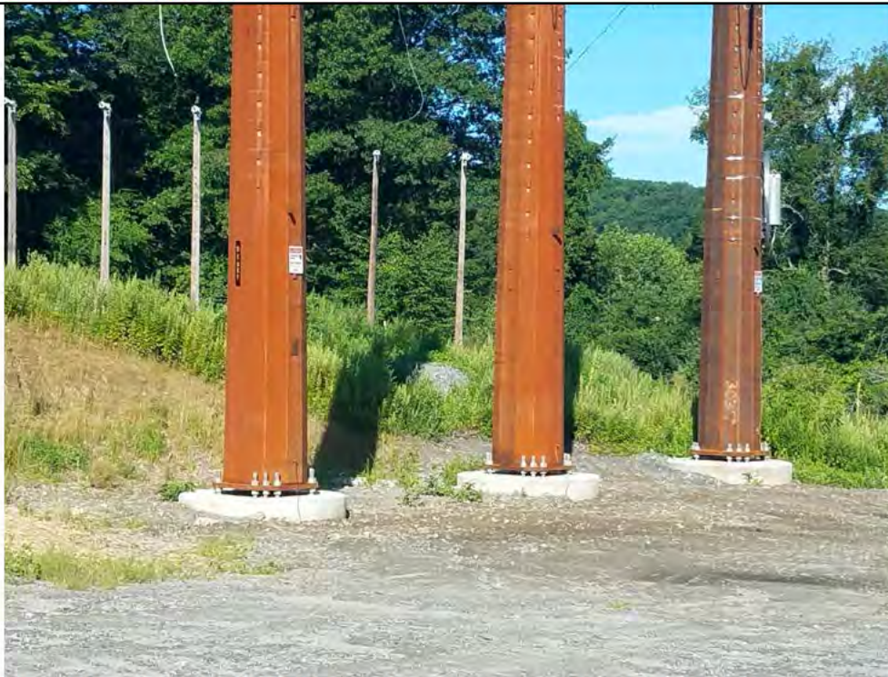
Photo 18: 08/02/2018, Bethel: Map 13, Str1027, Counterpoise system, trench backfilled and graded (see previous photo, Photo 4). Photo taken facing west.
