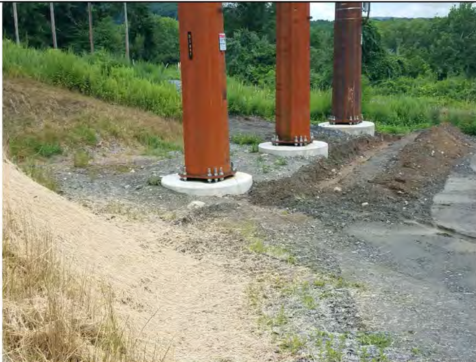
Photo 4: 07/26/2018, Bethel: Map 13, Str1027, trenching and installation of grounding cables for Counterpoise system. Photo taken facing west.
