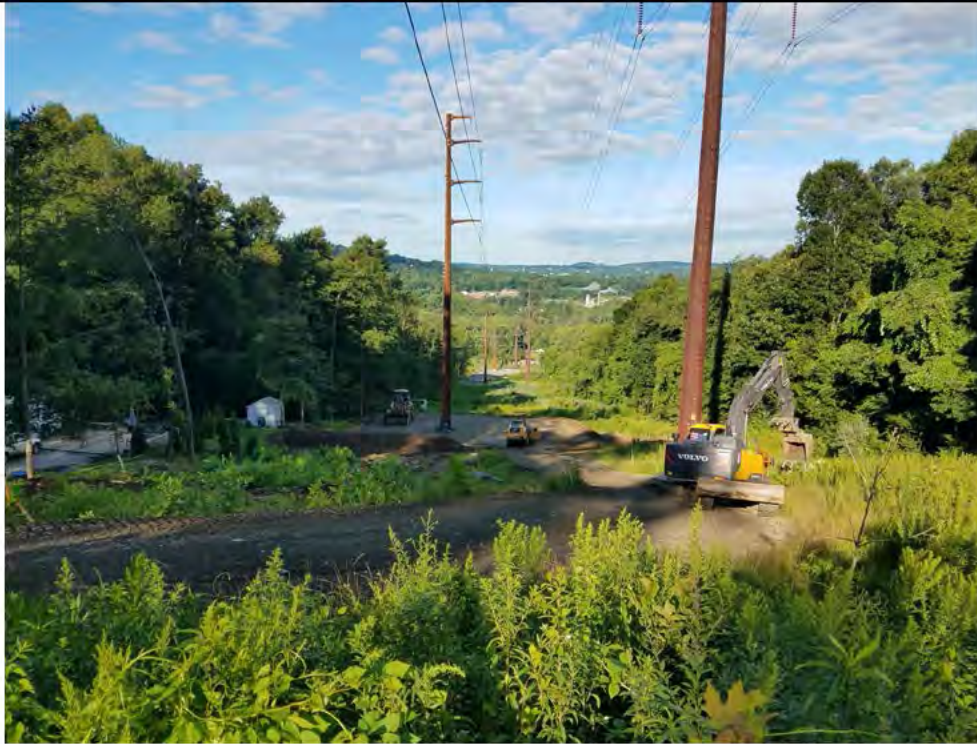
Photo 5: 08/02/2018, Danbury: Map 07, Str1014, work pad and access road restoration being performed by Supreme. Photo taken facing west.
