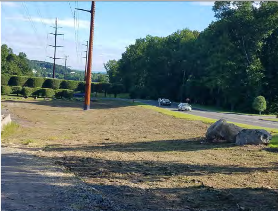
Photo 12: 08/02/2018, Brookfield: Map 13, Str1024, property owner performed work pad restoration (grading and hydroseeding). Photo taken facing north.
