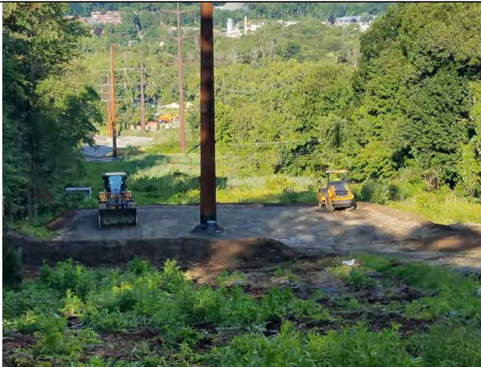
Photo 6: 08/02/2018, Danbury: Map 07, Str1014, work pad restoration being performed by Supreme. Photo taken facing west.
