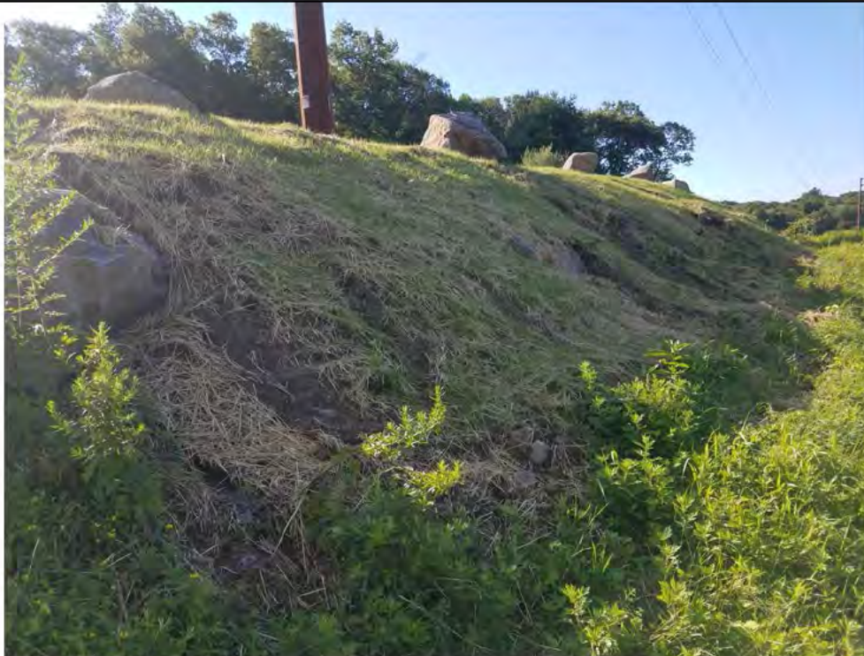
Photo 14: 08/02/2018, Bethel/Brookfield: Map 12, Str1023, slope erosion, west slope. Reference Additional Comments section Page 6 for additional details. Photo taken facing south.
