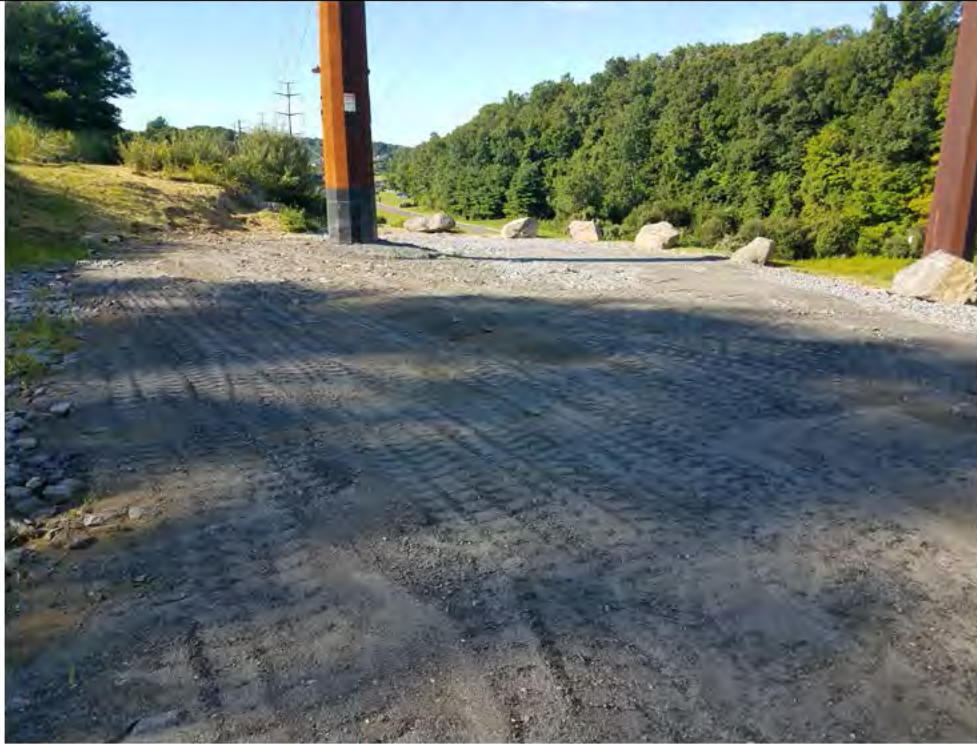
Photo 13: 08/02/2018, Bethel/Brookfield: Map 12, Str1023, work pad restoration (grading and boulder placements). Photo taken facing south.
