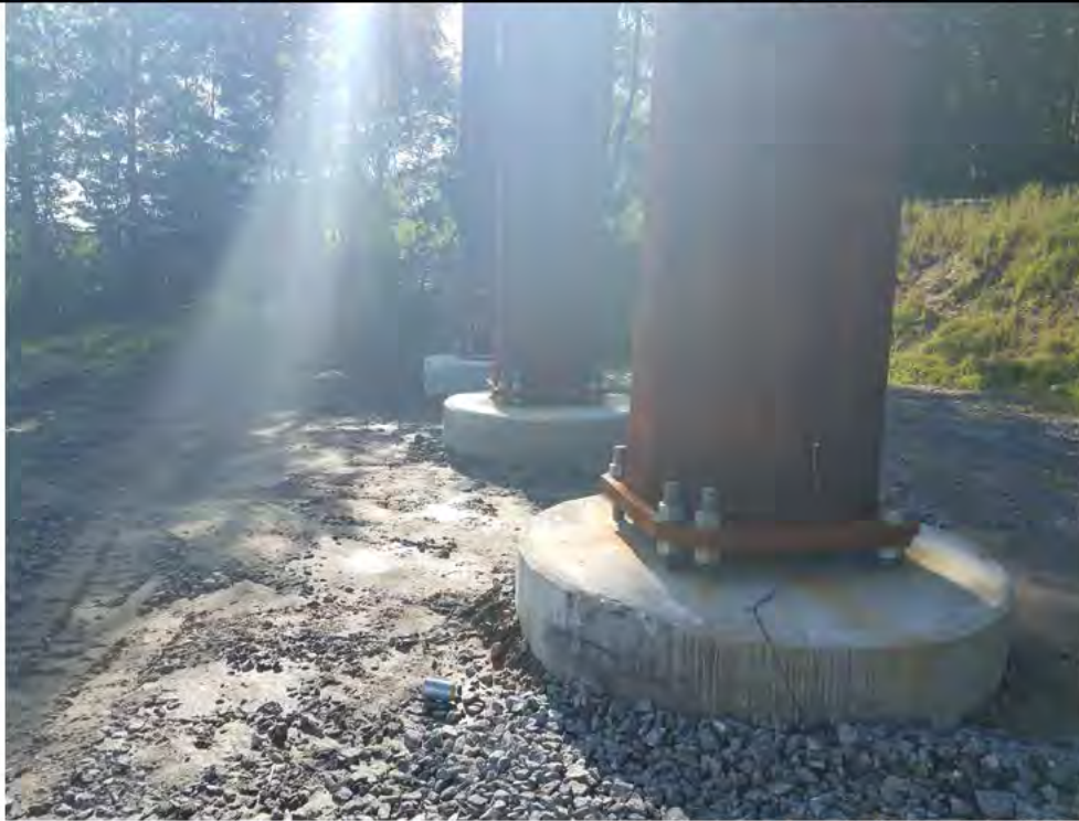
Photo 17: 08/02/2018, Bethel: Map 13, Str1026, Counterpoise system, trench backfilled and graded (see previous photo, Photo 3). Photo taken facing east.
