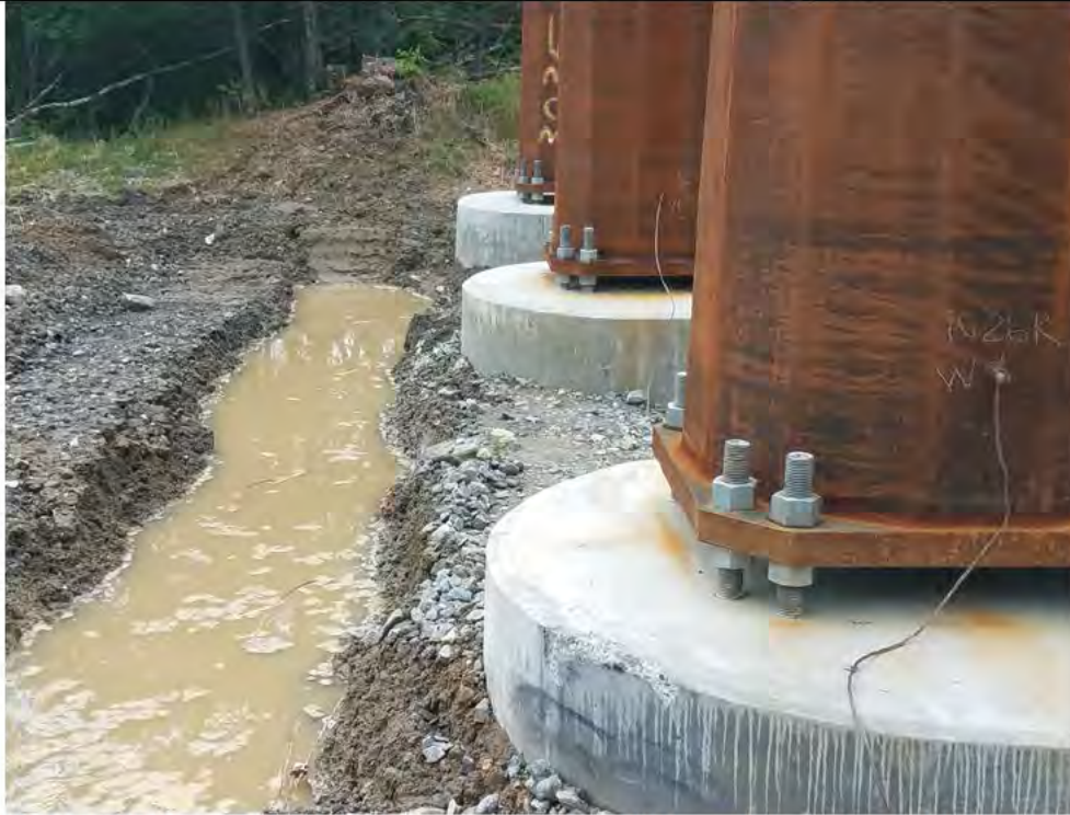
Photo 3: 07/26/2018, Bethel: Map 13, Str1026, trenching and installation of grounding cables for Counterpoise system. Photo taken facing east.
