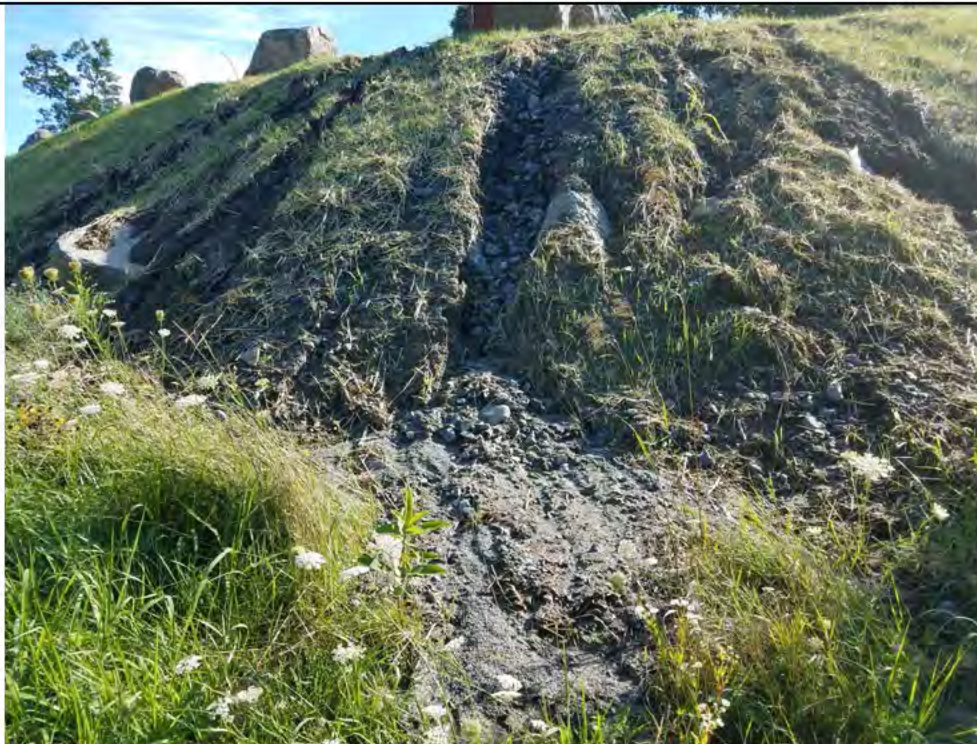
Photo 16: 08/02/2018, Bethel/Brookfield: Map 12, Str1023, slope erosion, southwest corner of slope. Reference Additional Comments section Page 6 for additional details. Photo taken facing northeast.
