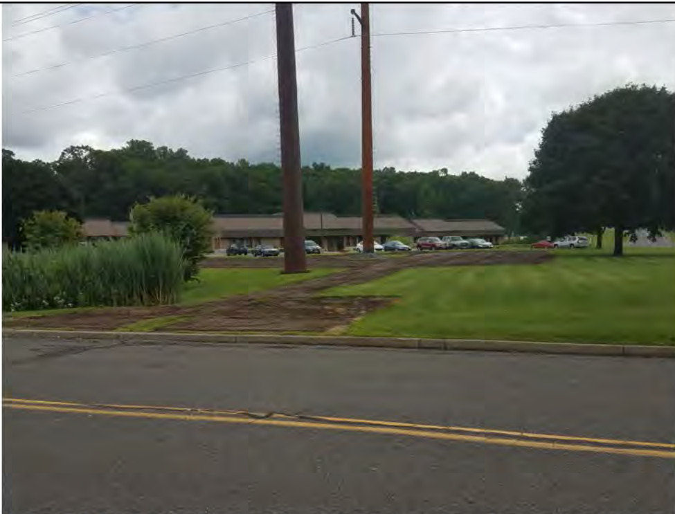
Photo 2: 07/26/2018, Bethel: Map 12, Str1022, access road to the structure area as well as the work pad constructed of wood mats has been removed. Wetland W5 is abutting to the north. Photo taken facing east. All appears to be in accordance with Eversources's BMP Manual. Area will be restored with loam and hydroseeding within the next week.
