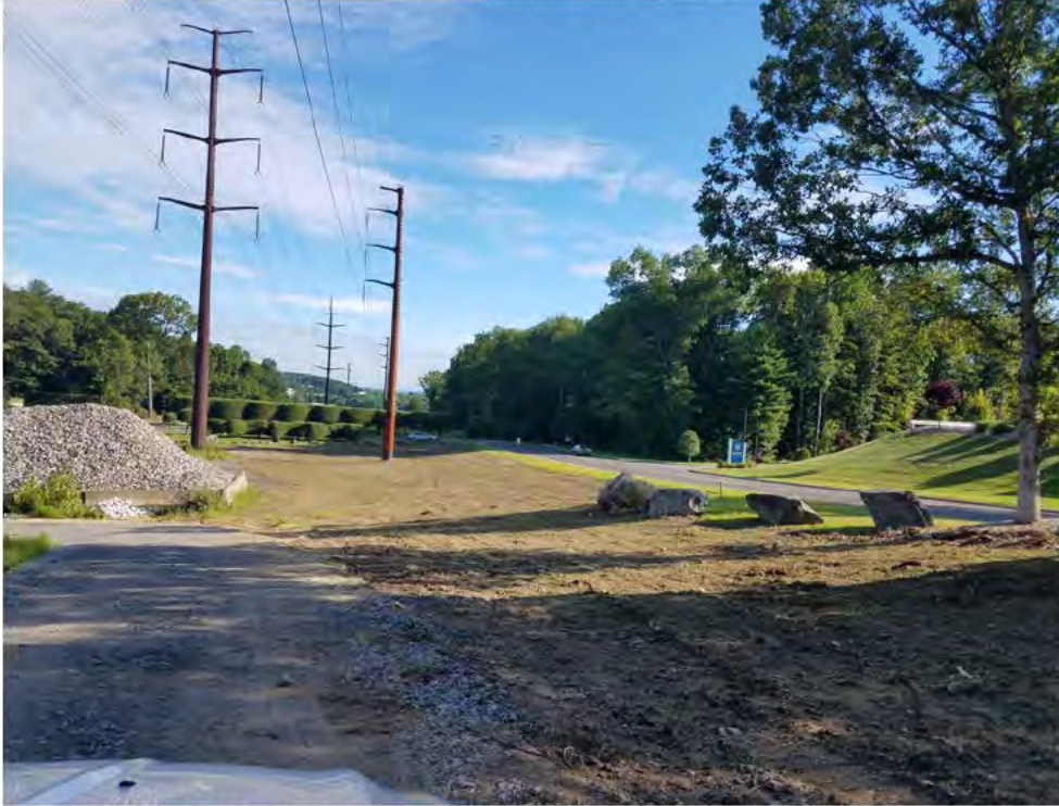
Photo 11: 08/02/2018, Brookfield: Map 13, Str1024, property owner performed work pad restoration (grading and hydroseeding). Photo taken facing north.
