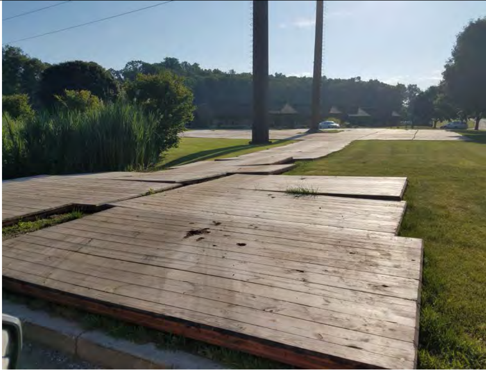
Photo 3: 07/13/2018, Bethel: Map 12, Str1022, access road to the structure area as well as the work pad is constructed with wood mats. Wetland W5 is abutting to the north. Photo taken facing east. All appears to be in accordance with Eversources's BMP Manual.
