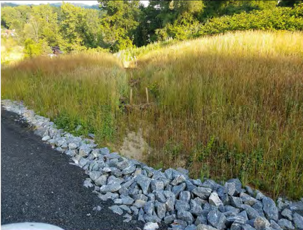
Photo 2: 07/13/2018, Danbury: Map 06, Str1013, slope stabilization (revegetation of disturbed area), drainage swale and temporary E&S controls (straw bale check dams) all appear to be in accordance with Eversource's BMP Manual. Photo taken facing north in the direction of Str1012.
