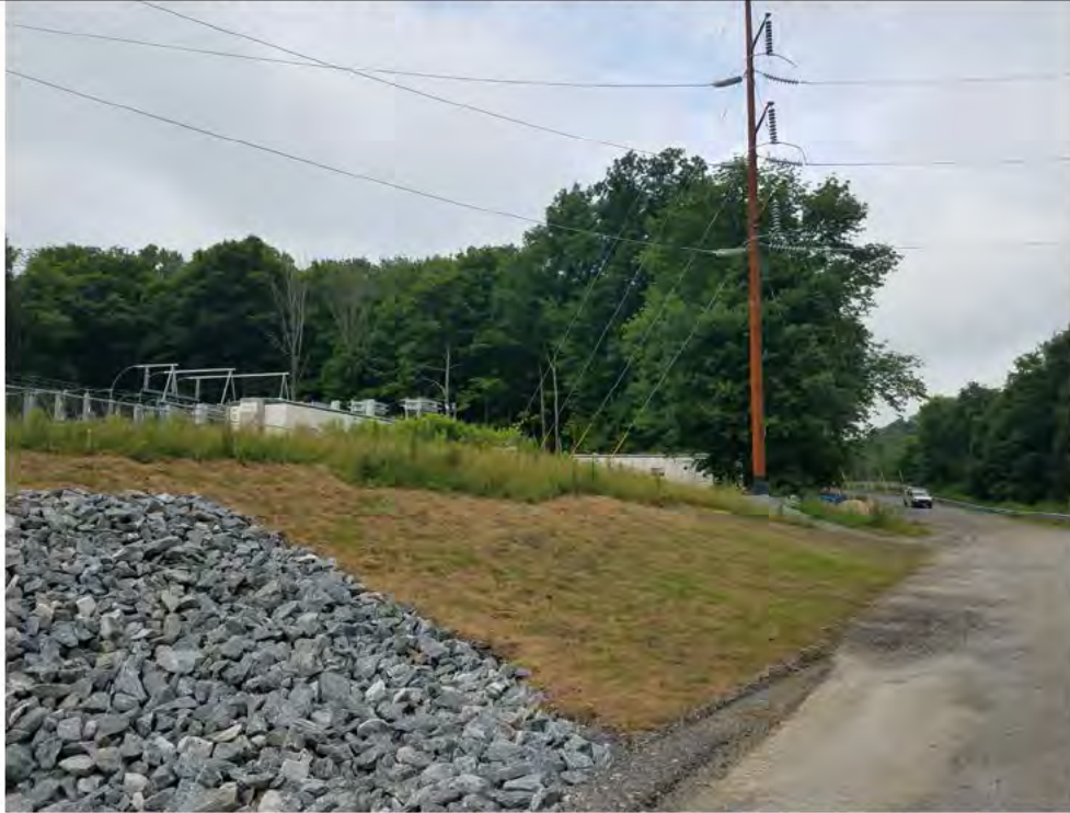
Photo 1: 07/05/18, Stony Hill Substation Str4648A stabilization of disturbed ground surfaces. Photo taken facing west along the Stony Hill Substation access road towards the Town of Brookfield Stony Hill Road.
