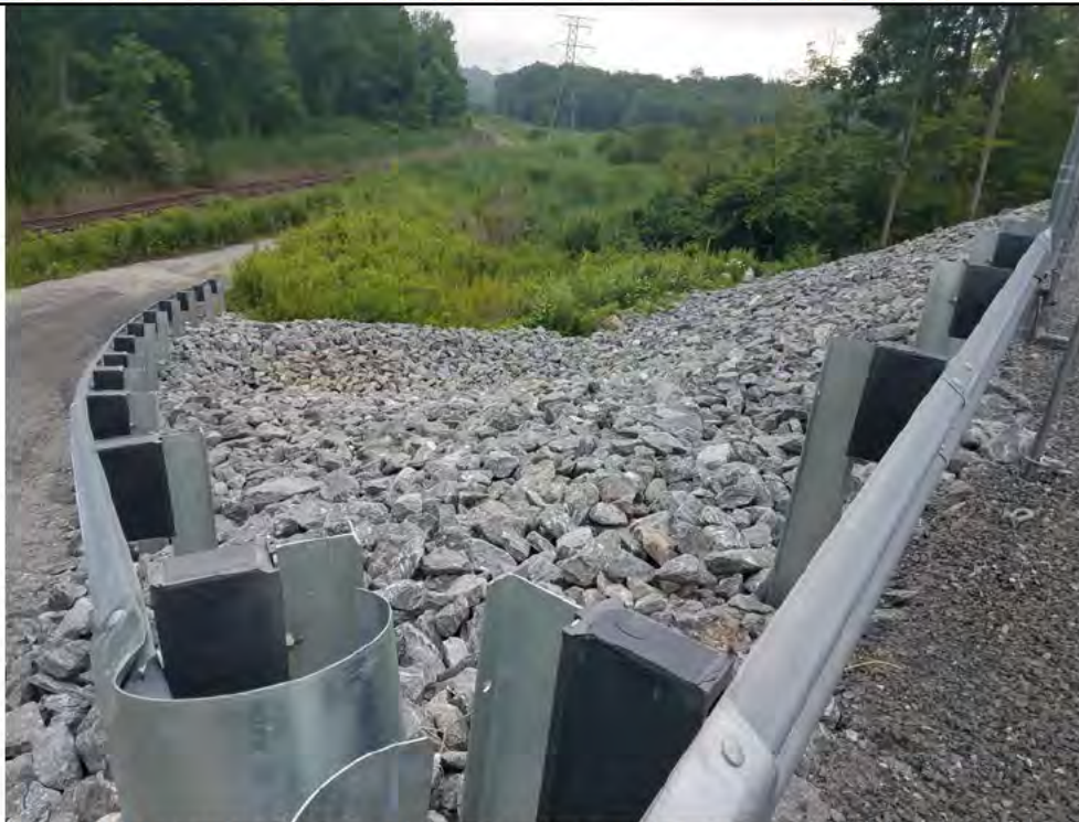
Photo 2: 07/05/18, Stony Hill Substation slope stabilization and site drainage feature abutting wetland W7. Photo taken facing northeast toward wetland W7.
