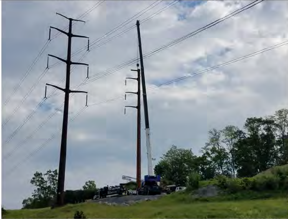
Photo 1: 05/31/2018, Brookfield: Map 12, Str1023, Michels setting the structure pole. Photo taken facing northeast from the area of Research Drive.
