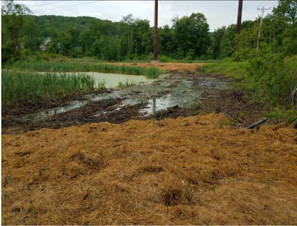
Photo 3: 05/31/2018, Bethel: Map 03, Str1007 and Wetland W1, Removal of timber mat access and work pad. Photo taken facing west, structure Str1007 shown central in the photo.
