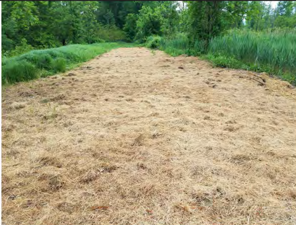
Photo 2: 05/31/2018, Bethel: Map 03, temporary equipment staging area for Str1007, removal of timber mat access and work pad. Photo taken facing south, town maintenance shed in the distance.
