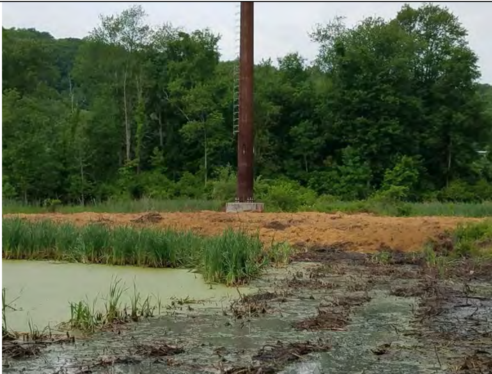
Photo 4: 05/31/2018, Bethel: Map 03, Str1007 and Wetland W1, Removal of timber mat access and work pad. Photo taken facing west, structure Str1007 shown.
