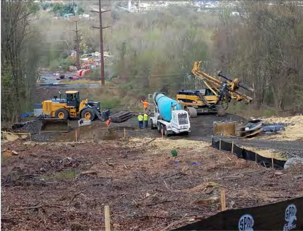
Photo 1: 05/04/2018, Bethel: Map 07, Michels drilling direct embed foundation at Str1014. Photo taken facing west toward Str1014 from Hearthstone Drive.
