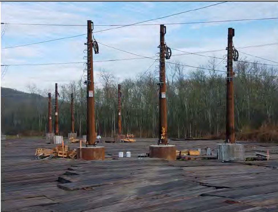
Photo 2: 05/04/2018, Bethel: Map 01, Str1000 through Str1003, weathered steel structures installed. Photo taken facing northwest from Str1000 toward Str1003 in the distance.
