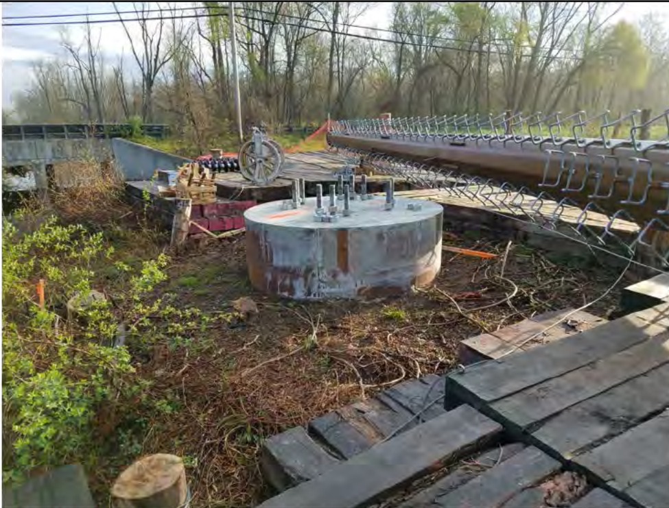
Photo 4: 05/04/2018, Bethel: Map 03, weather steel structure assembled and ready for installation. All drill cuttings removed from the area, little to no ground impacts outside of the foundation area within Wetland W-1. Photo taken facing north toward Shelter Rock Road.
