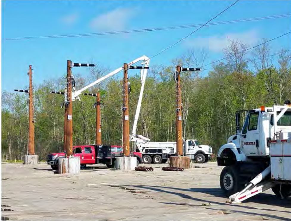
Photo 5: Bethel: Map 01, Str1002 through Str1003, set up to start pulling line, Str1000 through Str1005. Photo taken facing northwest.
