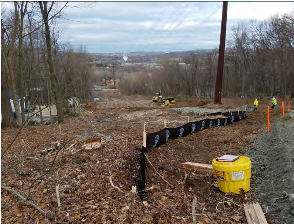
Photo 2: 04/18/2018, Bethel: Map 07, access road and pad construction at Str1014. Photo taken facing west towards Str1014 from Hearthstone Drive.
