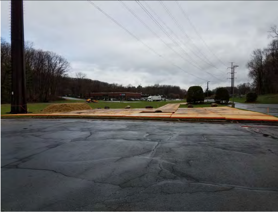
Photo 7: 04/26/2018, Bethel, Map 10, temporary matting for work pad and access road at Str1020, photo taken facing north toward Str1020 from the property paved lot.
