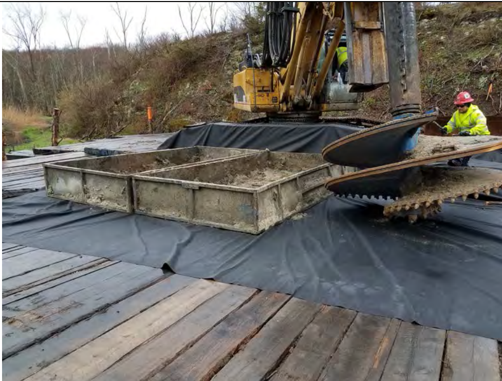
Photo 4: 04/26/2018, Danbury, Map 04, drilling equipment staged on the work pad, photo taken at Str1008.
