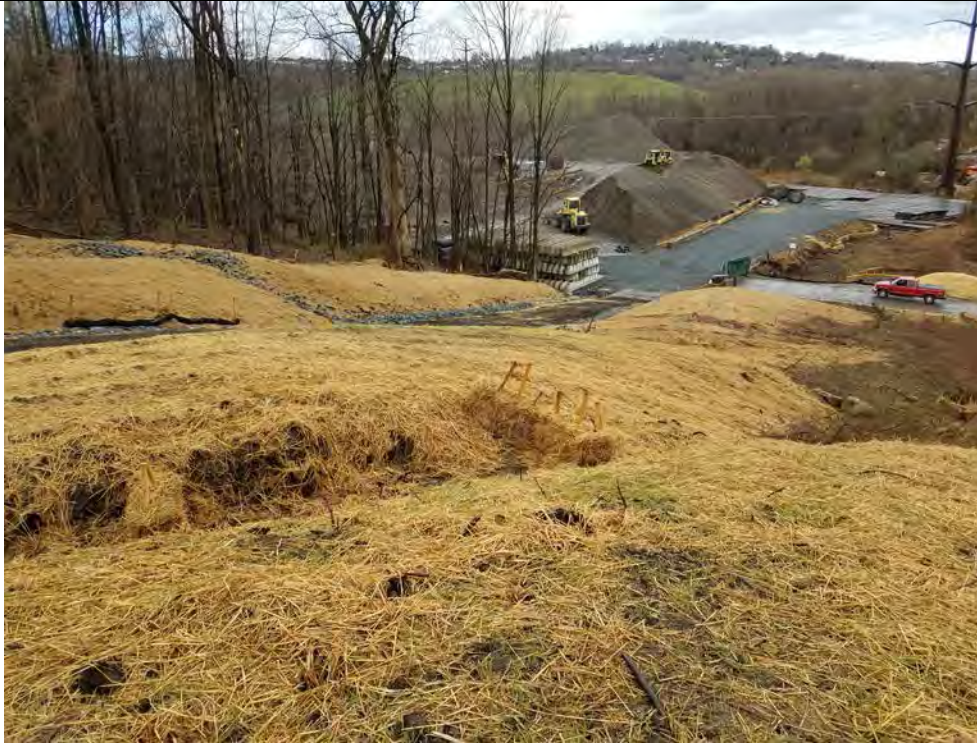
Photo 5: 04/26/2018, Danbury, Map 06, slope and exposed soil stabilization and various E&S controls implemented west of Str1013 down to Old Sherman Turnpike and the access road to Str1012-Str1011, photo taken facing west from Str1013.
