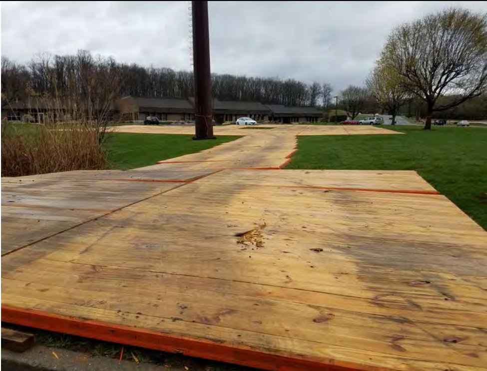
Photo 8: 04/26/2018, Bethel, Map 10, temporary matting for work pad and access road at Str1019, photo taken facing south toward Str1019 from the property paved lot.
