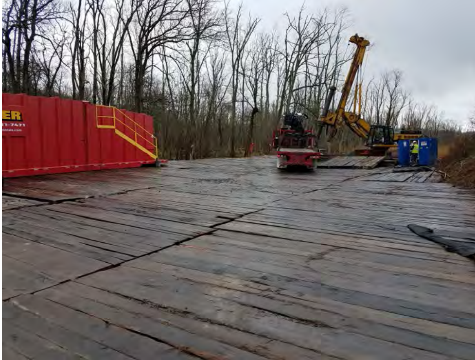
Photo 3: 04/26/2018, Danbury, Map 04, Frac tank and drilling equipment staged on the work pad, photo taken facing south toward Str1008.
