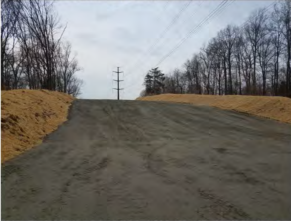
Photo 3: 04/13/2018, Bethel: Map 07, work and Pull pad west side of Str1015. Photo taken facing west.
