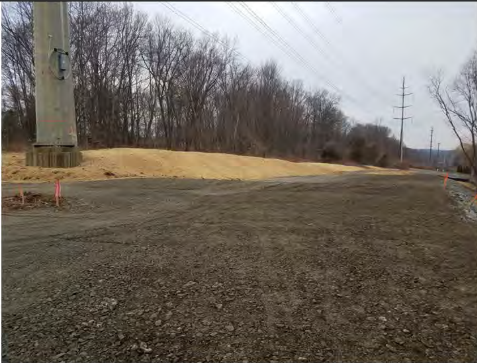
Photo 4: 04/13/2018, Bethel: Map 07, Work and Pull pad north side of Str1015. Photo taken facing north.
