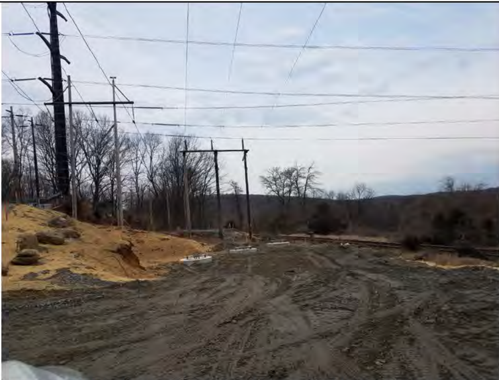
Photo 6: 04/13/2018, Brookfield: Map 13, Str1027 structure foundations. Photo taken facing west
