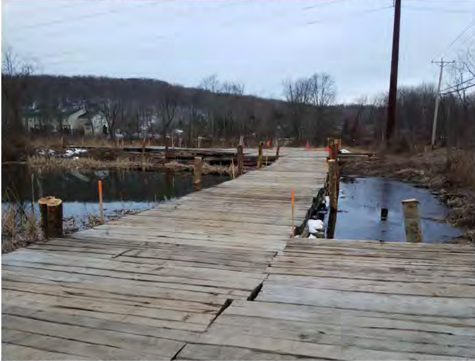
Photo 3: 03/23/2018, Bethel: Map 03, Str1007 timber mat access and work pad through Wetland W1.
