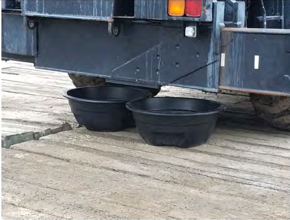
Photo 1: 03/23/2018, Bethel: Map 02, Str1000-1006, photo of spill protection under operating equipment/staged equipment, over timber mats placed within wetland W1.
