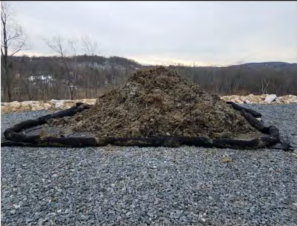
Photo 4: 03/23/2018, Danbury: Map 05, Str1009 work pad area, staged Wetland invasive species seed bank segregation material excavated from the top 4.5-feet of the landfill and to be disposed of off-site at an approved landfill.
