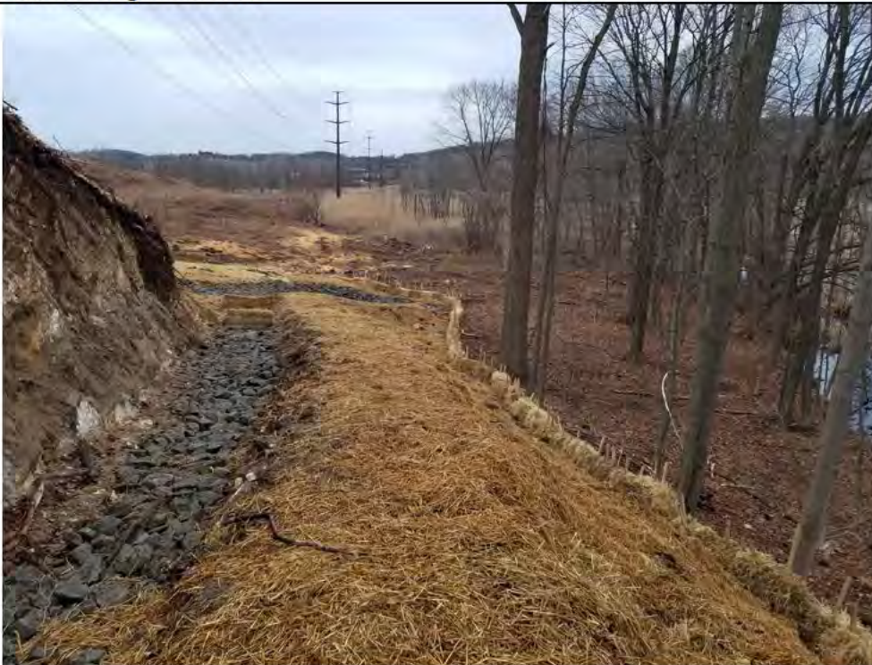
Photo 4: 02/22/2018, Danbury: Map 04, stone filled swale, mulch placement, and hay bales abutting Wetland W1 at bottom of slope east of Str1009, photo taken facing north towards Str1010.
