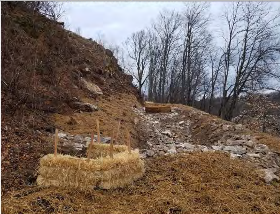
Photo 6: 02/22/2018, Danbury: Map 04, stone filled swale, mulch placement, and hay bales abutting Wetland W1 at bottom of slope southeast of Str1009, photo taken facing north towards Str1010.
