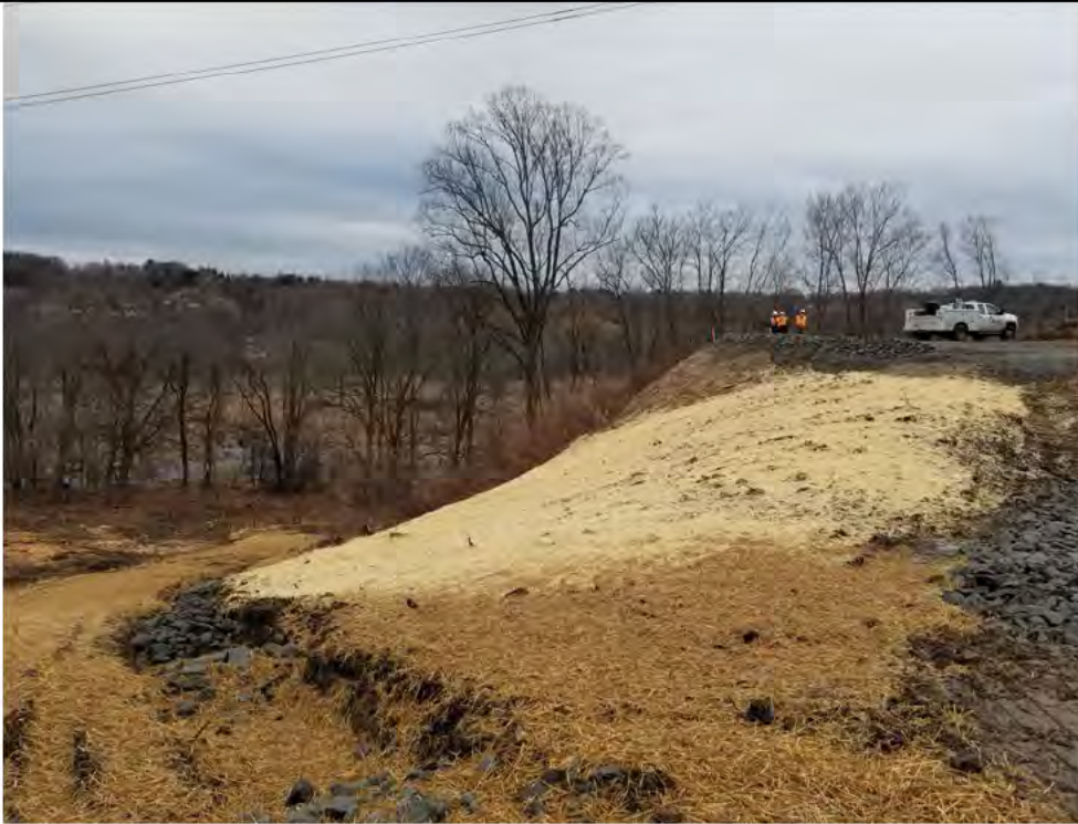
Photo 3: 02/22/2018, Danbury: Map 04, mulch placement for slope stabilization and stone filled swale at toe of slope for drainage, photo taken facing southeast.
