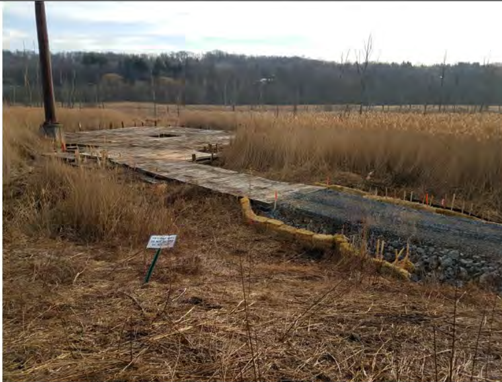
Photo 7: 03/01/2018, Danbury: Map 05, Str1010 pad completed, veg clearing completed and timber mats installed.
