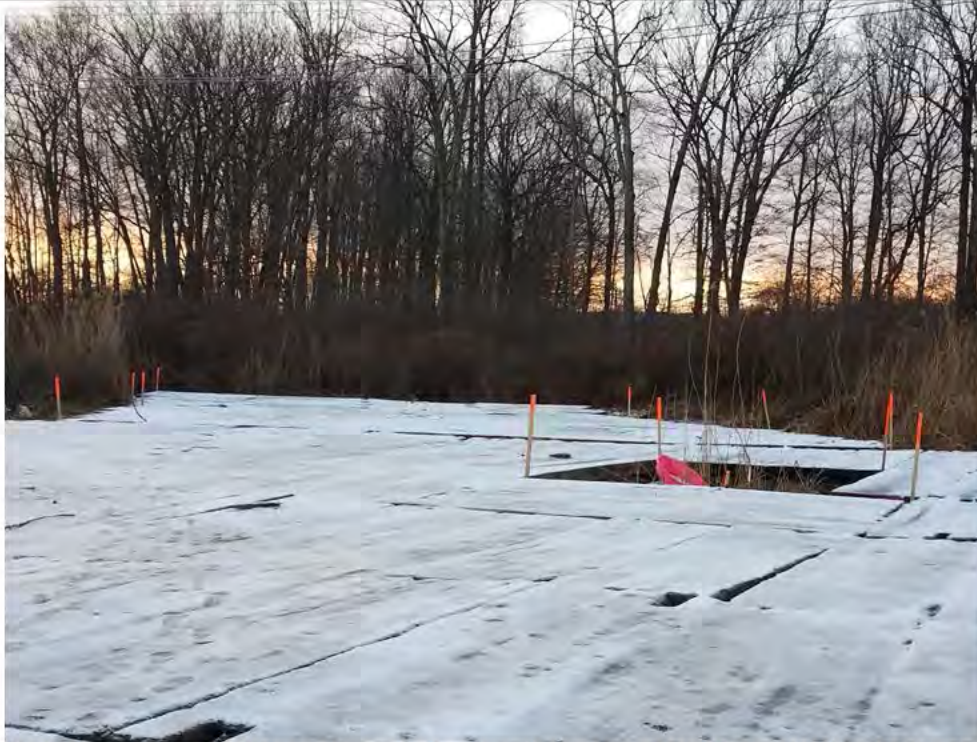
Photo 1: 02/08/2018, Bethel: Maps 01-02, south end of pull pad abutting Str1005 in Wetland W1, photo taken facing south.
