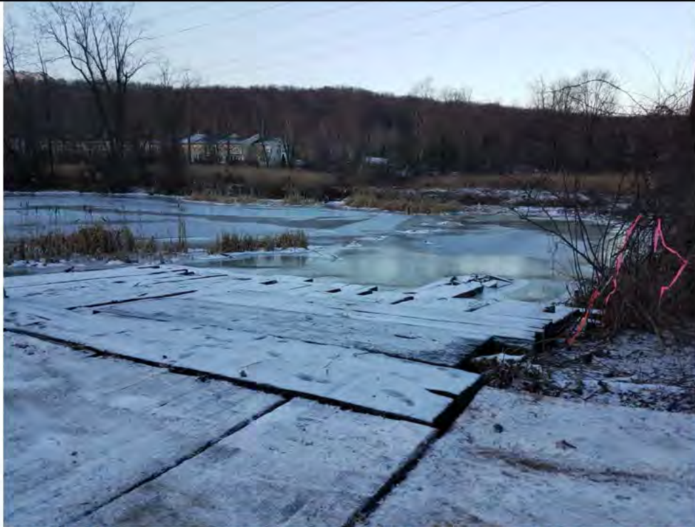
Photo 2: 02/08/2018, Bethel: Map 03, start of timber mat installation in Wetland W1 to access Str1007 to the west, photo facing west from the east access point off Shelter Rock Road.
