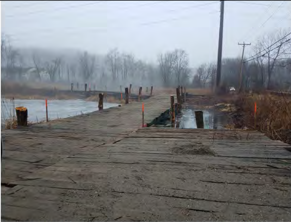
Photo 3: 02/15/2018, Bethel: Map 03, timber mat installation completed in Wetland W1 to access Str1007 to the west, photo facing west from the east access point off Shelter Rock Road.
