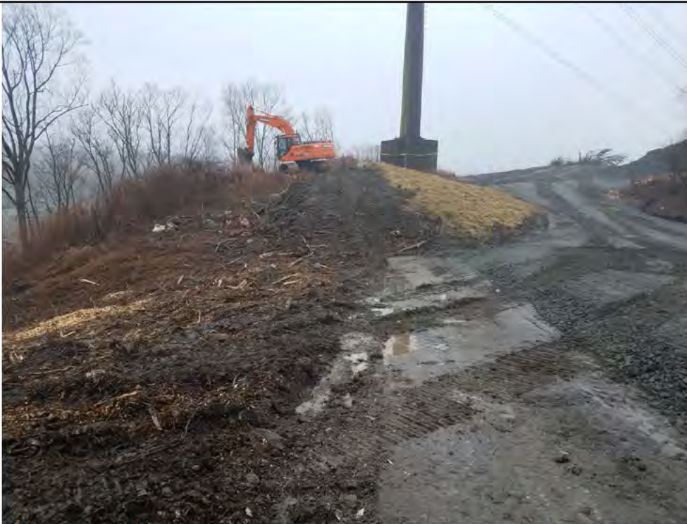
Photo 2: 02/15/2018, Danbury: Map 09, cutting grade and rough grading of pad at Str1009, photo taken facing southeast.
