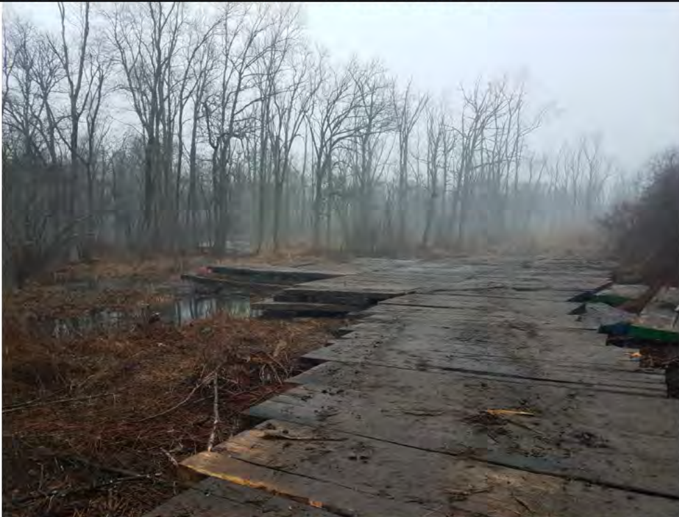
Photo 4: 02/15/2018, Danbury: Map 04, timber mat installation in progress in Wetland W1 at Str1008, Photo taken facing south toward Str1008.
