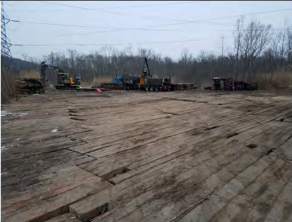
Photo 2: 01/11/2018, Bethel: Map 02, timber mat placement for structure pads 1000 through 1003. Working in Wetland W1.
