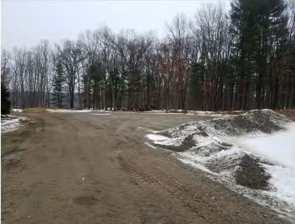
Photo 1: 01/11/18, Brookfield: Map 13, Str1025 pad construction in progress, awaiting placement of top course.
