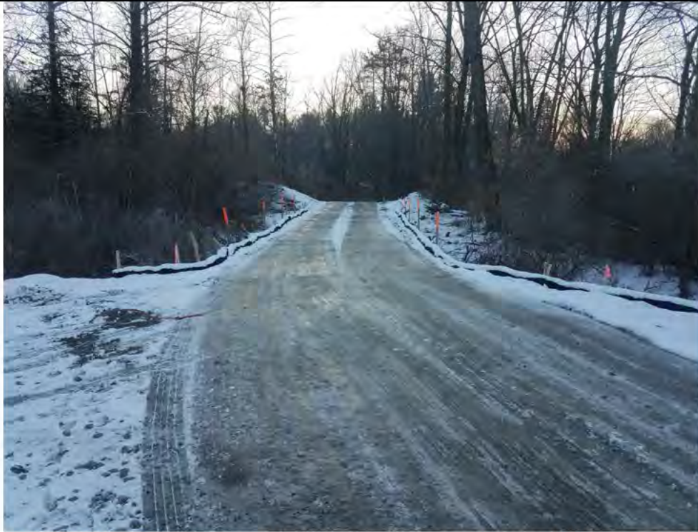
Photo 6: 01/18/2018, Bethel: Map 02, access road timber mat crossing to Plumtree Substation and structure pads 1000 through 1005 in Wetland W1.
