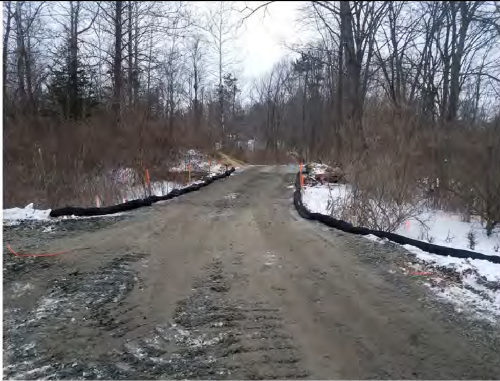
Photo 3: 01/11/2018, Bethel: Map 02, access road and timber mat crossing to Plumtree Substation and structures Str1000 through Str1003 and Wetland W1.
