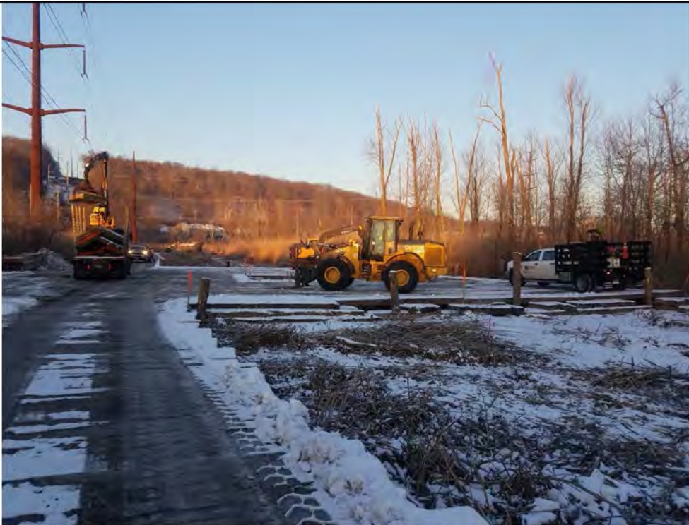
Photo 5: 01/18/2018, Bethel: Map 02, timber mat placement for structure pads 1004 through 1005. Working in Wetland W1.
