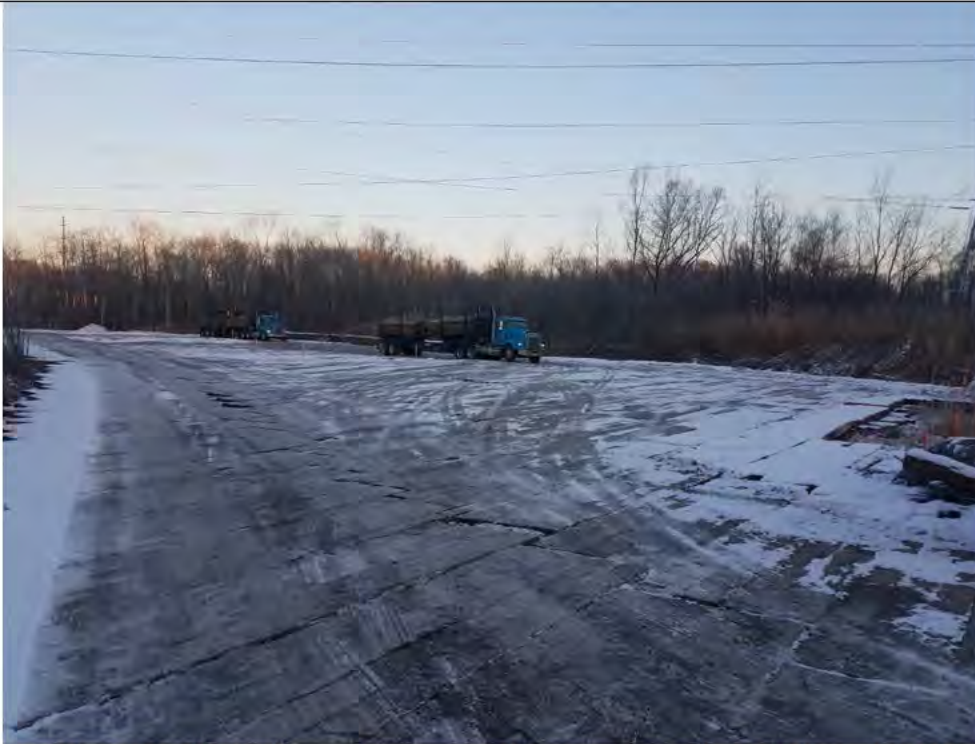
Photo 4: 01/18/2018, Bethel: Map 02, timber mat placement for structure pads 1000 through 1003. Working in Wetland W1.
