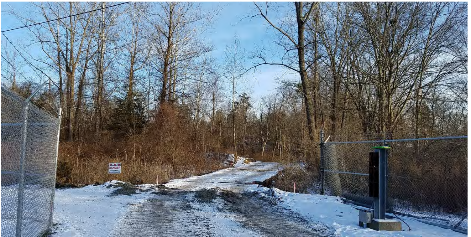
Photo #2: 1/3 – Between Plumtree Substation driveway and Plumtree Substation yard – Access route between the driveway and substation is cleared of trees. Uplands graded to a level surface and wetland crossing matted for tree clearing access. Facing southeast.
