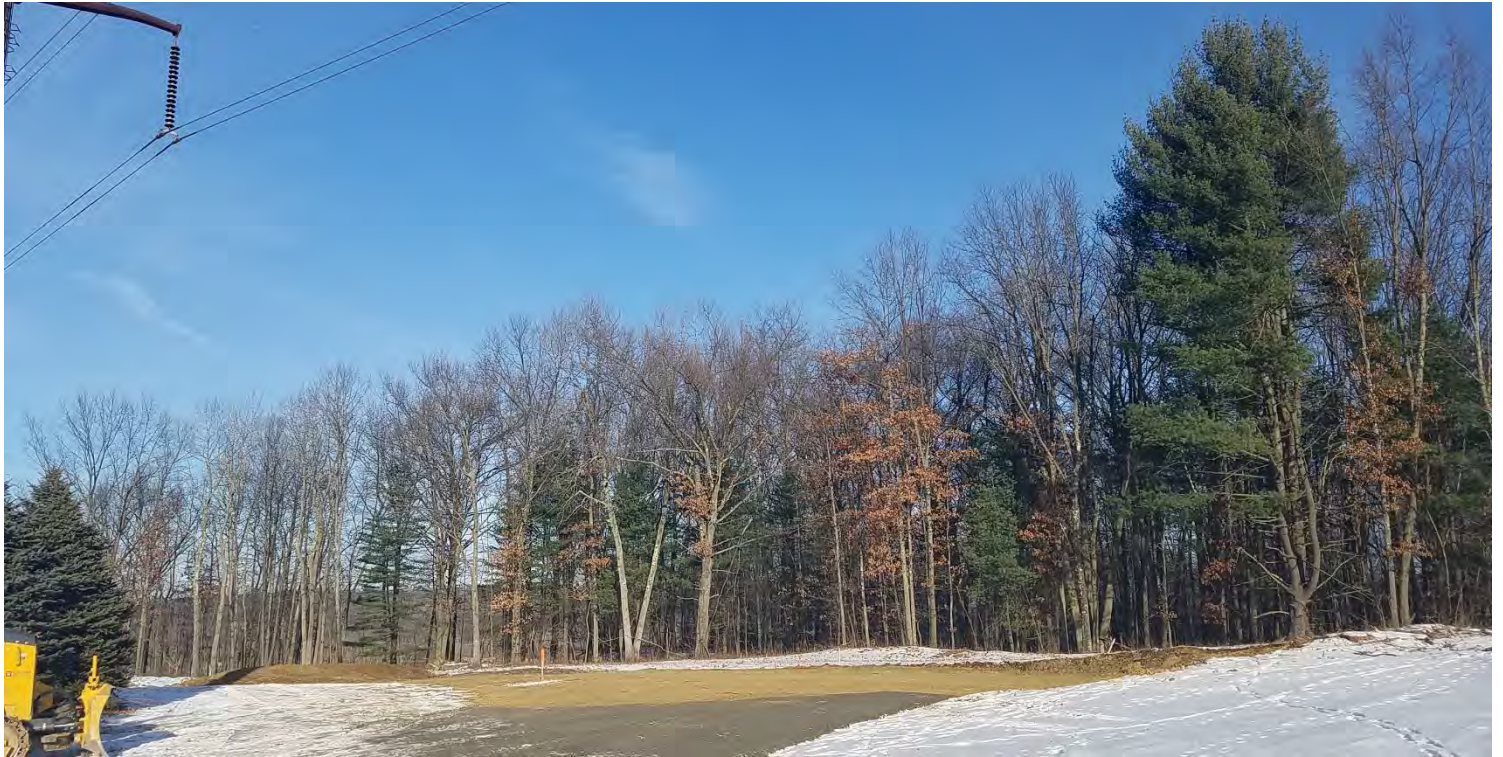
Photo #1: 1/3 – Structure 1025 north of Park Ridge Road – Grading of workpad for Structure 1025. Facing northeast.
