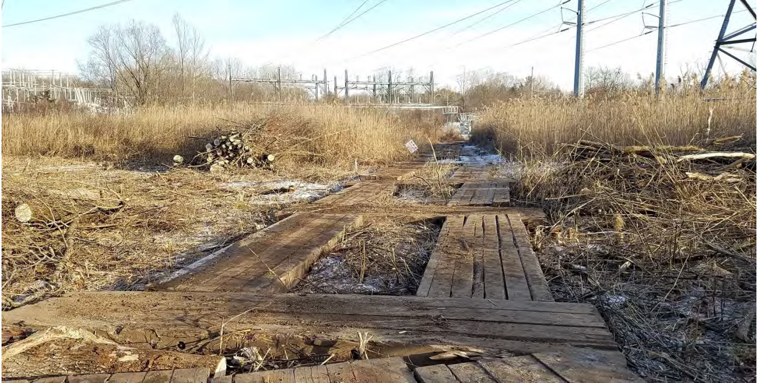
Photo #3: 1/3 – Near Structure 1003 west of Plumtree Substation – Temporary tree clearing access. Cleared brush and timber is temporarily staged within the permitted matted workpad footprints within Wetland W1. Staked locations of the limits of clearing were flagged with orange glow flagging prior the start of tree clearing in this area. Facing southeast.
