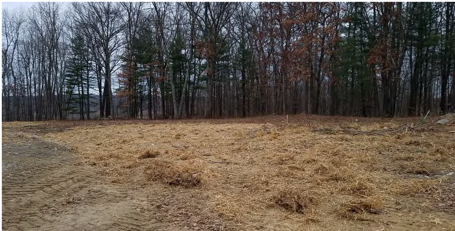
Photo #1: 12/22 – Between Park Ridge Road and Structure 1025 - Straw mulch applied over exposed soils post-tree clearing in the vicinity of Structure 1025. Facing northeast.
