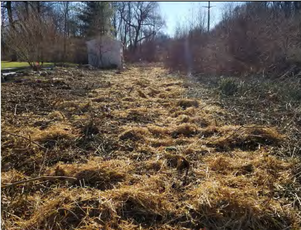
Photo 4: 12/21/17, Bethel: Map 8, vegetation and tree clearing area between Sky Edge Lane and Wetland W3, placement of straw mulch for stabilization and coverage of exposed soils.
