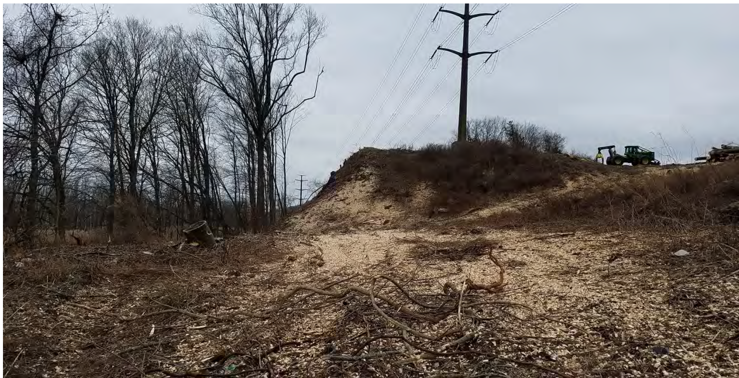
Photo #6: 12/22 – Near Structure 1009 - < 3” wood chip mulch applied for stabilization over exposed soils post-tree clearing. Facing South.
