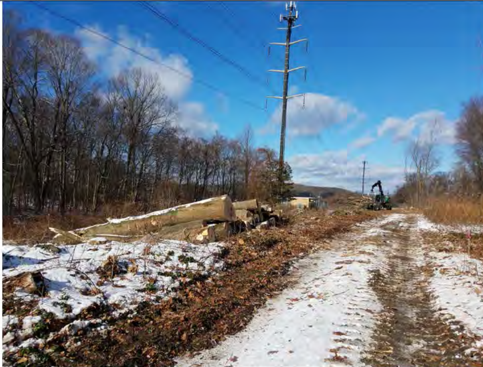
Photo 1: 12/14/2017, Bethel: Maps 8 and 9, clearing vegetation and trees between Sky Edge Lane and Str1017.
