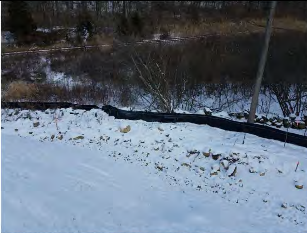
Photo 6: 12/14/17, CORRECTIVE ACTIONS: Brookfield, Exhibit 2B Vol 2 D&M Plan, Stony Hill Substation Expansion, Str4647A, and Wetland W7, northeast corner silt fence line, photo taken facing east, Repairs completed.
