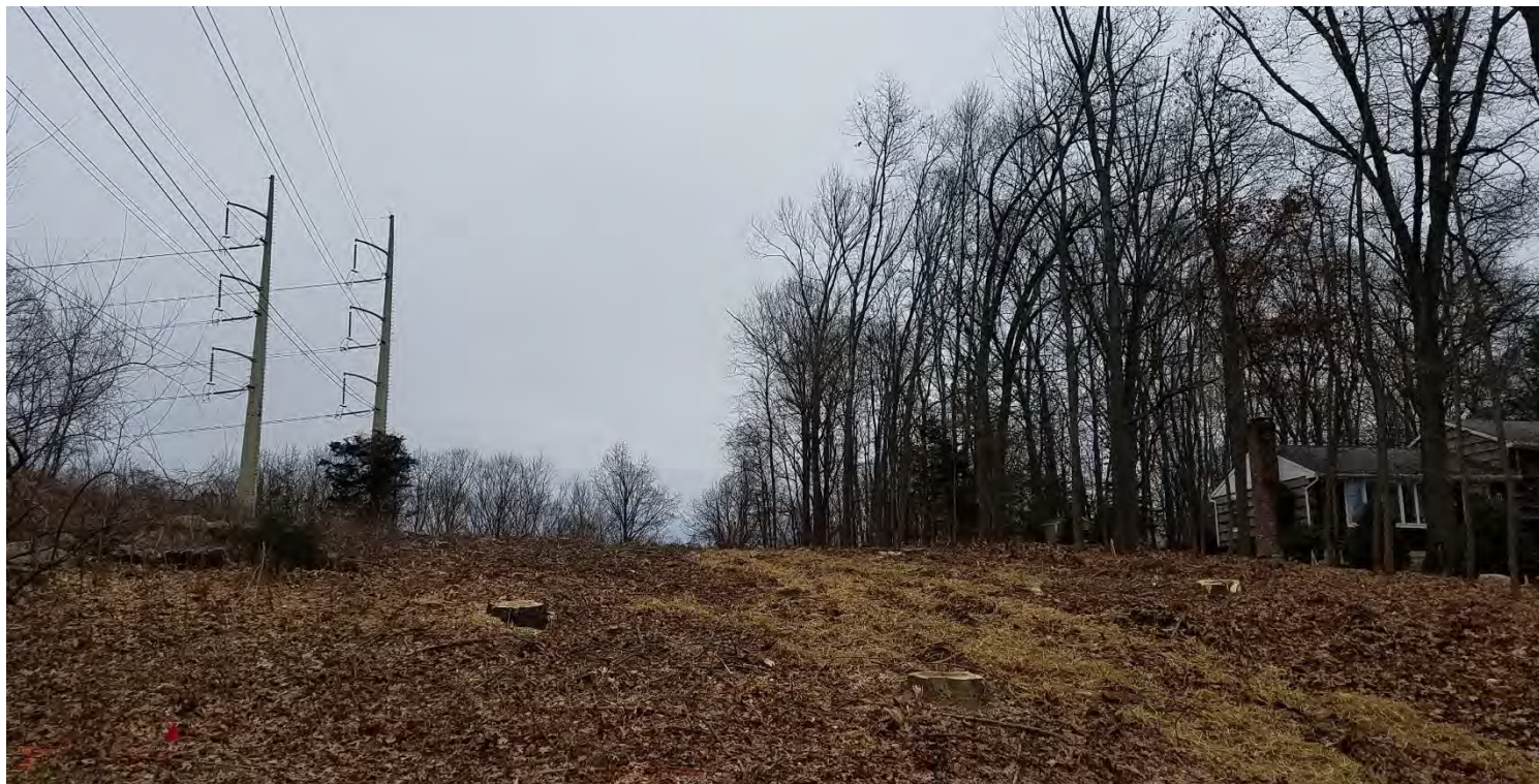
Photo #5: 12/22 – Between Hearthstone Drive and Structure 1015 - Straw mulch applied over exposed soils post-tree clearing. Facing east.
