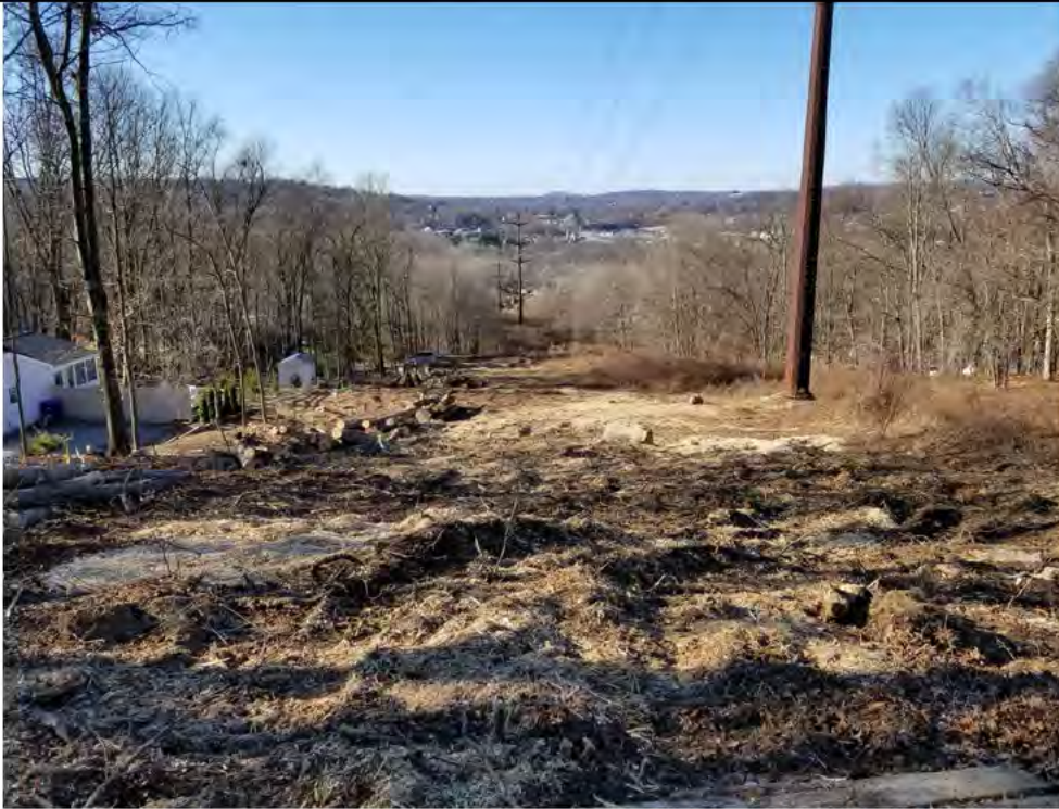
Photo 3: 12/21/17, Bethel: Map 7, vegetation and tree clearing area between Str1014 and Str1013, mixture of wood chips and straw mulch placed for stabilization and coverage of exposed soils.
