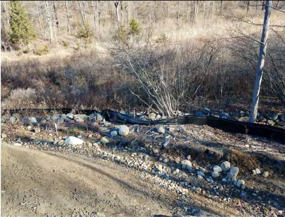
Photo 5: 12/07/17, Biweekly Report #5, Brookfield, Exhibit 2B Vol 2 D&M Plan, Stony Hill Substation Expansion, Str4647A, and Wetland W7, northeast corner silt fence line, photo taken facing east, in need of repairs.
