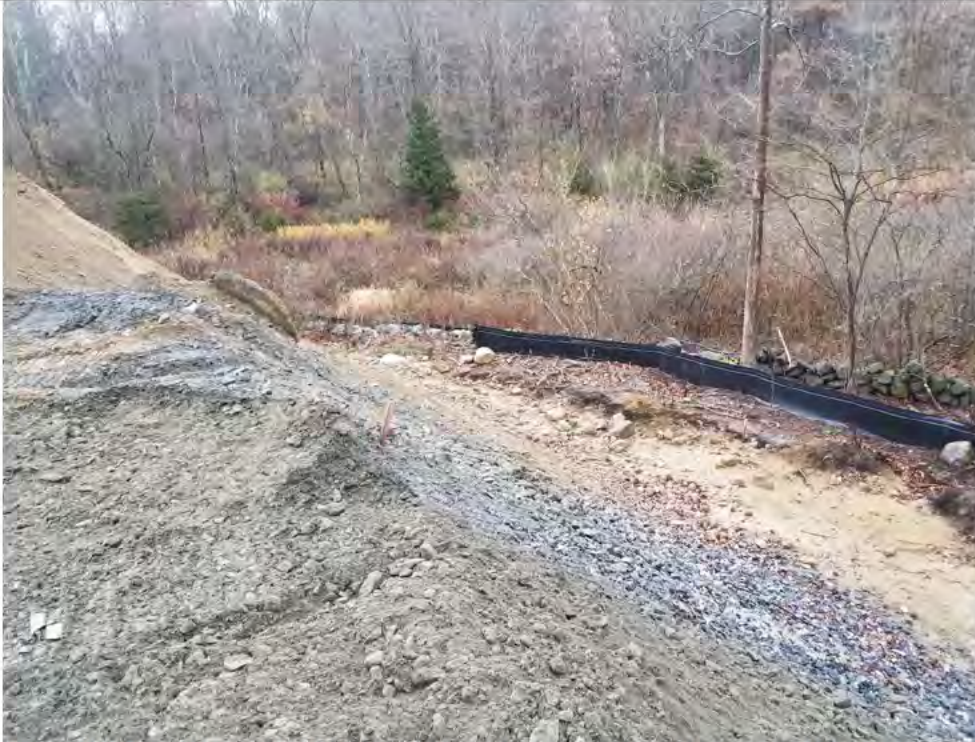
Photo 1: 11/16/17, Stony Hill Substation, Str4647A, silt fence line in northeast corner, W-7 north and east in this photo, photo taken facing north.
