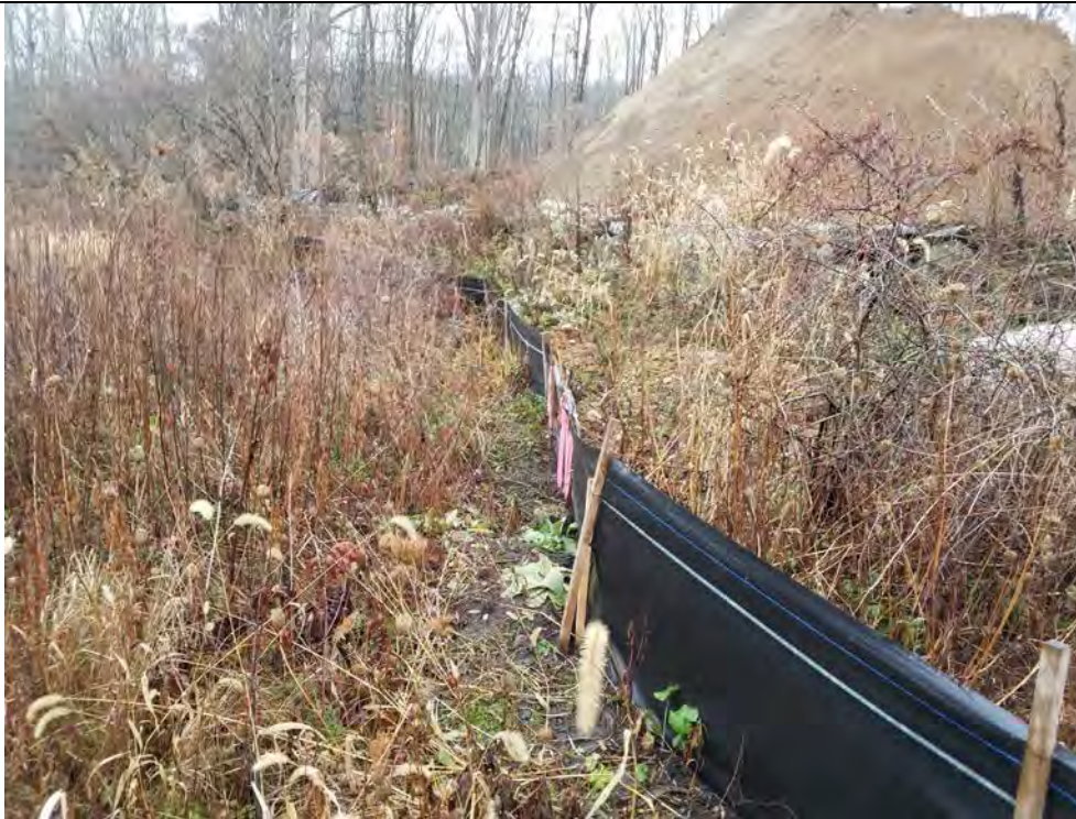
Photo 3: 11/22/17, Stony Hill Substation, Str4647A, silt fence line, east boundary, photo taken facing south. from the NE corner.
