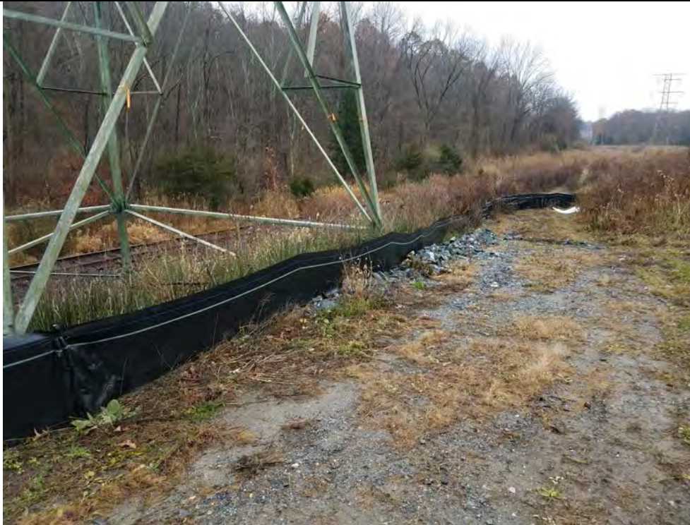
Photo 2: 11/22/17, Stony Hill Substation, Str4647A, silt fence line, north boundary, photo taken facing east.
