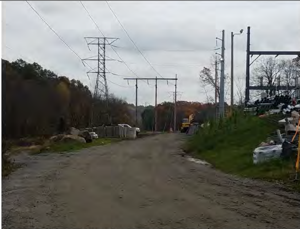
Photo 1: 11/02/17, Stony Hill Substation, Str4647A structures and lines, photo taken facing east.
