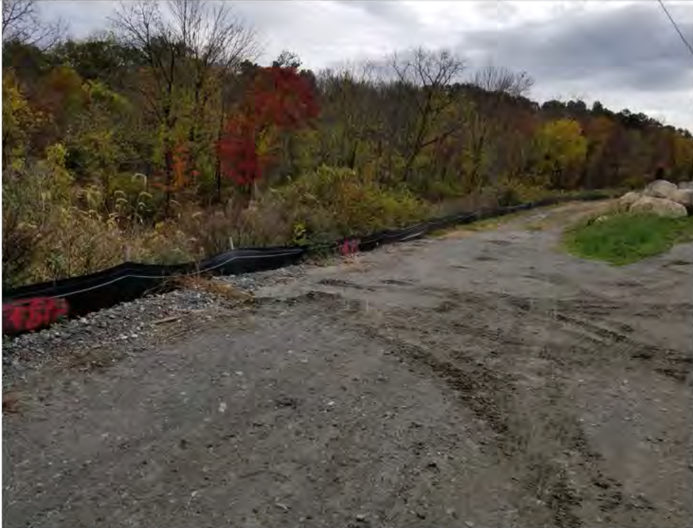
Photo 3: 10/26/17: Stony Hill Substation, Str4647A and substation work area perimeter silt fencing, photo taken facing east.
