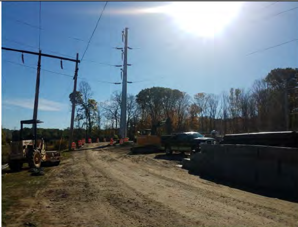
Photo 2: 10/19/17, Stony Hill Substation, Str4647A structures and lines, photo taken facing east.
