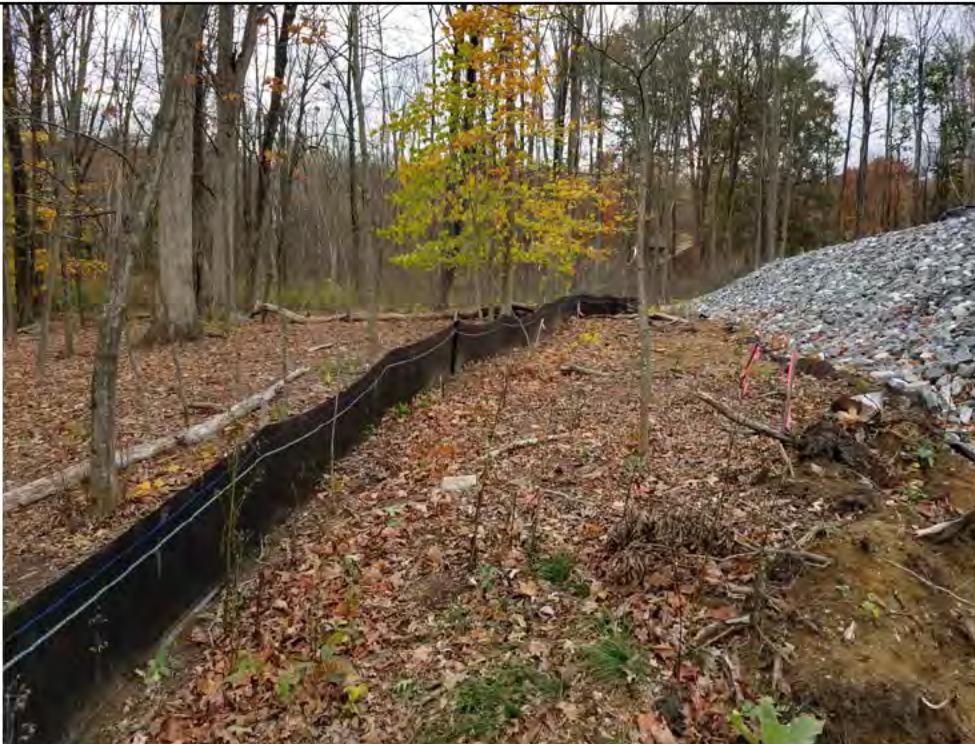
Photo 6:10/26/17: Stony Hill Substation, Str4647A and substation work area perimeter silt fencing, photo taken facing south.
