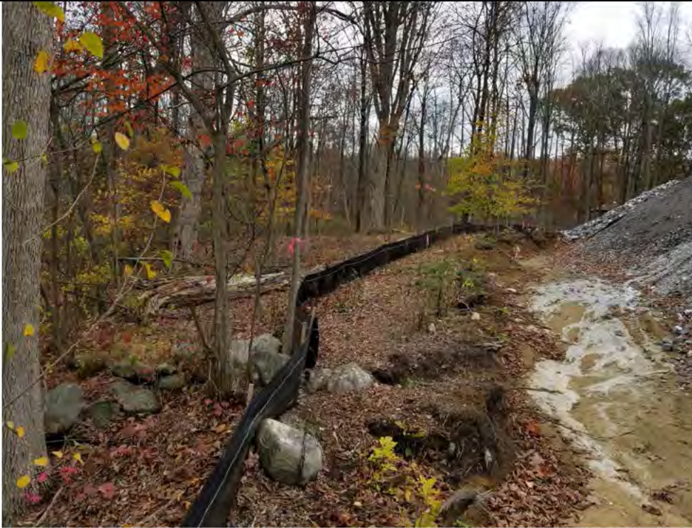
Photo 5:10/26/17: Stony Hill Substation, Str4647A and substation work area perimeter silt fencing, photo taken facing south.
