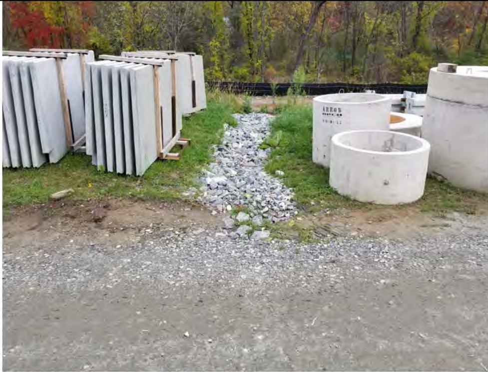
Photo 7:10/26/17: Stony Hill Substation, Str4647A and substation access road drainage, photo taken facing north.
