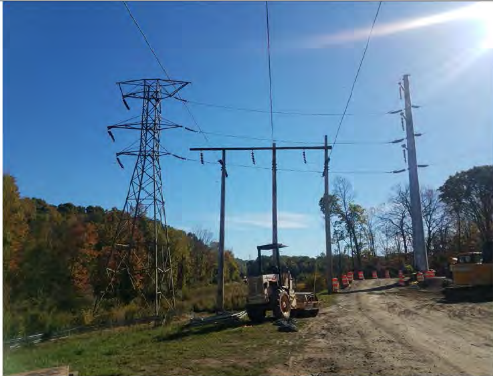
Photo 1: 10/19/17, Stony Hill Substation, Str4647A structures and lines, photo taken facing east.
