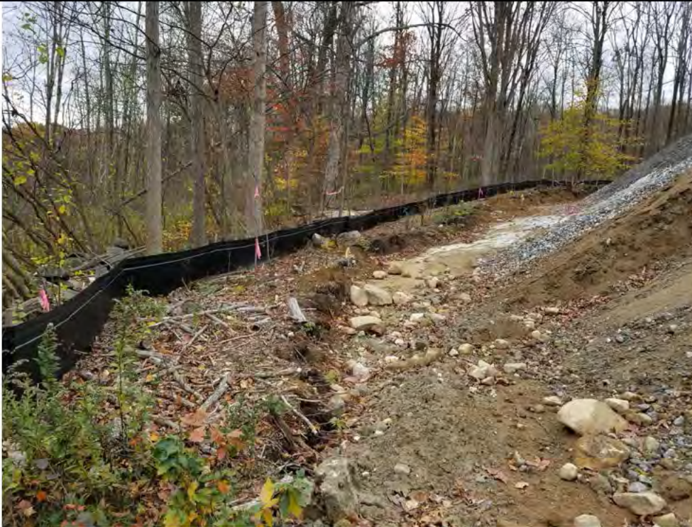
Photo 4: 10/26/17: Stony Hill Substation, Str4647A and substation work area perimeter silt fencing, photo taken facing south.
