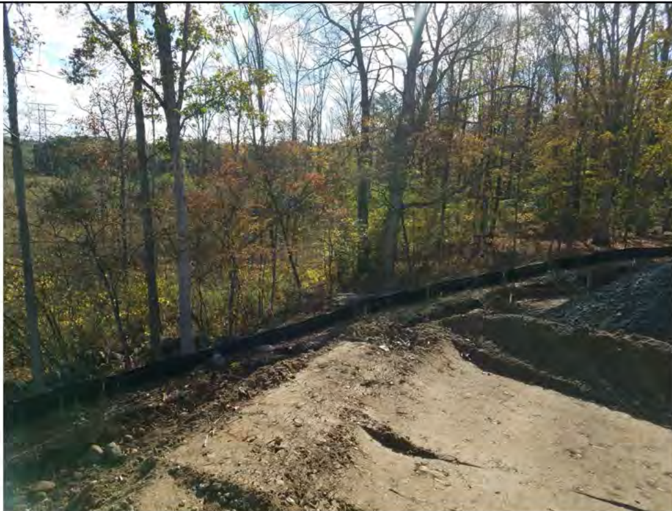
Photo 4: 10/12/17: Stony Hill Substation, silt fencing placement, photo taken facing west in the area of wetland W7.
