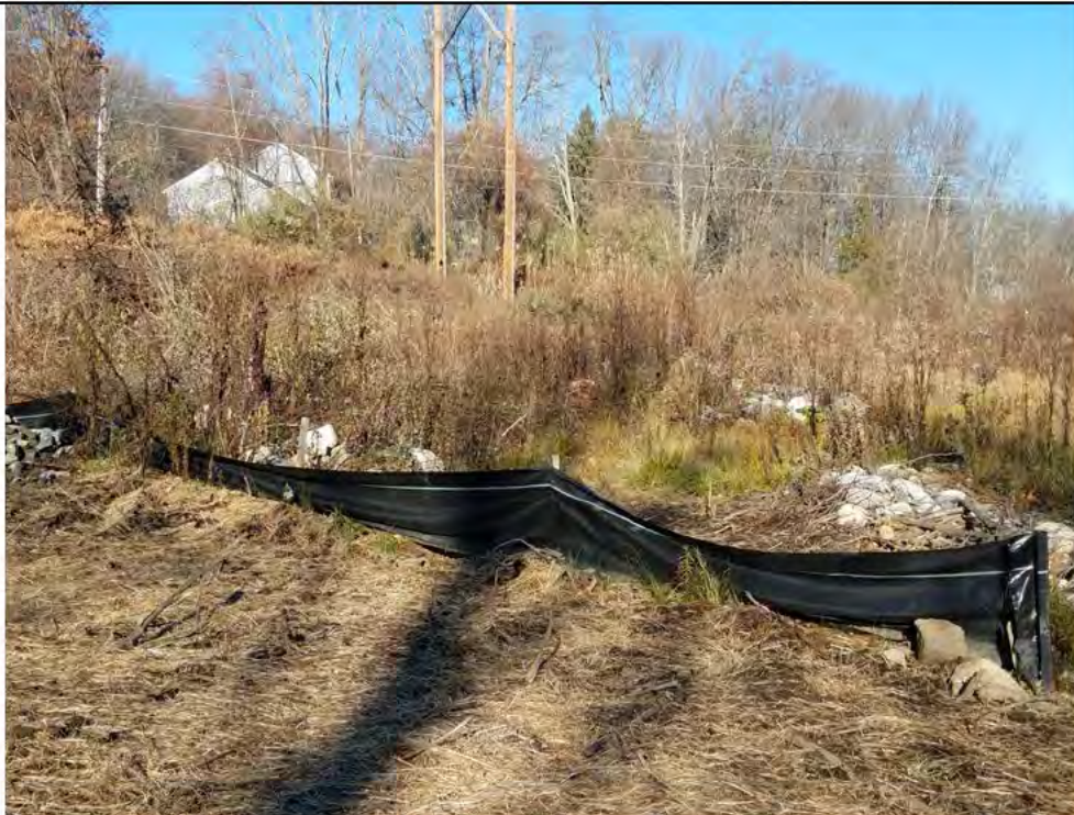
Photo 4: 11/24/17, Thomaston: Map 22, Str62 at W-D10, silt fence repairs required.
