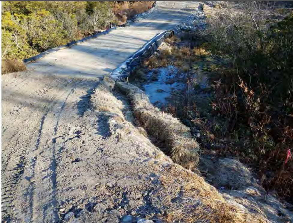
Photo 6: 11/24/17, Watertown: Map 14, CORRECTIVE ACTION-New hay bales and blown hay at W-C20.
