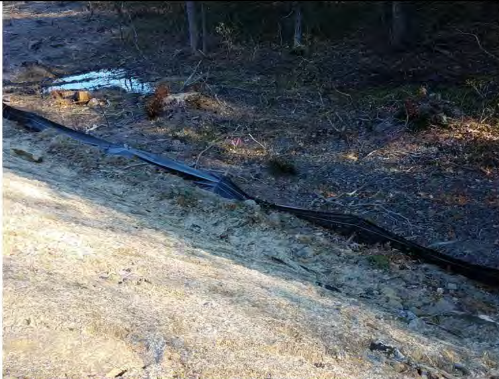
Photo 3: 11/24/17, Watertown: Map 14, Str39 at W-C20/VP-20-1, silt fence repairs required.
