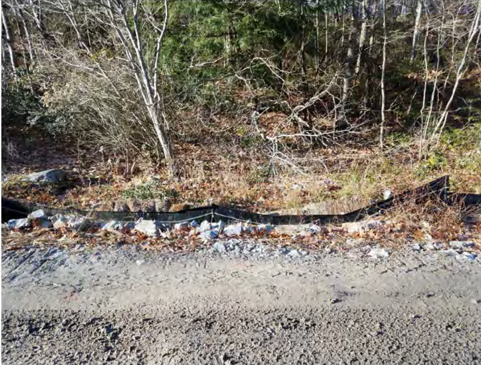
Photo 2: 11/24/17, Watertown: Map 12, W-C14 silt fence repairs required.
