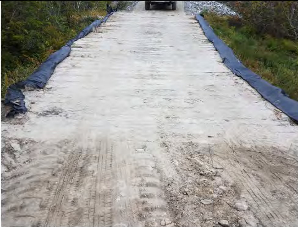
Photo 1: 10/06/17 , Watertown: Map 14, Wetland W-C20 timber mat crossing, sediment buildup on mats. Photo taken from Biweekly Report #22 showing existing sediment buildup and dry conditions.
