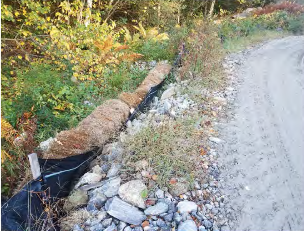
Photo 2: 10/13/17, Watertown: General conditions of many sections of silt fence and straw bales alongside of access roads of the ROW. Road base stone and riprap have pushed outward overloading the structural integrity of the E&S controls and many times tearing the fabric and allowing sediments to pass through.
