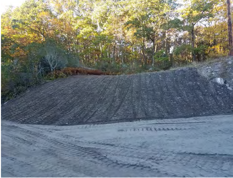
Photo 5: 10/20/17, Watertown: Maps 09-16, Str24-Str46, upland slope grading and preparing for seeding for restoration.
