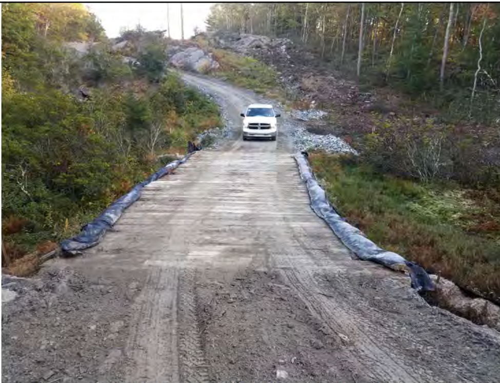
Photo 1-1: 10/13/17 , Watertown: Map 14, CORRECTIVE ACTION -Wetland W-C20 timber mat crossing, sediment buildup cleared, some recent minor buildup however hard-packed into the crevices of the timbers.
