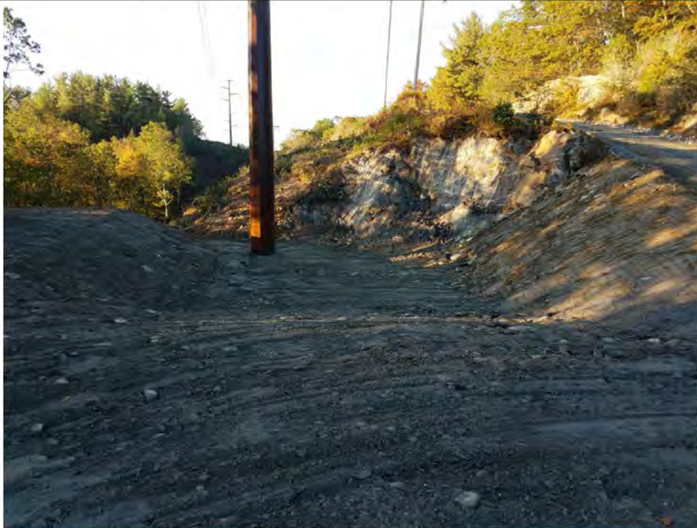
Photo 4: 10/13/17, Watertown: Map 15, Str42 partial restoration, grading and preparing for seeding and slope stabilization.
