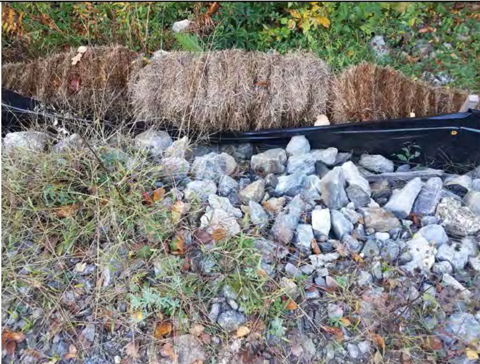
Photo 3: 10/13/17, Watertown: General conditions of many sections of silt fence and straw bales alongside of access roads of the ROW. Road base stone and riprap have pushed outward overloading the structural integrity of the E&S controls and many times tearing the fabric and allowing sediments to pass through.
