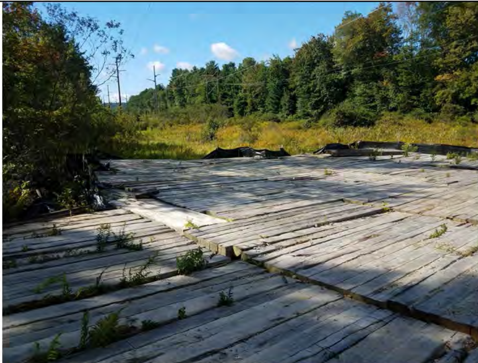
Photo 6: 10/06/2017, Harwinton: Map 35, Str95 perimeter fencing to prevent turtle access in poor condition.
