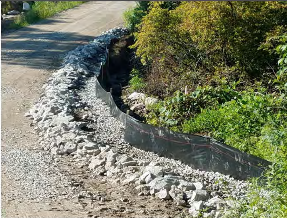
Photo 6: 07/21/2017, Watertown: Map 10, area of W-C3, access road at Str27, E&S control repair/improvements.
