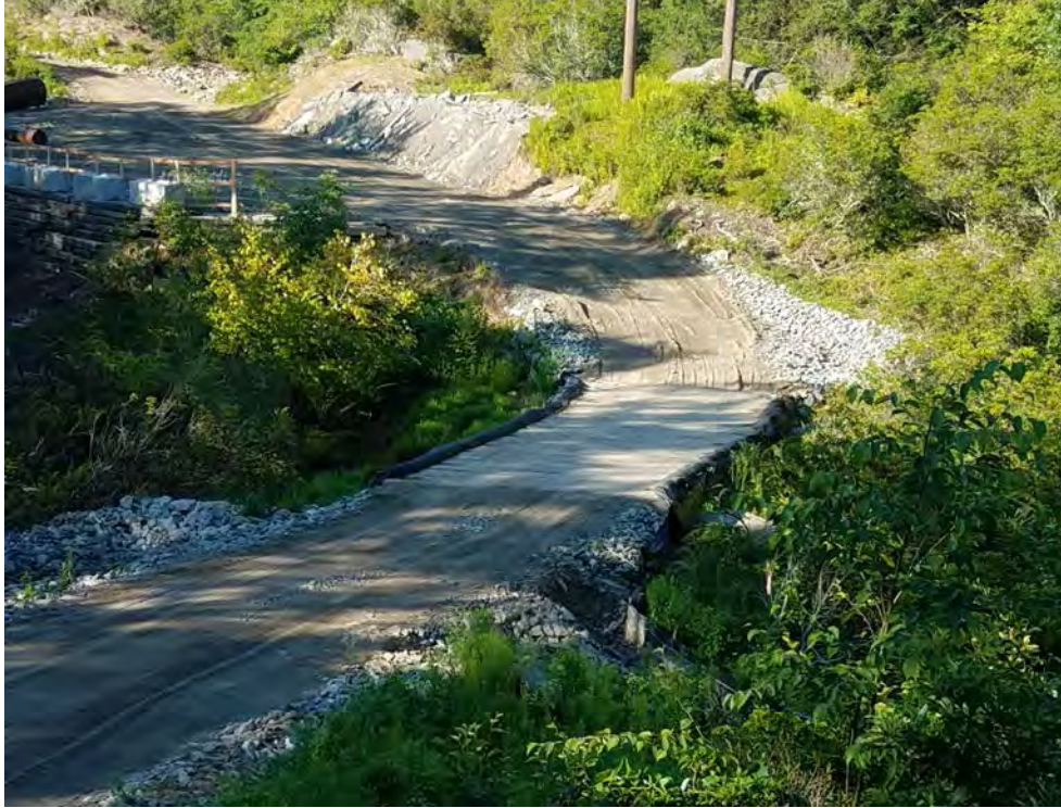
Photo 1: 07/21/2017, Watertown: Map 14, timber mat crossing at W-C20, timber mats cleared and E&S control repairs/improvements, sediment impacts cleared by hand to the waterline.
