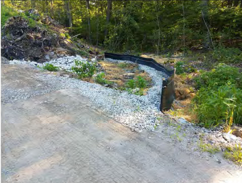
Photo 5: 07/21/2017, Watertown: Map 11, area of Str30 at W-C7, access road at Str30, repairs to E&S controls.
