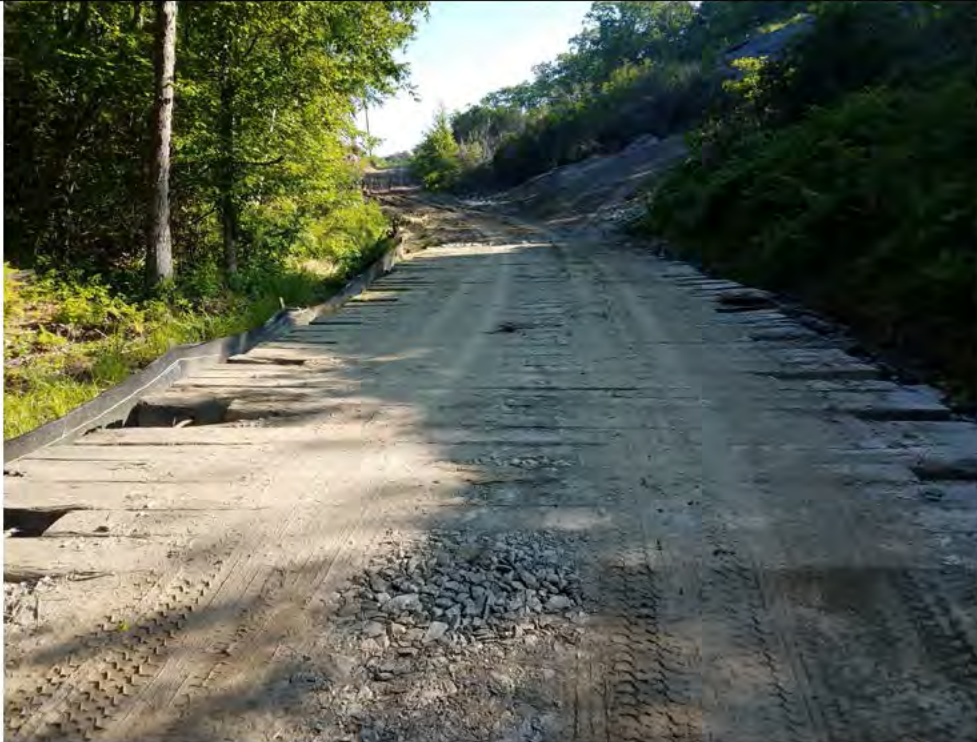
Photo 3: 07/21/2017, Watertown: Map 12, timber mat crossing at W-C15, timber mats cleared, E&S control repairs.
