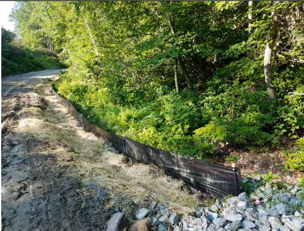
Photo 2: 07/21/2017, Watertown: Map 13, access road at W-C18, E&S control repair.
