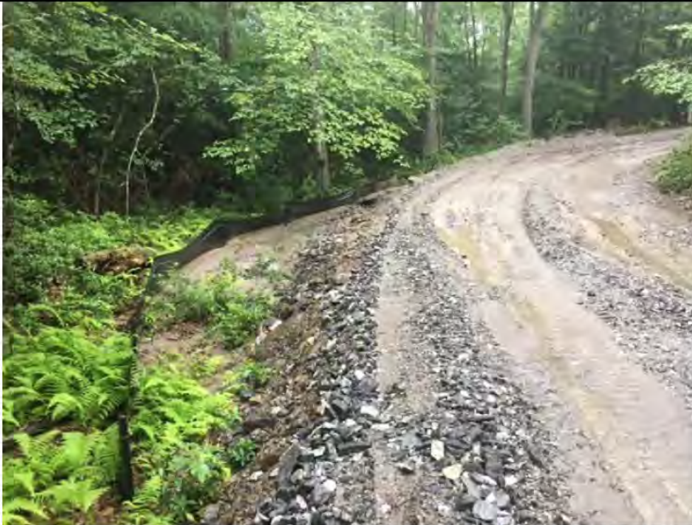
Photo 7: 07/07/2017, Watertown: Access road to Str42, excess sediment buildup and silt fence failure, sedimentation into wooded area.
