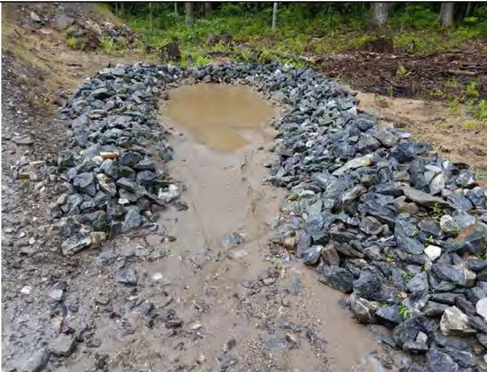
Photo 12: 07/07/2017, Watertown: Access road to Str37 at W-C7, excessive sediment buildup in temporary sediment trap, minor break through and sedimentation, not into W-C7.
