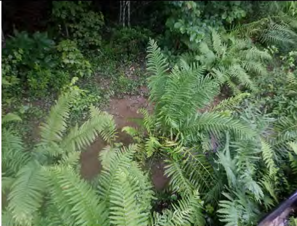
Photo 15: 07/07/2017, Watertown: Access road at W-C18, surface water runoff, excessive sediment buildup on silt fence, silt fence failure, sedimentation into W-C18.
