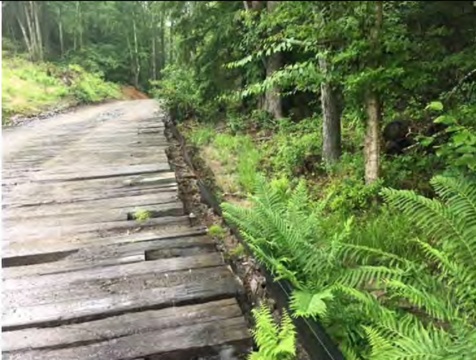
Photo 16: 07/07/2017, Watertown: Access road at W-C18, surface water runoff, excessive sediment buildup on silt fence, silt fence failure, sedimentation into W-C18.
