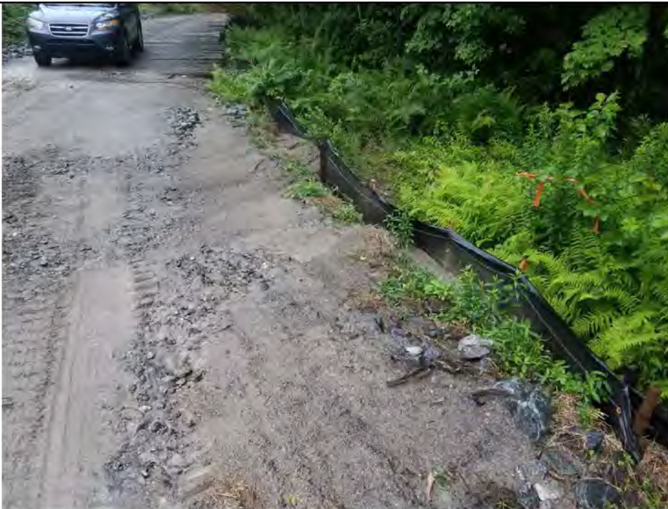
Photo 14: 07/07/2017, Watertown: Access road at W-C18, surface water runoff, excessive sediment buildup on silt fence, silt fence failure, sedimentation into W-C18.
