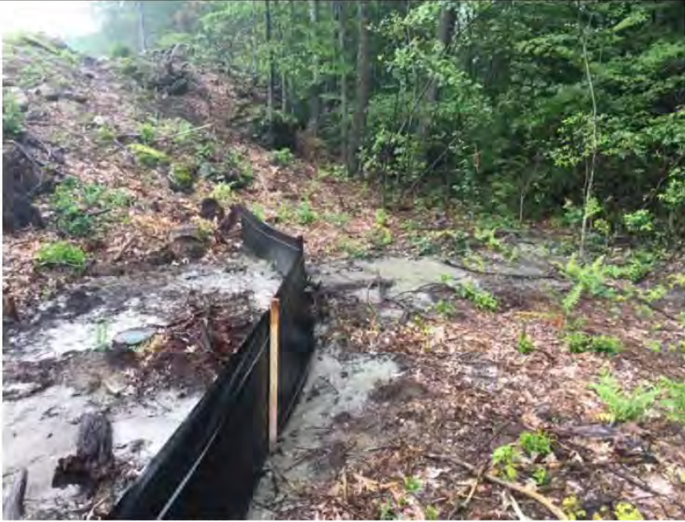
Photo 1: 07/07/2017, Watertown: Area of Str30 at W-C7, silt fence failure.
