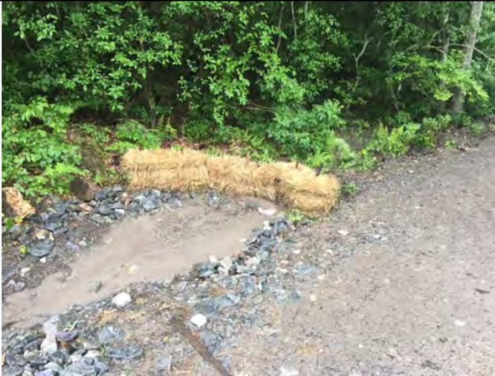
Photo 3: 07/07/2017, Watertown: Area of Str36, temporary sedimentation trap, excess sediment buildup.
