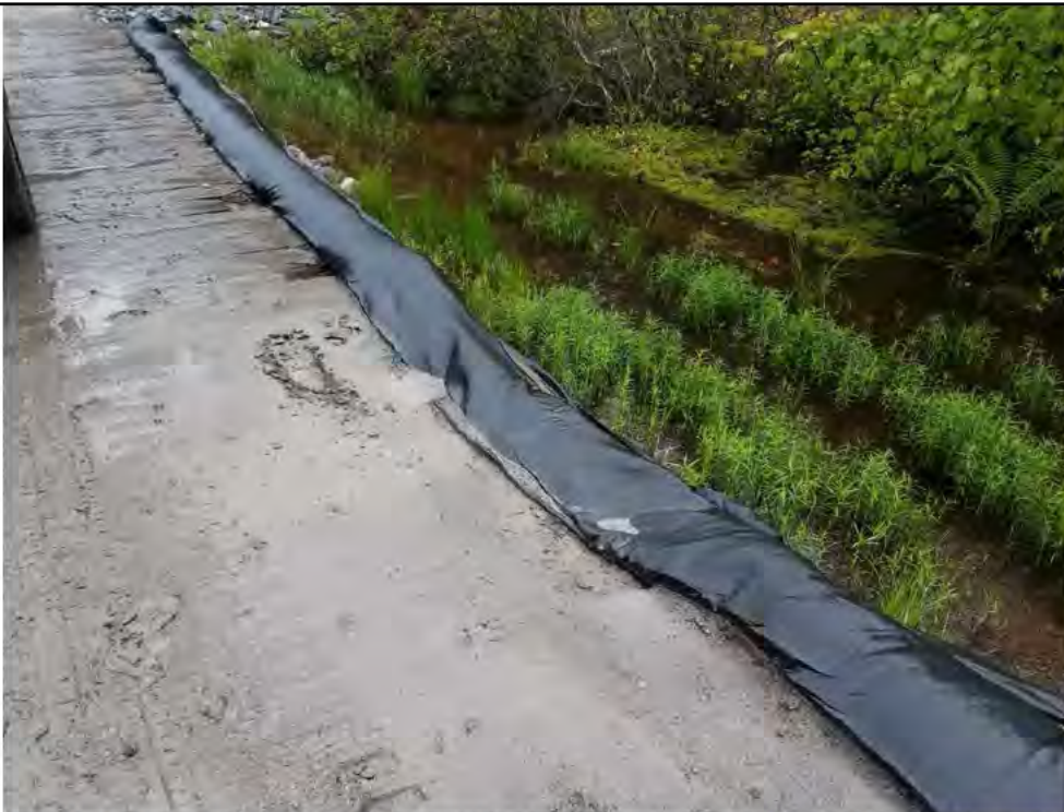
Photo 18: 07/07/2017, Watertown: Access road at W-C20, surface water runoff, excessive sediment buildup on timber mats, sedimentation into W-C20.
