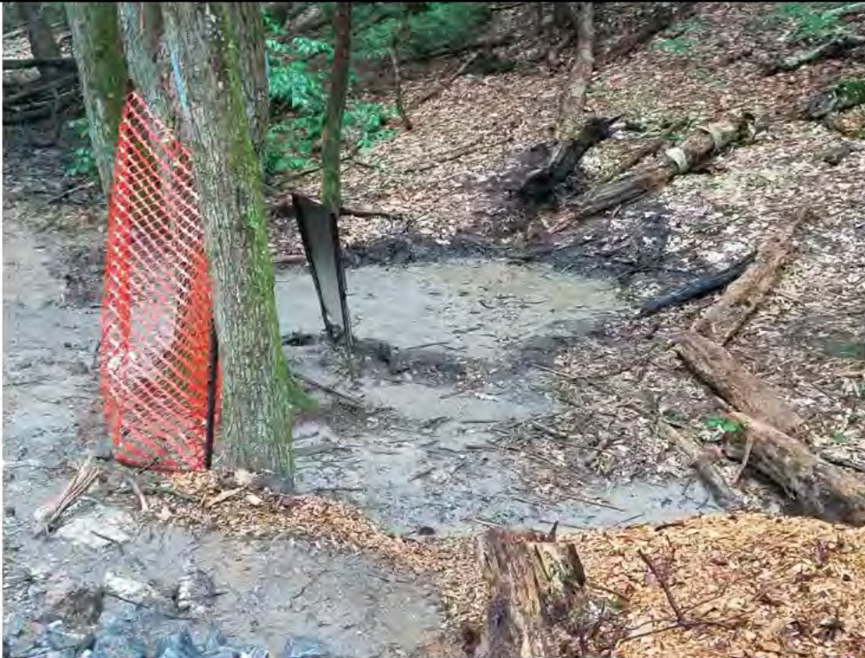
Photo 11: 07/07/2017, Watertown: Access road to Str45, surface water runoff, sedimentation into wooded area and designated CT State hiking trail access point.
