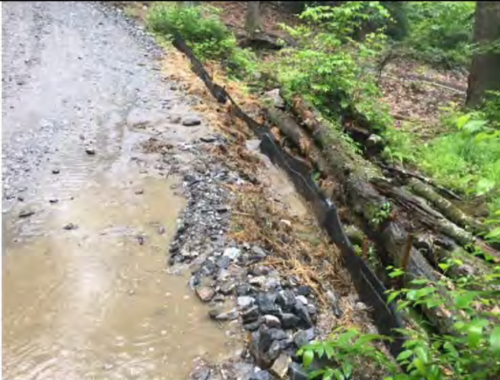
Photo 9: 07/07/2017, Watertown: Access road to Str45, excess sediment buildup and silt fence failure.
