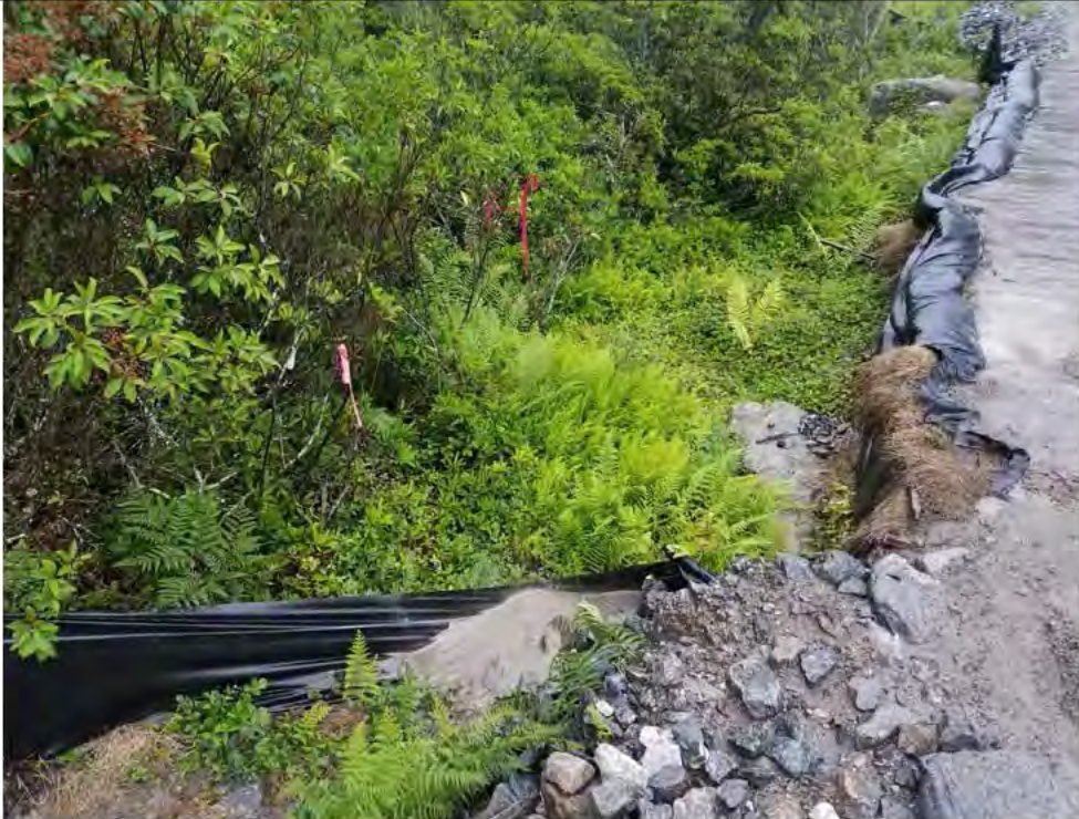
Photo 17: 07/07/2017, Watertown: Access road at W-C20, surface water runoff, excessive sediment buildup on silt fence, silt fence failure, sedimentation into W-C20.
