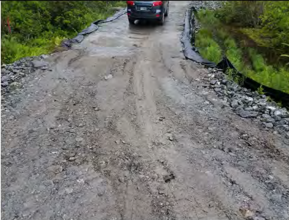
Photo 19: 07/07/2017, Watertown: Access road at W-C20, surface water runoff, excessive sediment buildup on silt fence, silt fence failure, sedimentation into W-C20.
