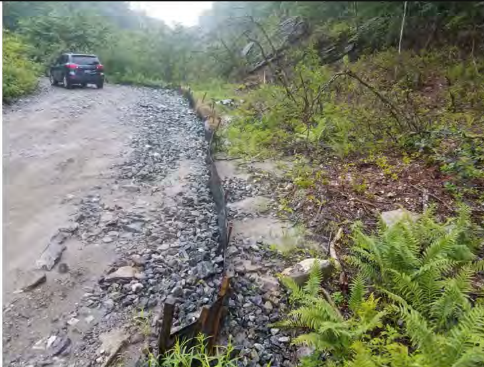
Photo 2: 07/07/2017, Watertown: Area of Str34 at W-C15, silt fence failure.
