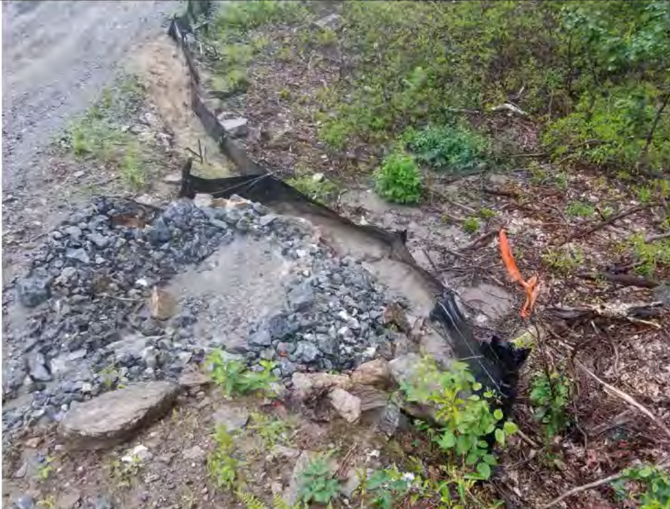
Photo 13: 07/07/2017, Watertown: Access road at W-C15, surface water runoff, improperly sized/constructed sedimentation trap. Silt fence failure, sedimentation into W-C15.
