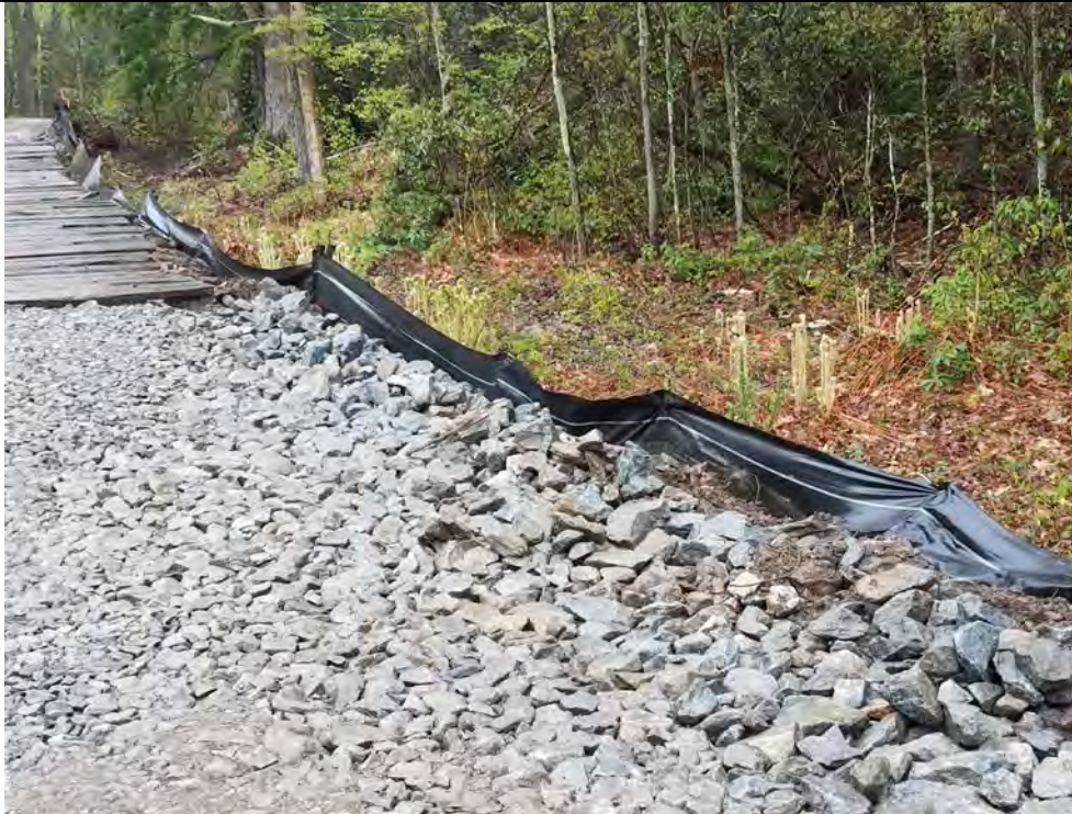
Photo 6: 05/05/2017, Watertown: Map 13, E&S repairs needed in area of wetland W-C18.
