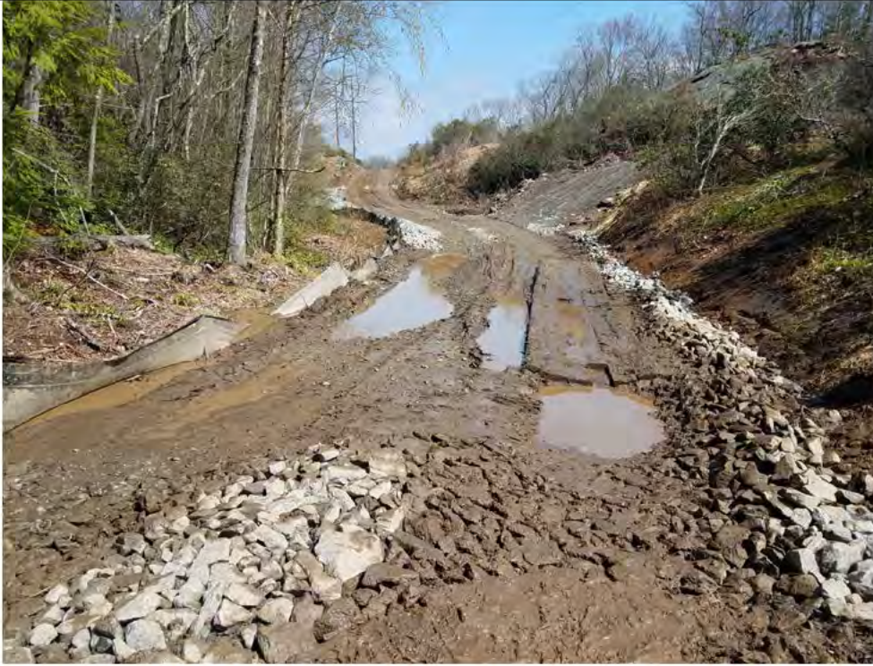
Photo 1: 4/28/2017, Watertown: Map 13, Wetland W-C18 impacts, ponding, rutting, failed E&S controls.
