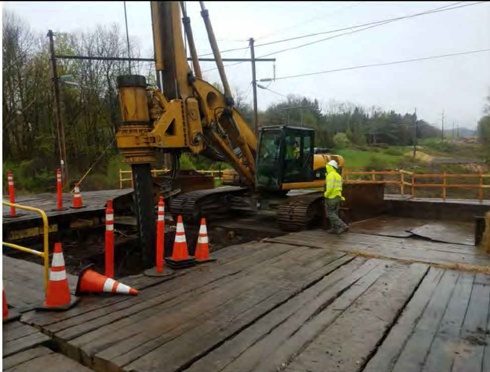
Photo 9: 05/05/2017, Thomaston: Map 22, PAR drilling to install a drilled shaft vertical deadend steel structure.
