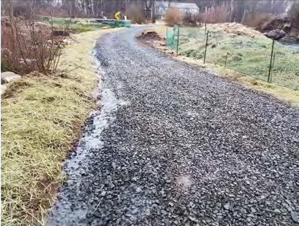
Photo 5: 3/31/2017, Litchfield: Maps 28 & 29, access road to Str80 abutting private driveway, repairs made to driveway after surface water runoff erosion was reported by property owner.
