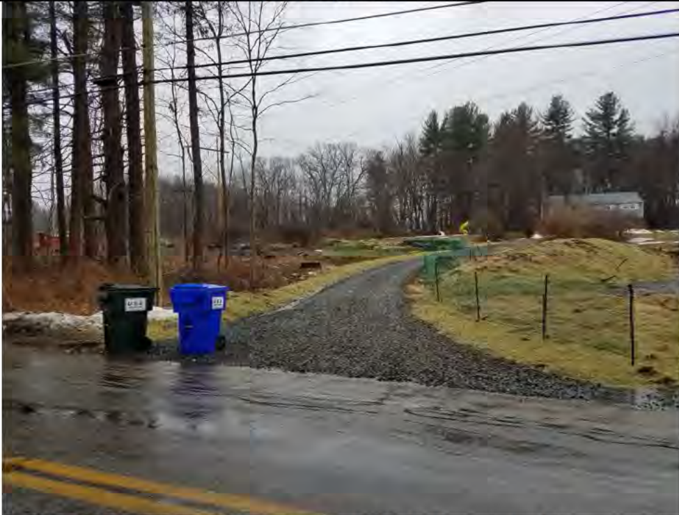
Photo 6: 3/31/2017, Litchfield: Maps 28 & 29, access road to Str80 abutting private driveway, repairs made to driveway after surface water runoff erosion was reported by property owner.
