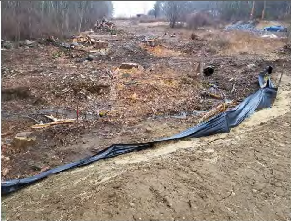
Photo 10: 3/31/2017, Litchfield: Map 29, Str83 abutting W-F4 and S-F2, failing E&S.
