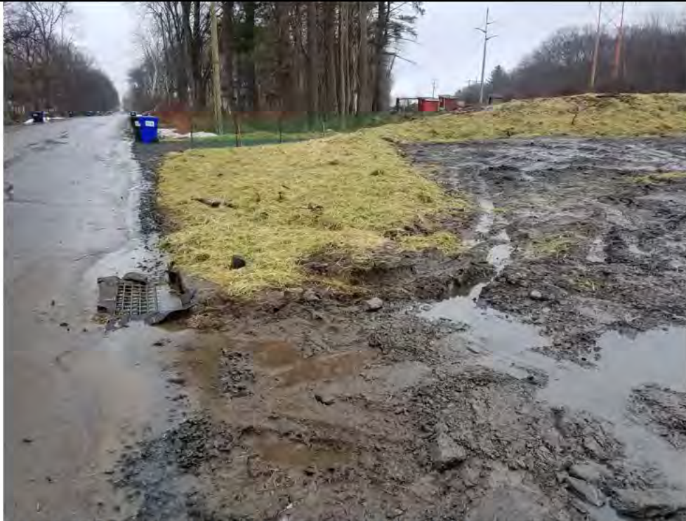
Photo 7: 3/31/2017, Litchfield: Map 29, Str81 abutting Campville Road, E&S, tracking pad, and catch basin protection needed. Corrections were reportedly made on this day after the time of this inspection.
