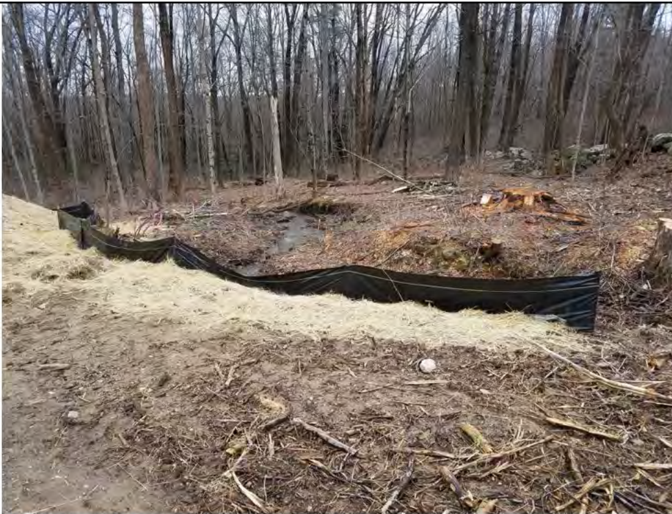
Photo 20: 04/07/2017, Litchfield: Map 29, E&S controls at Str83.
