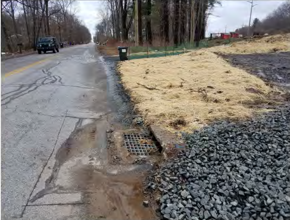
Photo 19: 04/07/2015, Litchfield: Map 29, between ROW access road to Str80 (Southard property) and street access to Str81, E&S controls and catch basin drainage protection measures.
