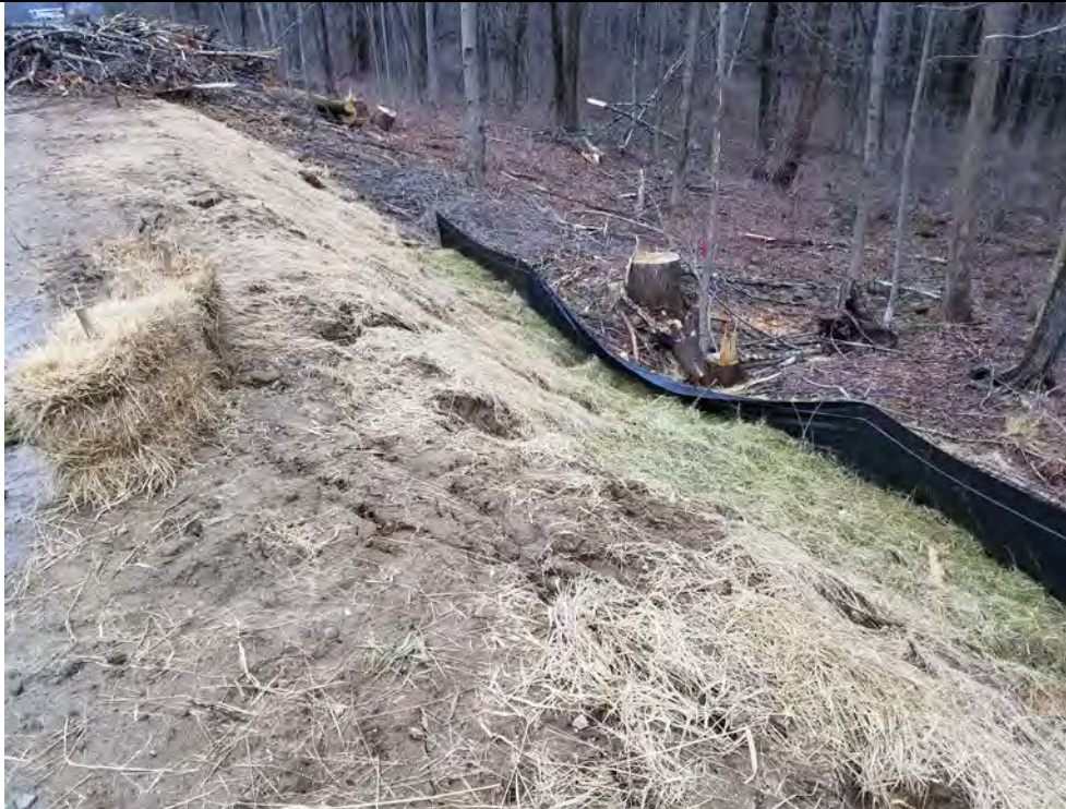
Photo 22: 04/07/2017, Litchfield: Map 29, E&S controls at Str83, erosion of slope material.
