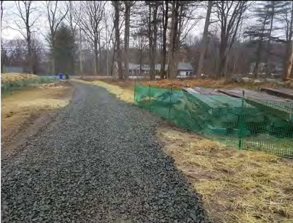
Photo 3: 3/31/2017, Litchfield: Maps 28 & 29, access road to Str80 abutting private driveway, repairs made to driveway after surface water runoff erosion was reported by property owner.
