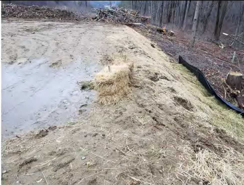
Photo 23: 04/07/2017, Litchfield: Map 29, E&S controls at Str83, ponding on top of pad and runoff causing rills to form.
