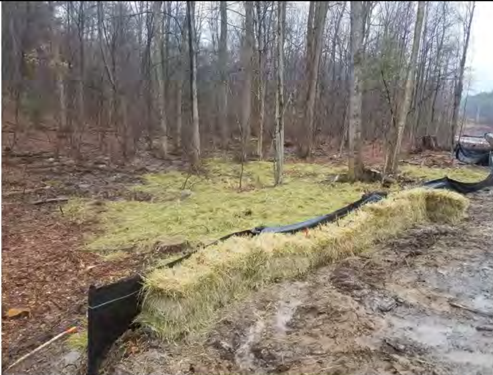
Photo 13: 3/31/2017, Harwinton: Map 35, Str96 abutting W-G1, restoration and installation of E&S, post wetland impact.
