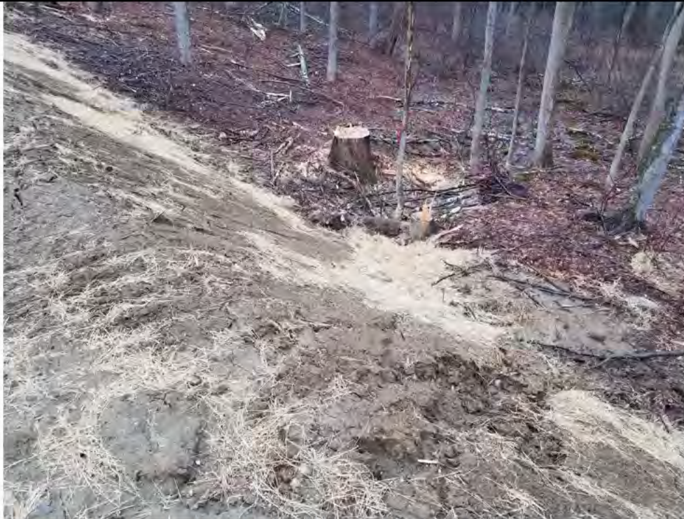
Photo 11: 3/31/2017, Litchfield: Map 29, Str83 abutting W-F4 and S-F2, E&S and pad armament required.
