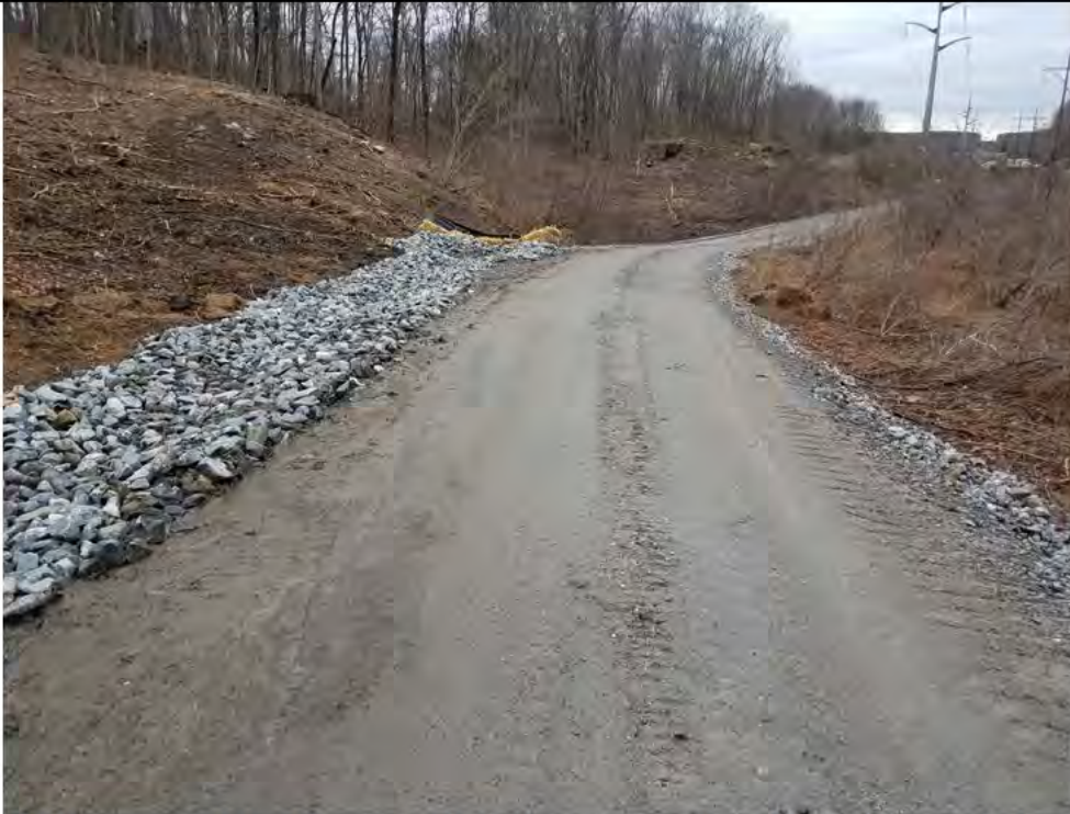
Photo 16: 04/07/2017, Thomaston: Map25, rock swale to temporary sediment basin/trap for surface water diversion.
