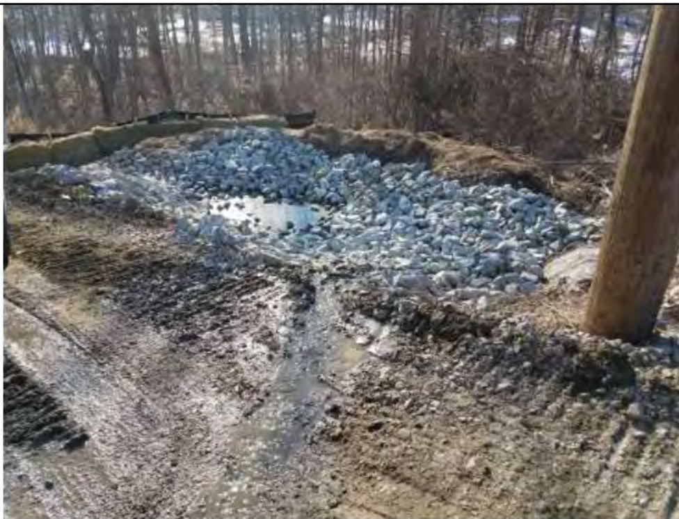
Photo 16: 2/23/2017, Litchfield, Map 26: Water bar and plunge pool upland of W-E2, DVP-E2-1 and DVP-E2-2.
