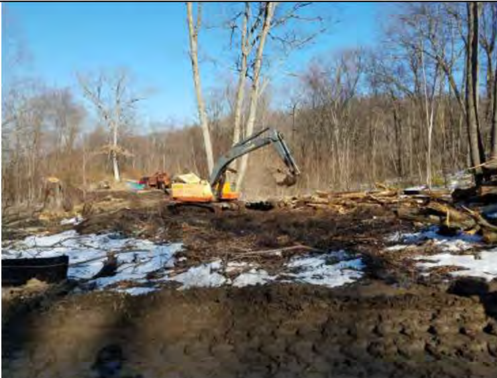
Photo 14: 2/23/2017, Watertown, Map 10: Non project related disturbance to W-C1/S-C1 by abutting landowner
