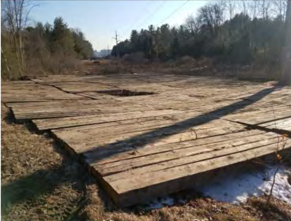
Photo 19: 2/23/2017, Harwinton, Map 35: Str95, matted pad, silt fencing still to be installed around exterior edge of mats to prevent turtle access per BMPs.
