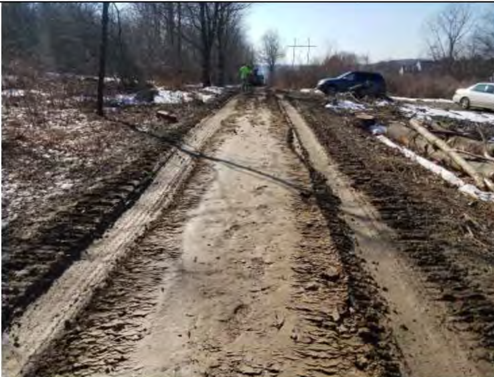
Photo 12: 2/23/2017, Watertown, Map 9A: Soft ground conditions, Northern grading road to remove rutting.
