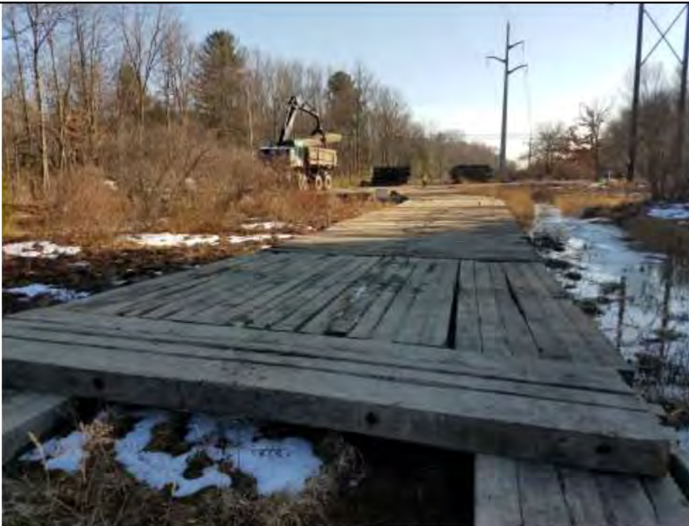
Photo 18: 2/23/2017, Litchfield, Map 28: Timber mat access road from Str78 to Str79 through W-E10, with 10'+/- animal crossing spaced every 36' along the approximate 500-foot run.
