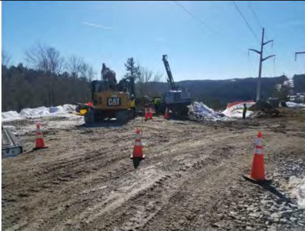
Photo 2: 2/17/2017, Harwinton, Map 32: Construction of temp structures north of Str88, drilling guide anchor holes.
