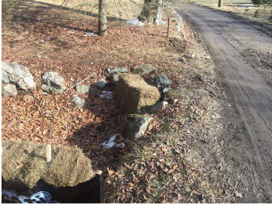
Photo #41: Thomaston- Morton Property, access road to Str58 and Str59, implementation of E&S controls
