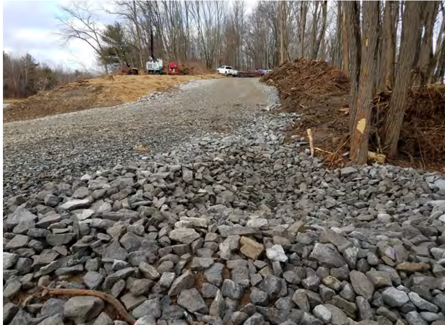
Photo #15:1/19/17, Litchfield: Access road to Str86, Str3236, Str3171, plunge pool at entrance/exit off Rt 8N
