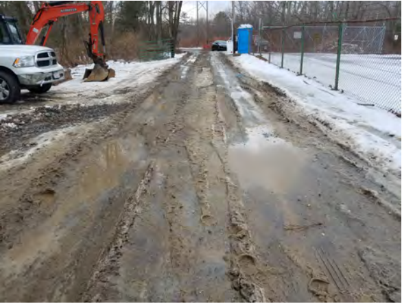
Photo #36:1/26/17, Harwinton- Campville Substation access road, petroleum release to ground
