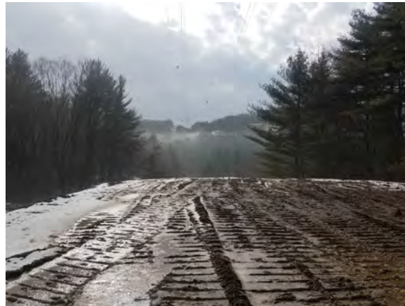
Photo #20:1/26/17, Harwinton- Str3235 and Str3174 pad construction, standing at Str3235 facing south toward Str86 in the far distance
