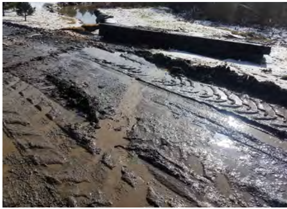
Photo #25:1/26/17, Thomaston- Robert K. & Jean R. Morton Property(41033, Map 21), access road to Str58-Str60, run off to Morton Pond
