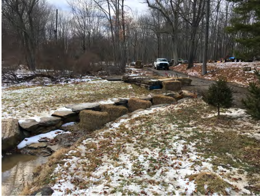
Photo #43: Thomaston- Morton Property, access road to Str58 and Str59, implementation of E&S controls
