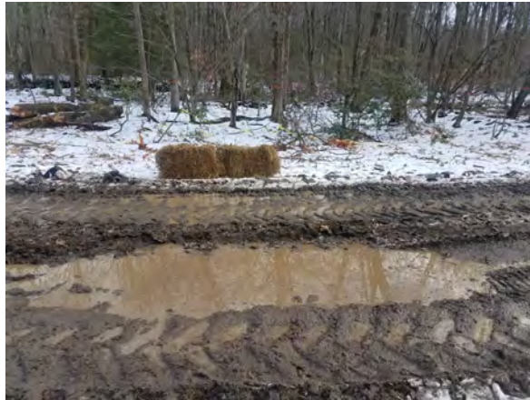
Photo #23:1/26/17, Thomaston- Additional hay bales to be added along the edge of the access road in the area of W-D4/VP D4-1 between Str53 and Str54
