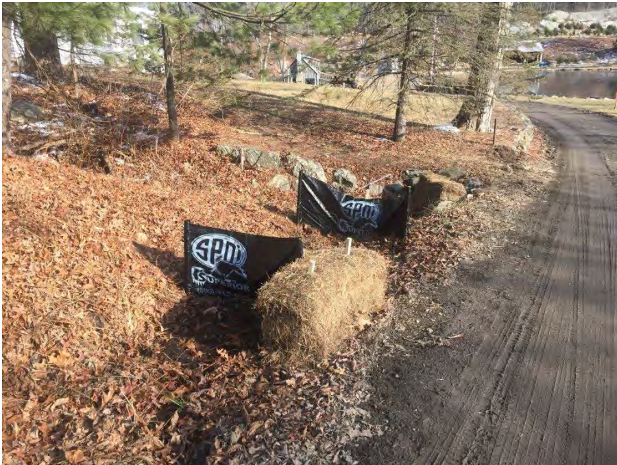
Photo #40: Thomaston- Morton Property, access road to Str58 and Str59, implementation of E&S controls
