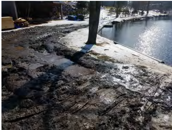
Photo #29:1/26/17, Thomaston- Robert K. & Jean R. Morton Property(41033, Map 21), access road to Str58-Str60, muddy conditions
