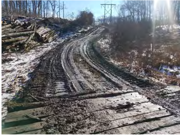
Photo #31:1/26/17, Watertown- Access road to Str24 through Str46, timber mats across W-C1 intermittent watercourse
