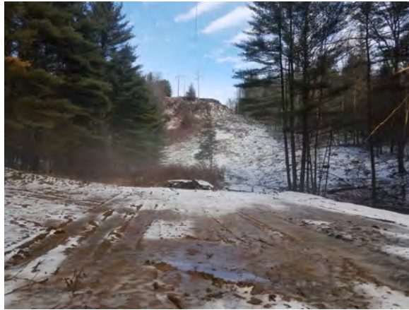
Photo #19:1/26/17, Harwinton- Clearing between Str87 and Str88 completed, standing at Pad Str87 facing north toward Str88 in the distance
