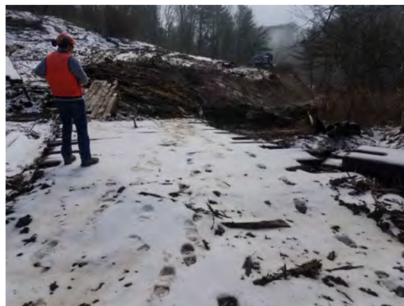
Photo #21:1/26/17, Harwinton- Timber mat crossing at the proposed culvert replacement (watercourse S-F11, Detail Sheet 10) moving approximately 10-feet to the east
