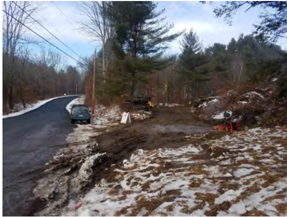
Photo #22:1/26/17, Harwinton- Access road to Str87 at Wildcat Hill Road, stone apron/tracking pad to be constructed
