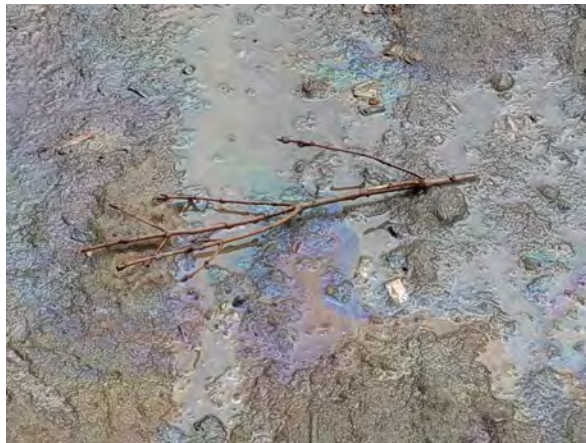
Photo #38:1/26/17, Harwinton- Campville Substation access road, petroleum release to ground
