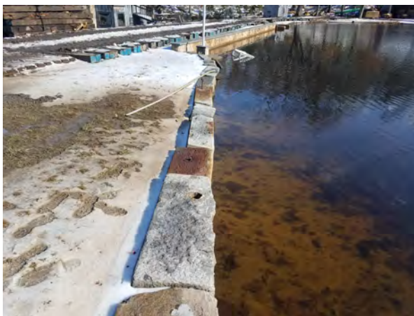
Photo #30:1/26/17, Thomaston- Robert K. & Jean R. Morton Property(41033, Map 21), access road to Str58-Str60, run off to Morton Pond
