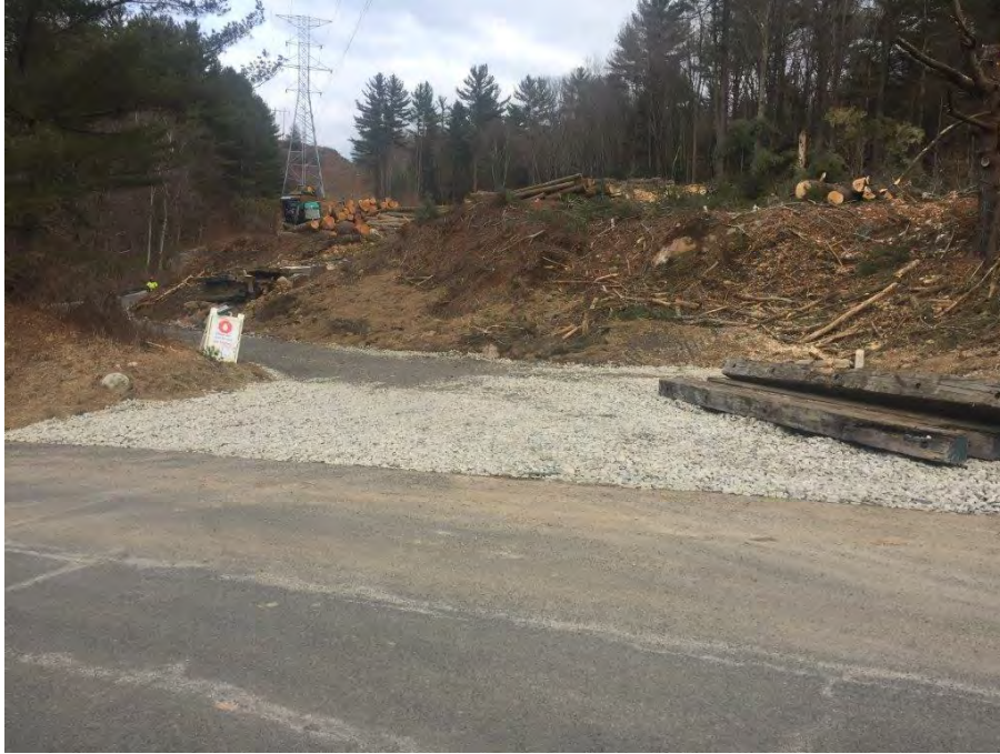
Photo #39: Harwinton- Stone apron/tracking pad added to access road at Str96 off Wildcat Hill Road
