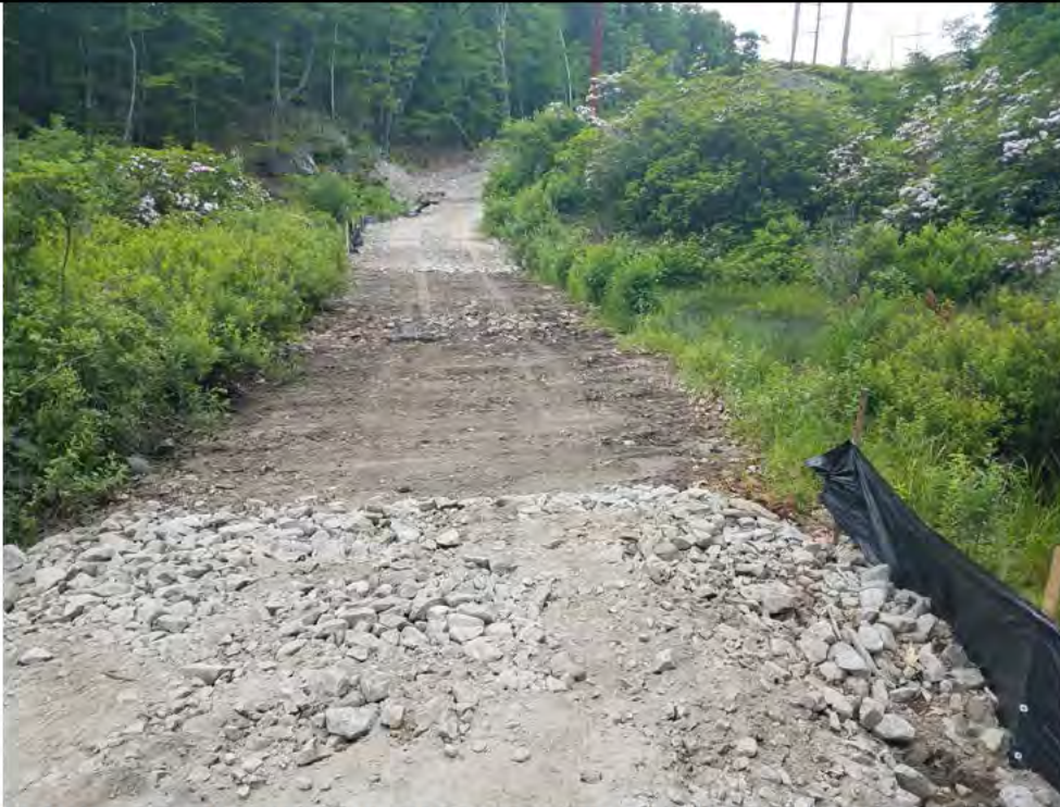
Photo 7: 06/15/2018, Watertown: Map 11, wetland/vernal pool W-C12/VP-C12-1, timber mat crossing removed, access road graded, and existing silt fence repaired. No visible impacts to wetland or vernal pool observed.
