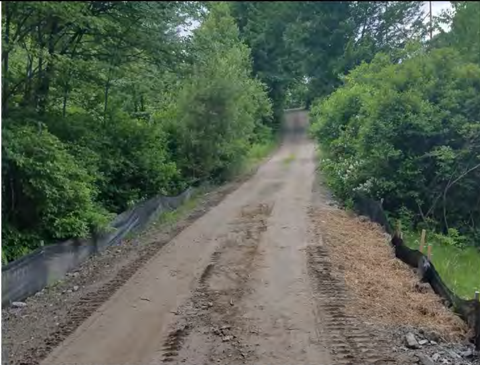
Photo 9: 06/15/2018, Watertown: Map 09A, access road to Str24-Str46 off of High Meadow Road, timber mats removed prior to last fall's winter shut down, silt fence repaired, hay mulch placed in disturbed ground area abutting wetland W-C2A.
