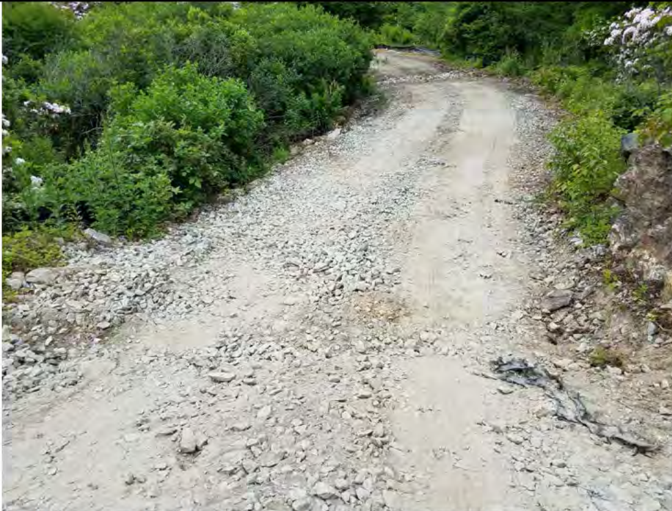
Photo 3: 06/15/2018, Watertown: Map 12, Wetland W-C15, stone access road graded, sections of silt fence removed (as instructed), full veg growth, area deemed stabilized, no soil movement around the area of the wetland. No visible impacts to the wetland.
