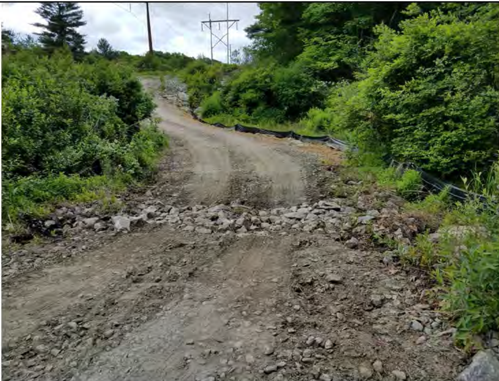
Photo 4: 06/15/2018, Watertown: Map 12, watercourse S-C15, timber mat crossing removed, stone hard bottom crossing improved, stone access road graded, and existing silt fence repaired.
