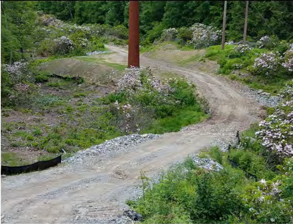
Photo 1: 06/15/2018, Watertown: Map 14, Wetland/Vernal Pool W-C20/VP-C20-1, timber mat crossing removed, stone access road graded, water bars & sediment traps cleaned out, and existing silt fence sections repaired.
