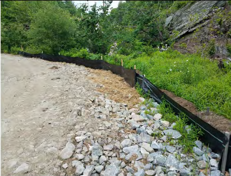
Photo 5: 06/15/2018, Watertown: Map 12, area of watercourse S-C4 and south end of W-C15, stone access road graded and improved, silt fence repaired and/or replaced, deteriorated hay bale/s appropriately distributed and utilized for stabilization of disturbed/exposed ground surface. No visible impacts to watercourse or wetland observed.
