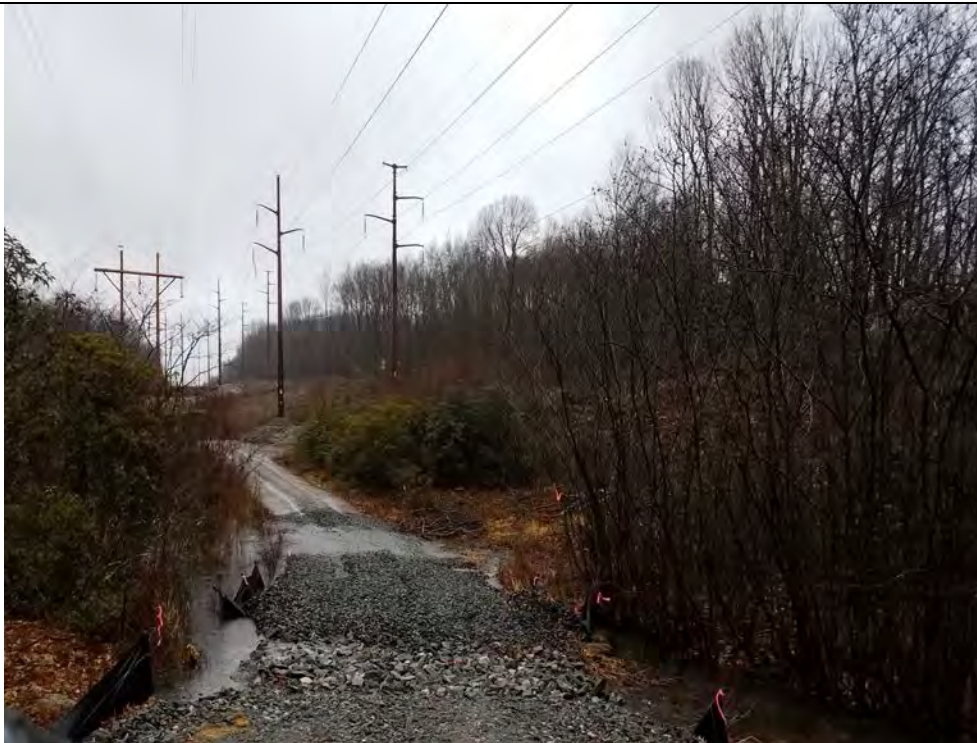
Photo 2: 03/02/2018, Thomaston: Map 25, S-E3 crossing between Str71 and Str72, Photo taken facing north towards Str72, water overflowing access road approximately 20-feet south of the constructed crossing.
