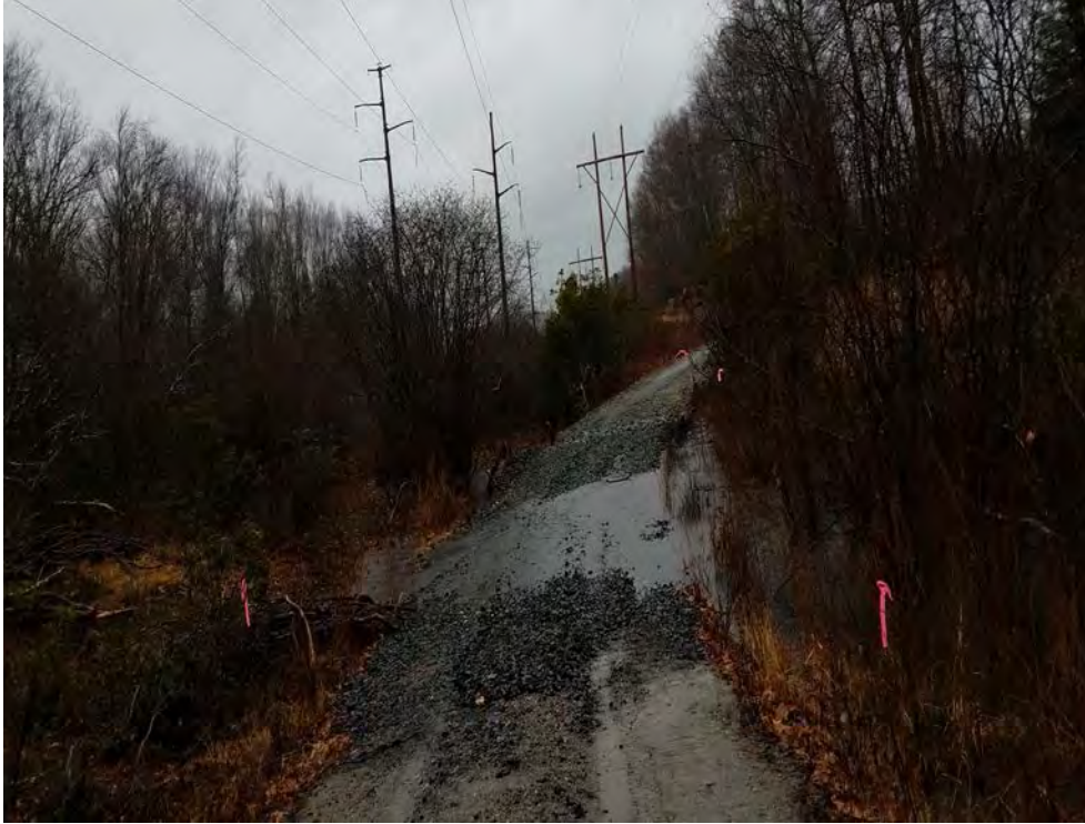
Photo 1: 03/02/2018, Thomaston: Map 25, S-E3 crossing between Str71 and Str72, Photo taken facing south towards Str71, Water overflowing access road approximately 20-feet north of the constructed crossing.
