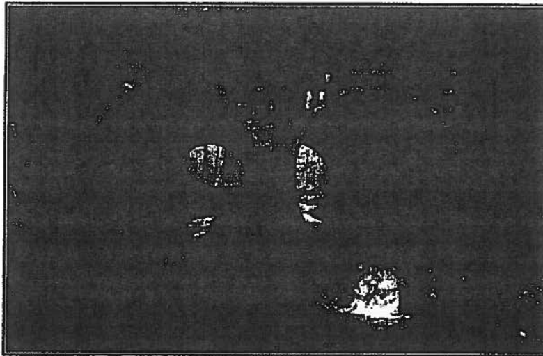
Figure 2. Example of culverts perched above streambed.
