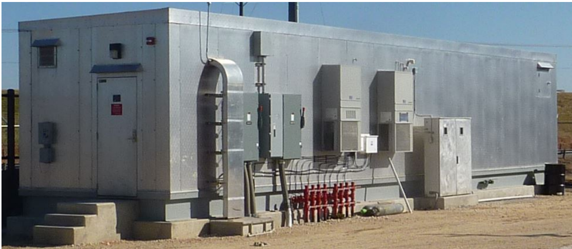
Figure H-10 Typical HPFF Pump House
