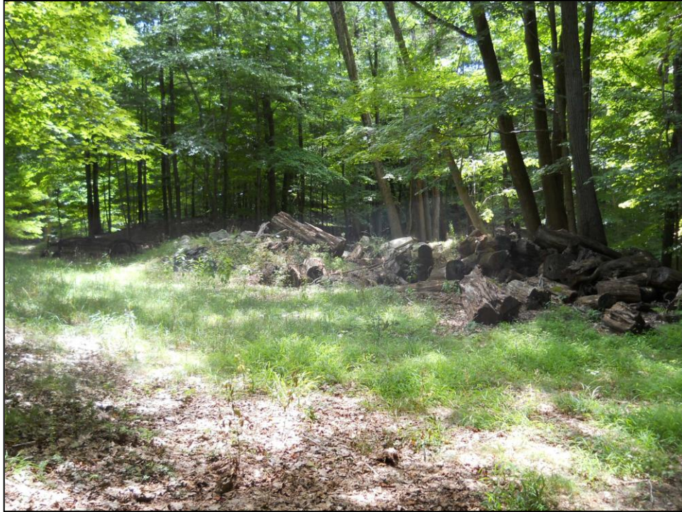
Overview photo of the proposed lease area associated with Alternate 2 facing southeast (Note push piles and debris).
