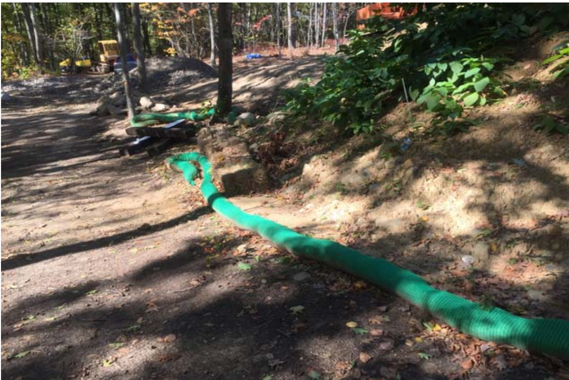
Photo 4: View of CA#11, remove accumulated sediment from compost filter sock at temporary soil stockpile, looking north.
